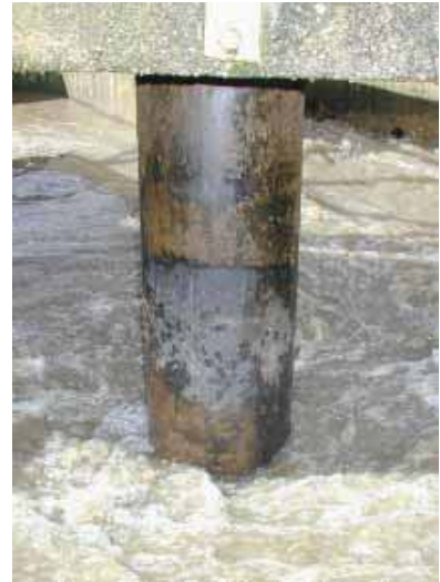
The effects of the continuous aeration can be clearly seen on the tank surface.
