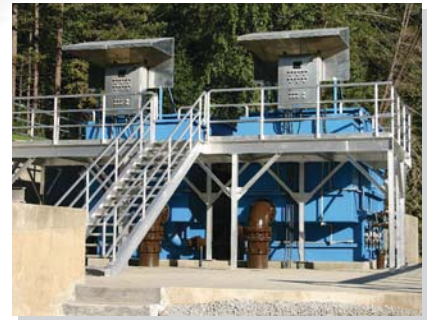
Two AquaDisk® Filters with walkway access.
