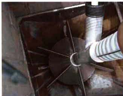
DynaSand Filter modules in concrete basin
