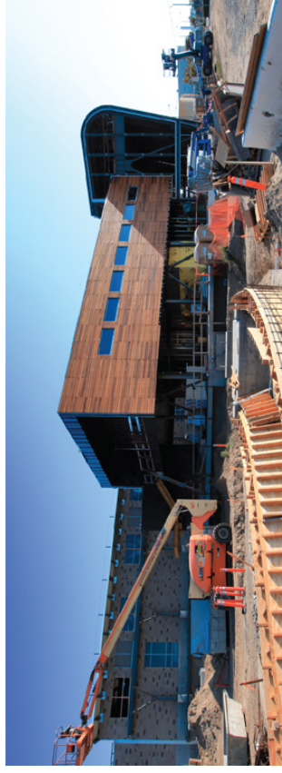
Advanced Water Purification Facility (AWPF)
