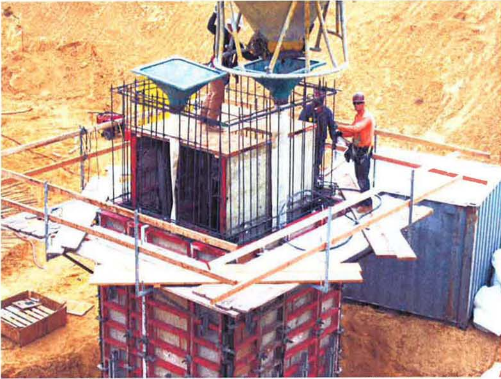
Pouring RAS/WAS Pump Station walls with funnels and tremies or "elephant trunks".
