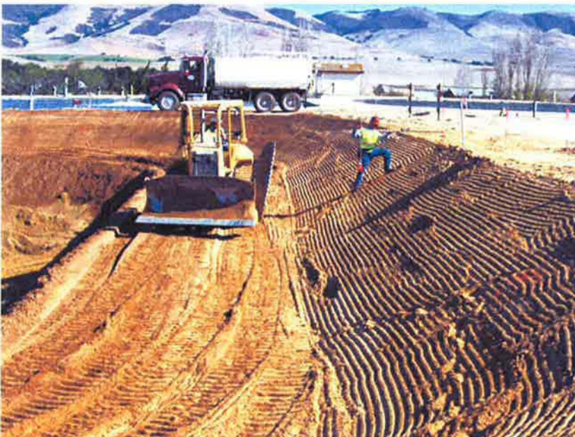
Cutting slopes at old Pond #1 to shape new slopes for Emergency Holding Basin.
