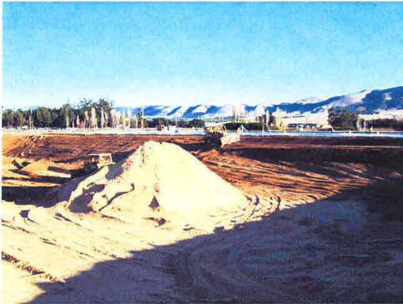
Gathering native material from existing Pond #1 slopes for forming new separation embankment.
