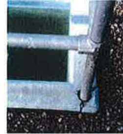
Figure 4. Cracking and spalling were observed around rail posts and tops of structure walls.
