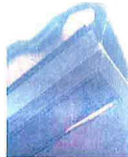
Figure 5. The Project Team will address building issues such as this roof damage that District staff is planning to repair in the near term.
