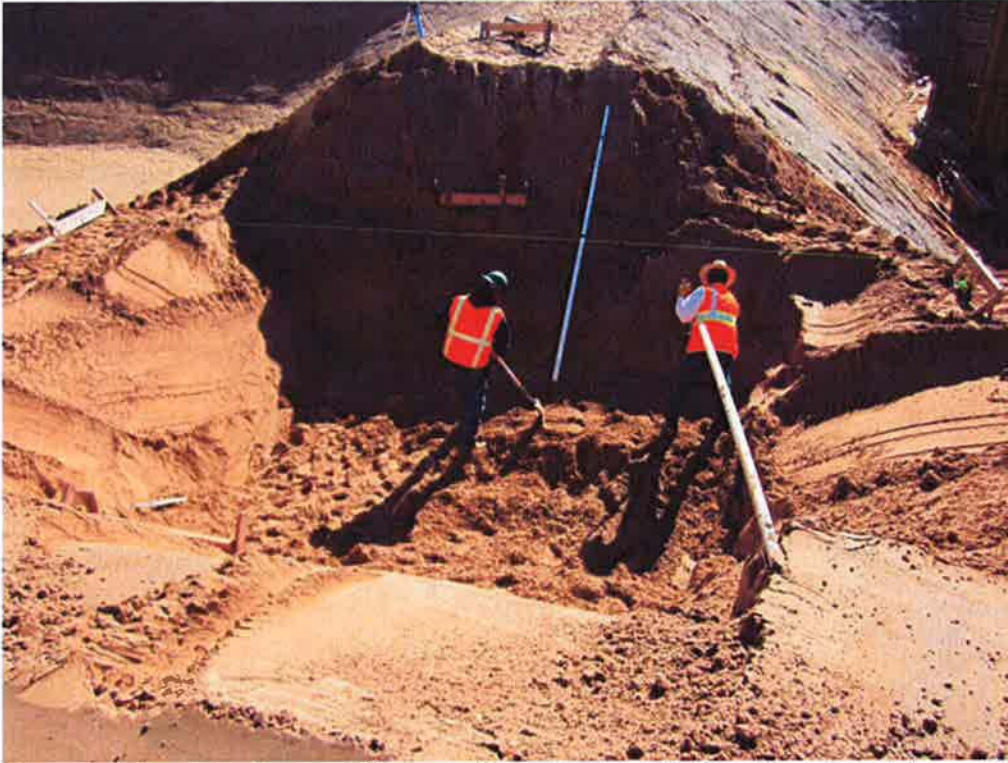
Completed excavation and fine grading of subgrade for effluent weir box at Emergency Basin.
