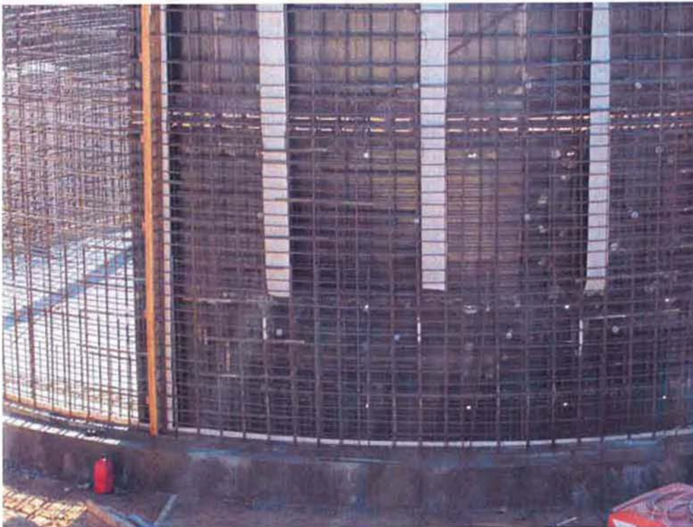
Tremmies installed to insure proper placement of concrete inside the wall and prevent separation of aggregate.
