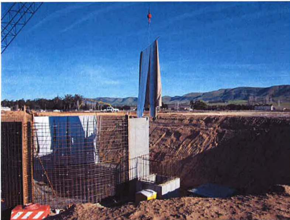
Wall forms removed and curing blankets in place and being installed on Clarifier #1.
