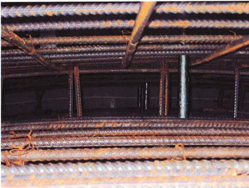
Looking down from top of forms through the rebar to the construction joint at the bottom of a wall.
