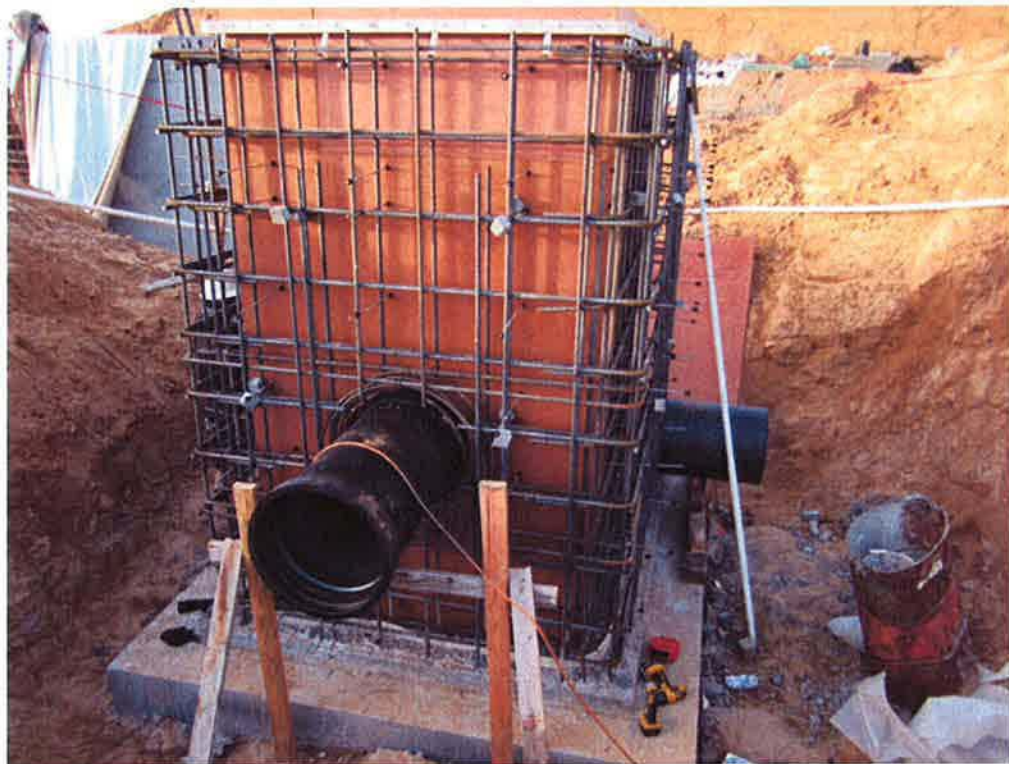
Wall forms, rebar and pipe penetrations installed for weir box at Emergency Basin.
