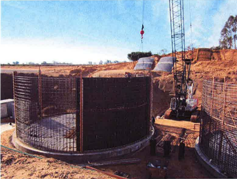
Lowering the second part of the inside form into place at Clarifier #1 for the first wall pour.
