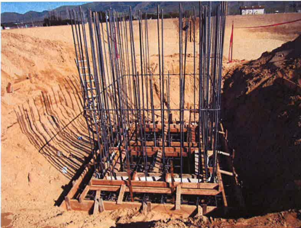
Forms and rebar installed for foundation of effluent weir box at Emergency Basin.
