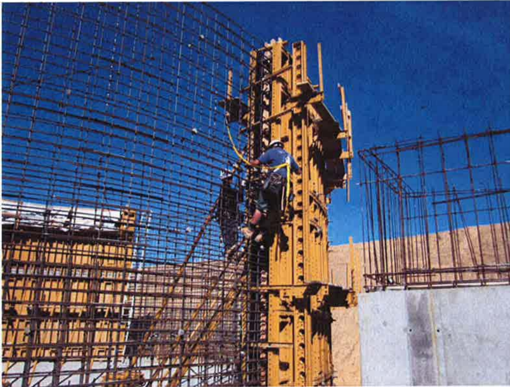
Securing the ends of wall forms at the construction joint at Clarifier #1.
