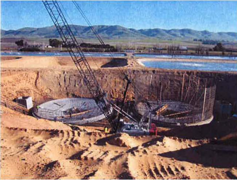
Foundations of clarifiers poured and cured, CMC Steel completing installation of rebar for walls.
