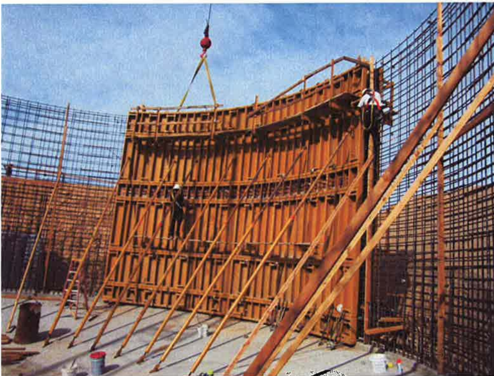
Finalizing adjustments to the forms and installing the walkway at the top at Clarifier #2.
