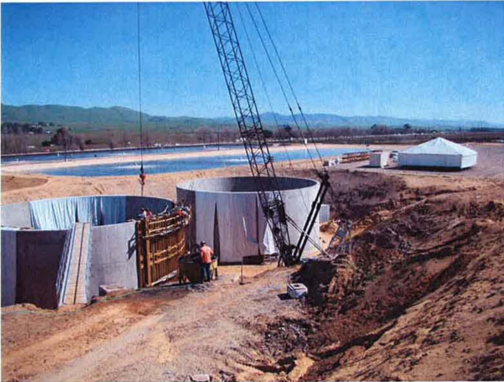
Pour completed at Clarifier #2 for the last wall section of the Clarifiers.
