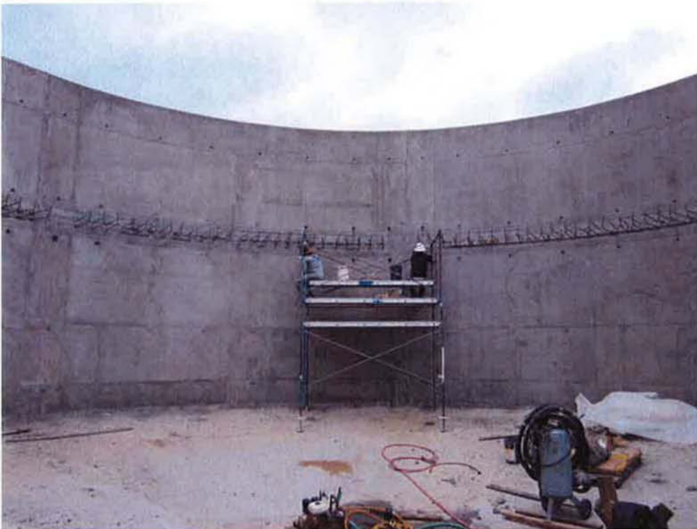
Cleaning up inside of clarifiers and patching form tie holes to prepare for sealant application.
