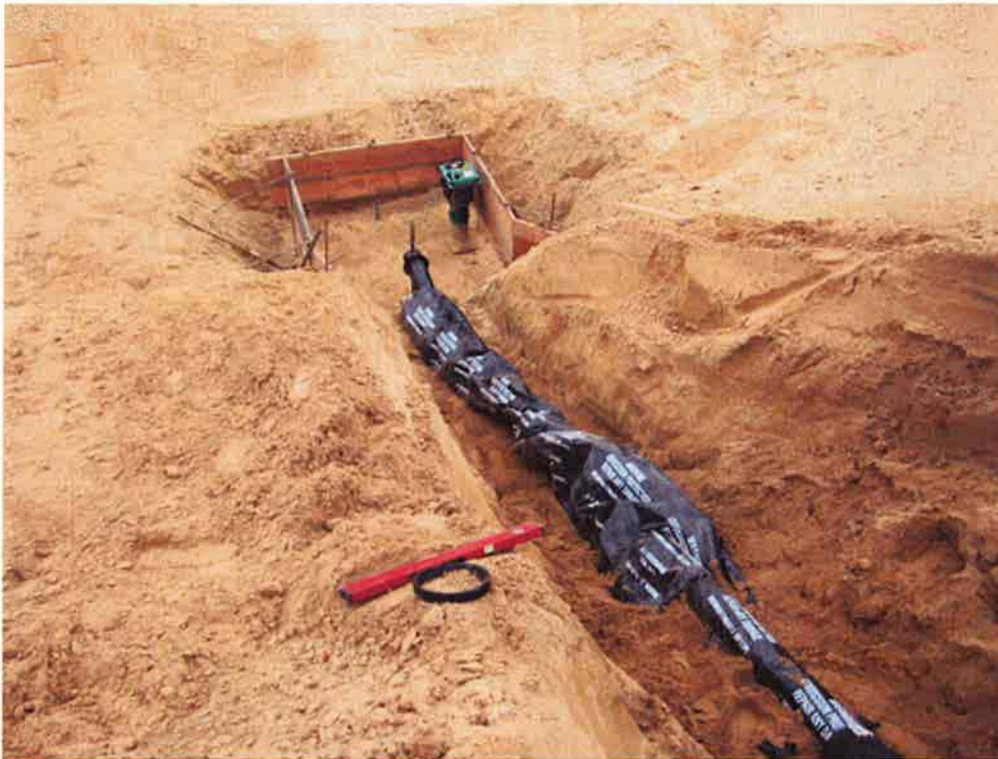
Installation of the 6" SD pipe and forming of the catch basin at the bottom of the Aeration Basin.
