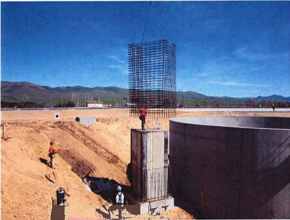
Lowering reinforcing steel into place over the inside forms of RAS/WAS Pump Station #2.
