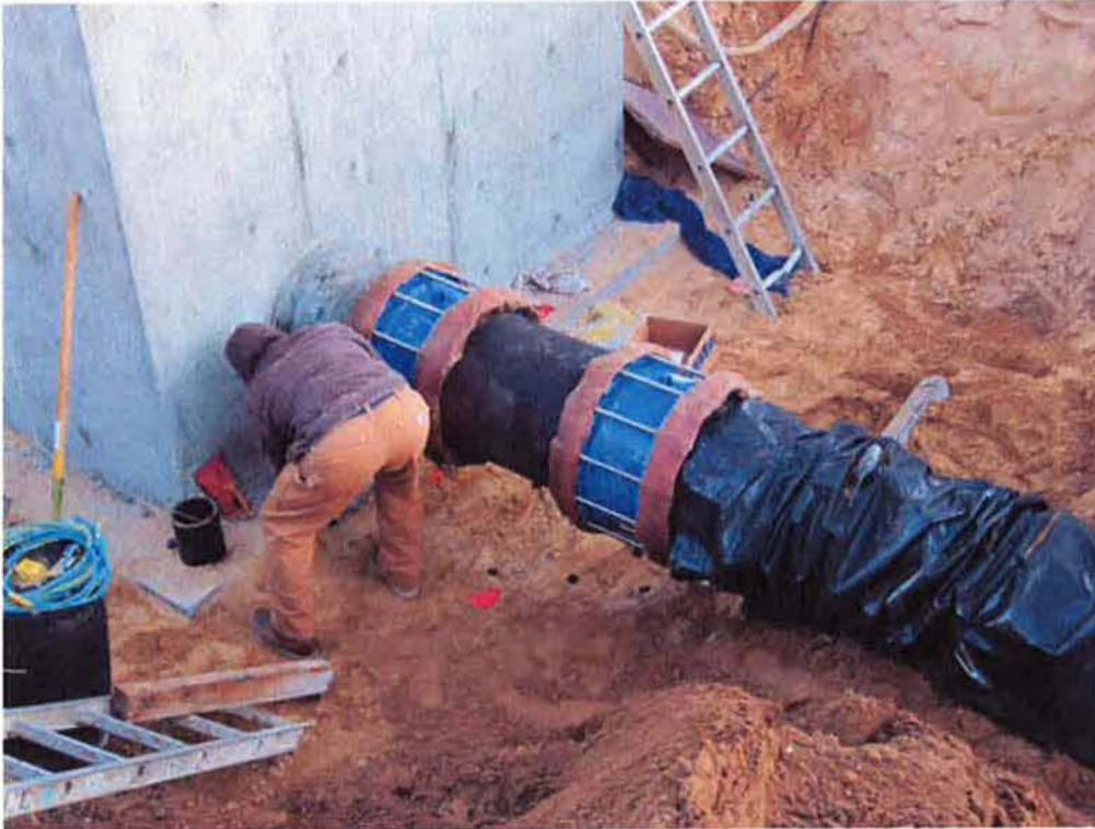
Couplings installed and wrapped with wax tape at the Aeration Basin weir box.
