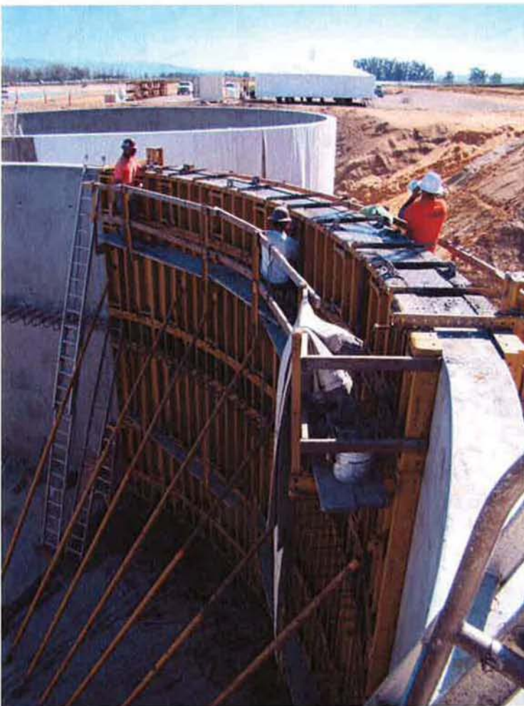
Finishing the top of the last wall section to be poured at Clarifier #2.
