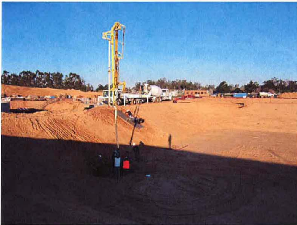
Pouring the effluent pipe concrete apron and the catch basin at the Emergency Holding Basin.
