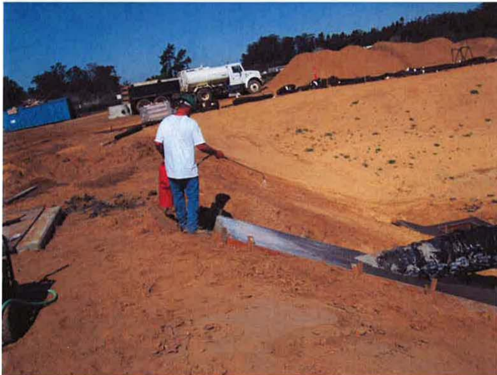
Applying curing compound to the concrete apron for the effluent pipe in the Aeration Basin.
