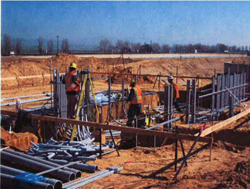
Conduit installation below the foundation on the MCC side of the Electrical/Blower Building.
