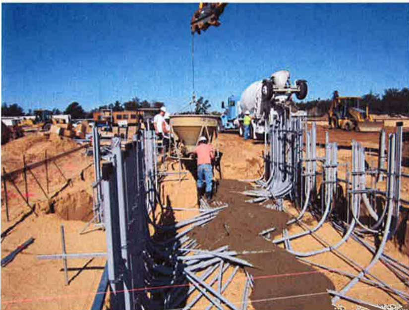
Pouring slurry for backfill around the conduits under the Electrical/Blower Building foundation.
