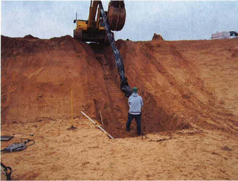
Installing the 6" SD pipe to the catch basin at bottom of the Aeration Basin.
