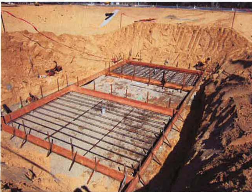
Installing forms and reinforcement for the foundations of the Air Vault and Meter Vaults.
