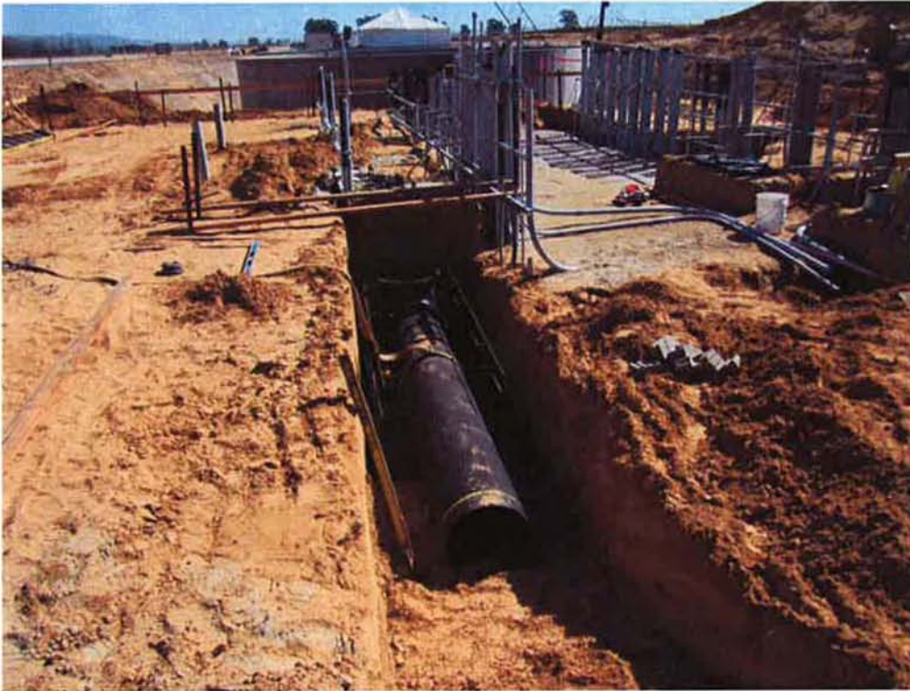
Installing the 18" AR piping from the Electrical/Blower Building to the Air Vault and Meter Vault.
