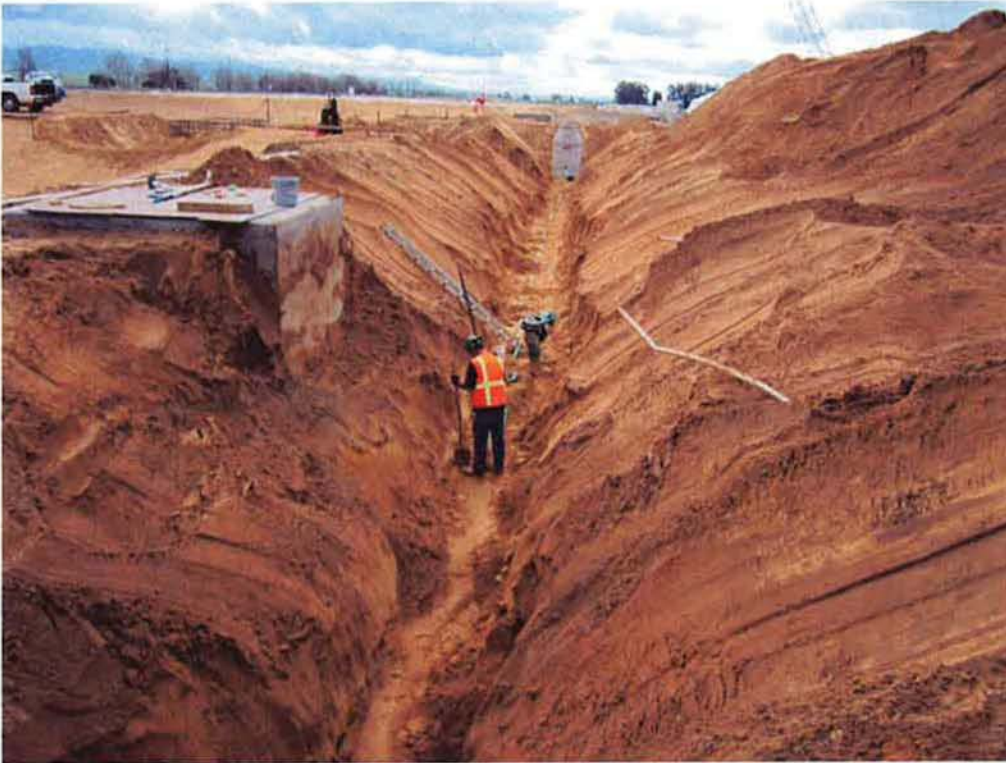
Backfilling and installing locator tape over 8" DR piping from Manhole #5 to Manhole #4.
