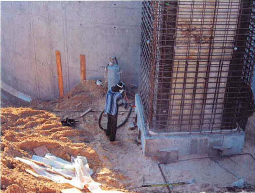
Sand blasting the top of the first wall pour of RAS/WAS Pump Station #2 to prepare for the second wall pour.
