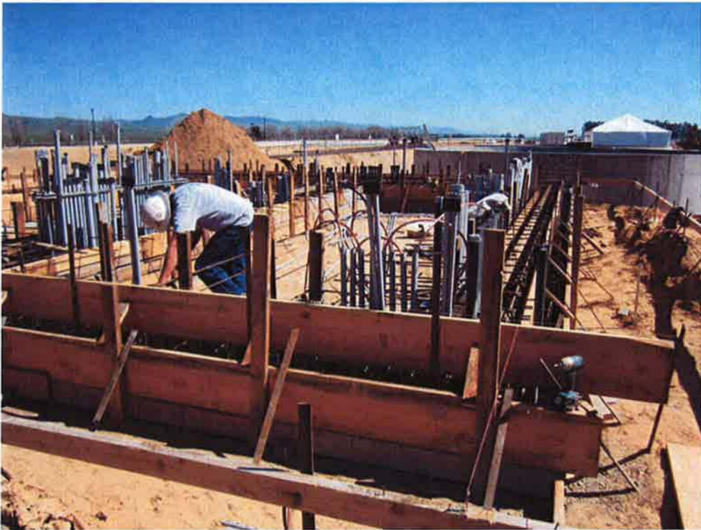
Bergelectric installing conduit and grounding cables through footing rebar and forms for Electrical/Blower Building.
