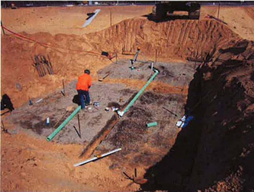
Installing drain pipes underneath the Air Vault and Meter Vaults for the piping to the Aeration Basin.
