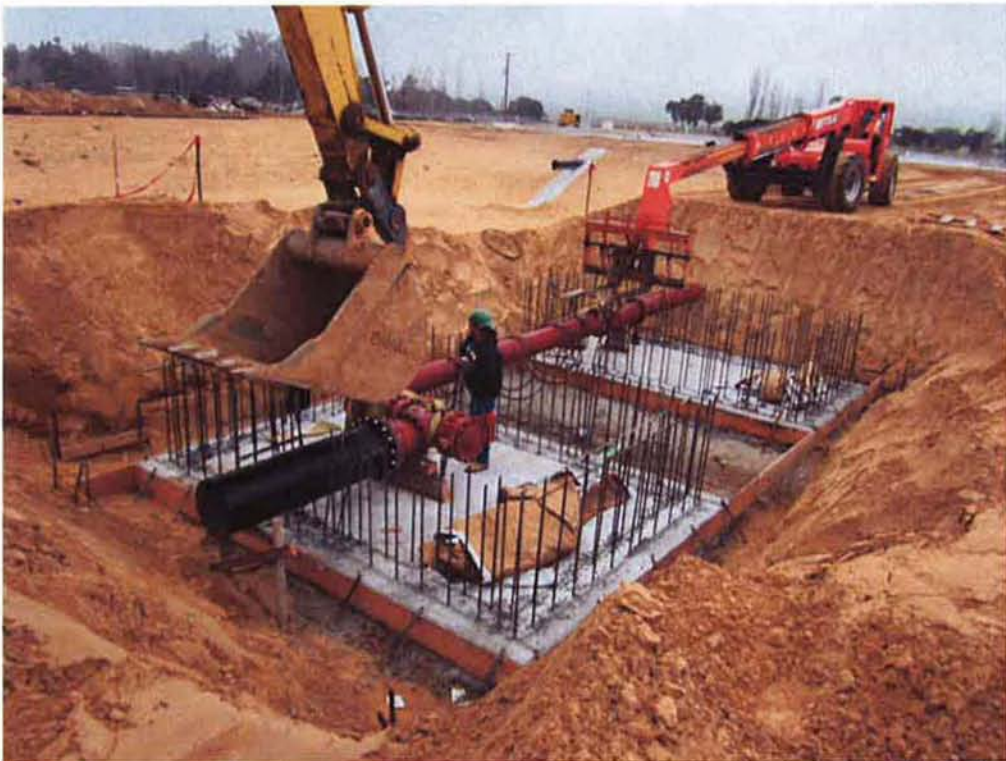
Installing the air piping through the Air Vault and Meter Vault for the Aeration Basin.
