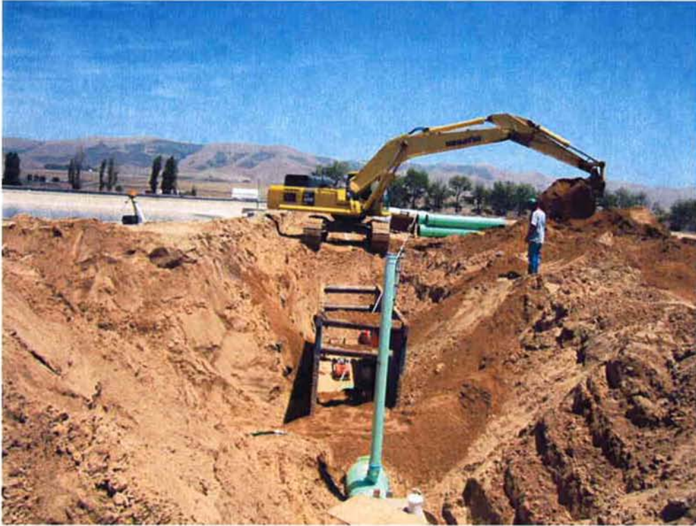
Cushman installing 24" SE2 pipe going east along the south end of Pond #4. Pipe riser is for pressure cleanout.
