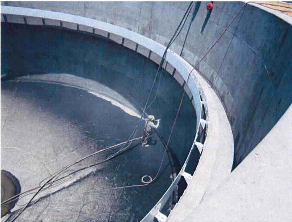
Subcontractor KNK Coating sandblasting the surface of Clarifier #2 in preparation for applying Xypex coating.
