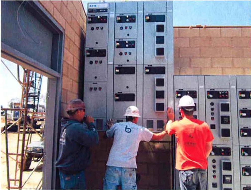
Cushman and Bergelectric setting electrical equipment on equipment pads before installing the roof.
