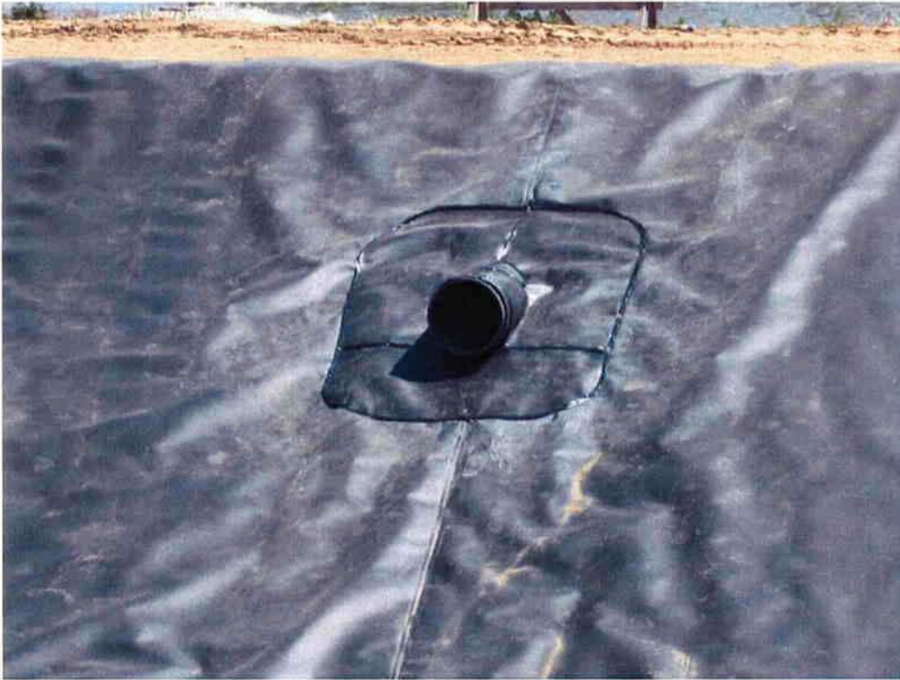
Final liner installation with extrusion weld around the pipe inlet of Aeration Basin #1.
