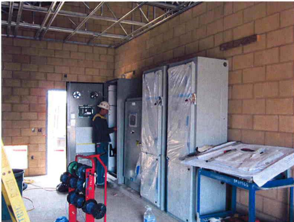
Instrument control panels and variable frequency drives installed.
