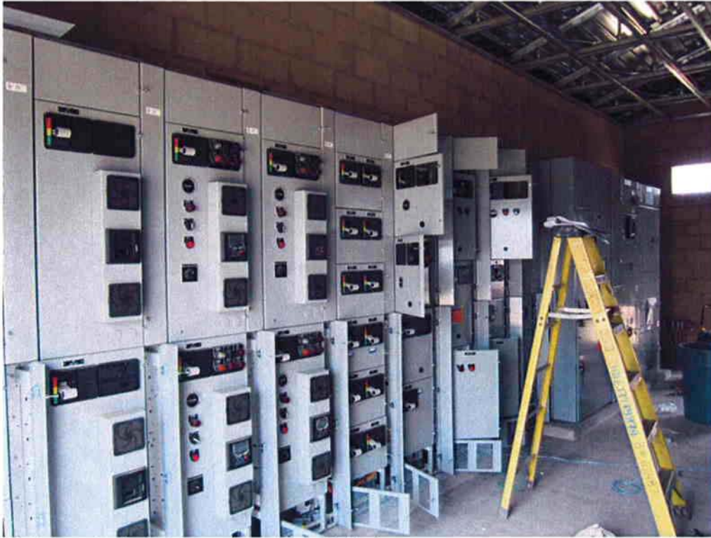
Motor control center equipment installed.
