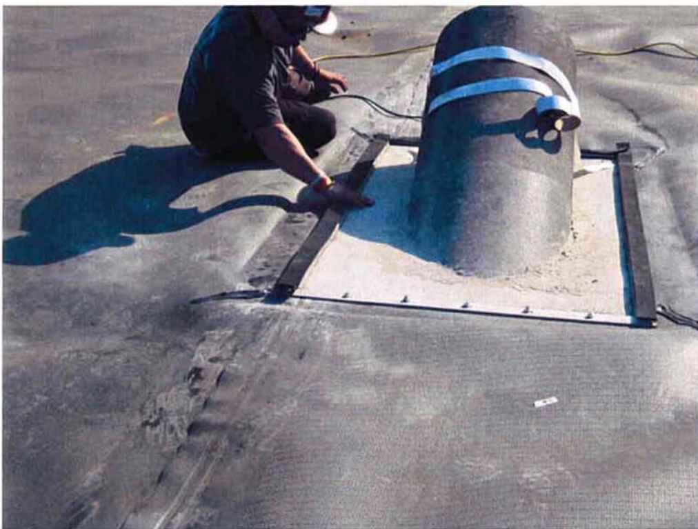
Installing the baton and boot at the inlet pipe penetration in Aeration Basin #1.
