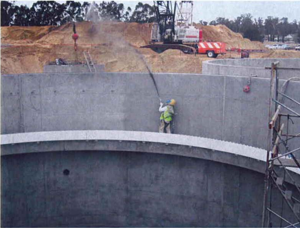
KNK Coating sandblasting the inside of Clarifier #1 in preparation for applying the Xypex coating.
