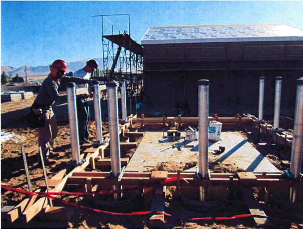
Cushman installing bollards around transformer pad in preparation for PG&E installing the transformer.
