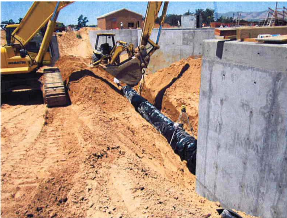
Cushman installing the 16" SE1 piping between the Process Water Pump Station and Clarifier #1.
