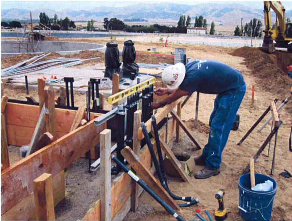
Bergelectric installing conduit through the footings of the Sodium Hypochlorite Storage building.
