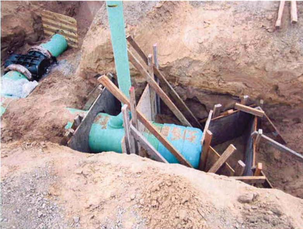
Forms for pouring thrust block at a tee on the 24" SE2 pipe.
