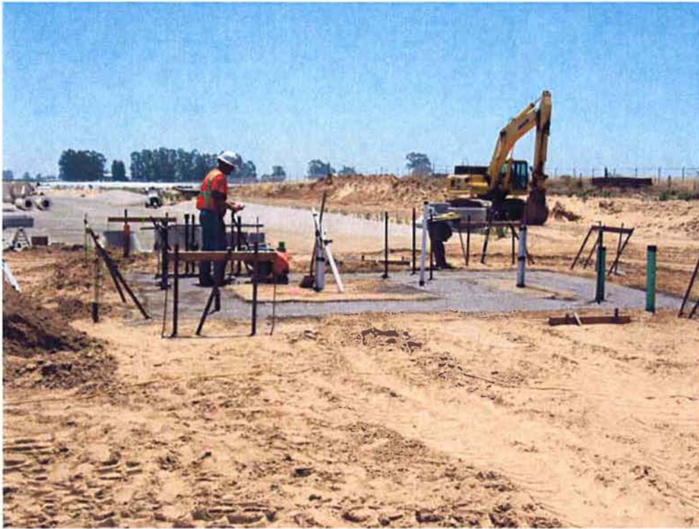
Compacting the base for the footings of the Sodium Hypochlorite Storage building.
