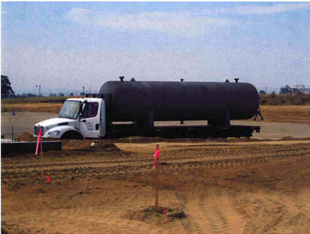
Receiving the hydropneumatic tank.
