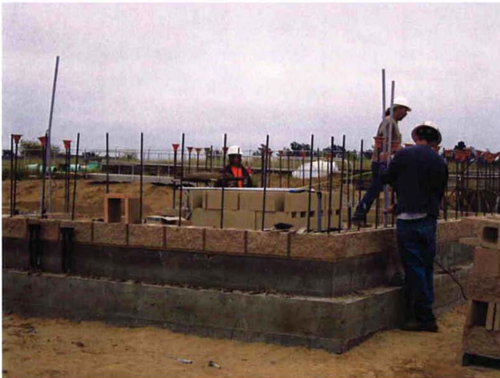
Beinscroth Masonry placing first course of block at the Sodium Hypochlorite Building and Bergelectric installing conduit running through the walls.
