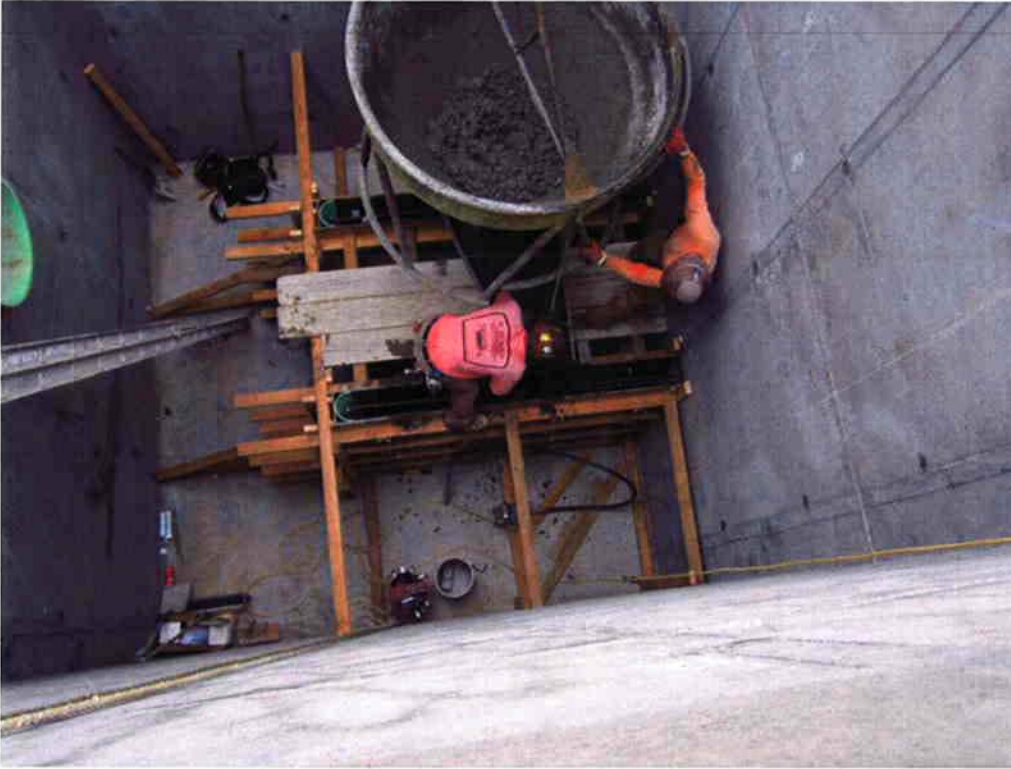
Pouring the dividing walls for the prerotation basins in the Influent Pump Station.
