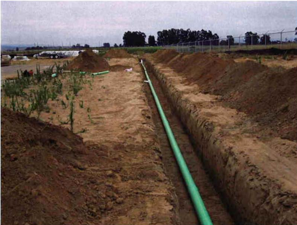
Cushman installing the 6-inch DR piping to the west of the Sludge Drying Beds.
