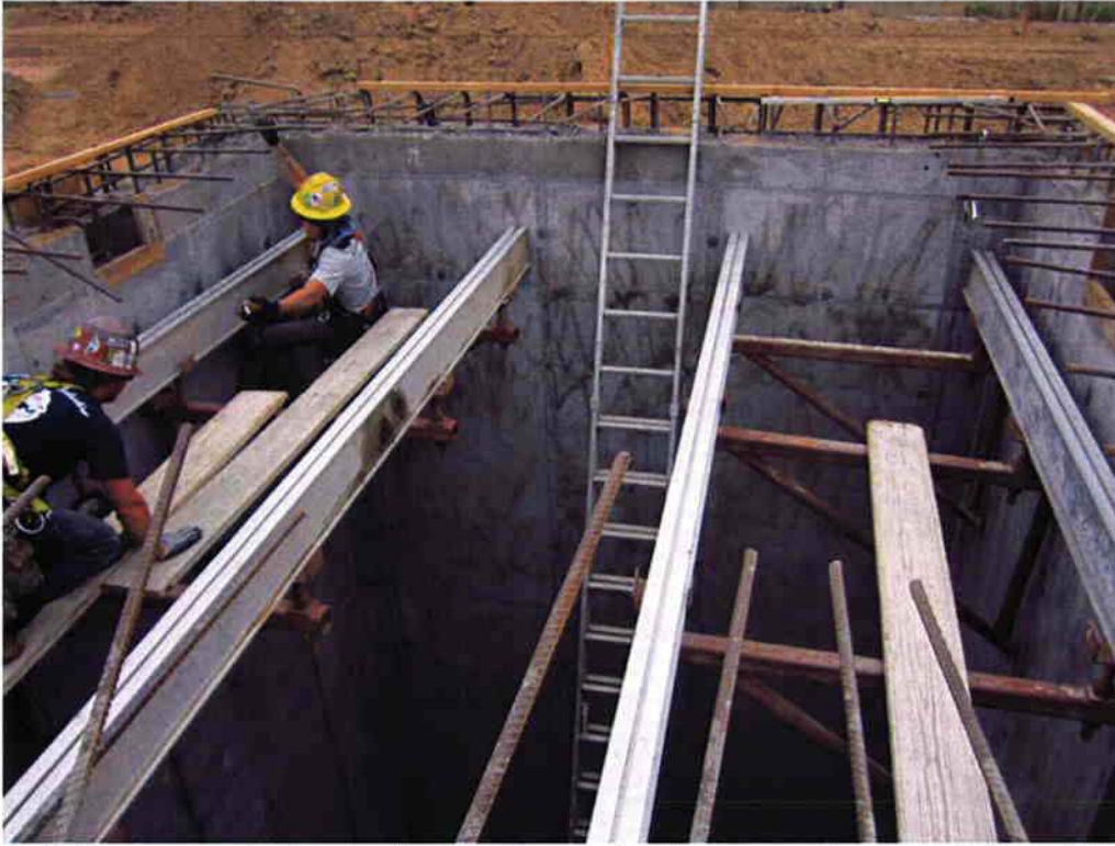
Installing supports for shoring to prepare for deck pour at Influent Pump Station.
