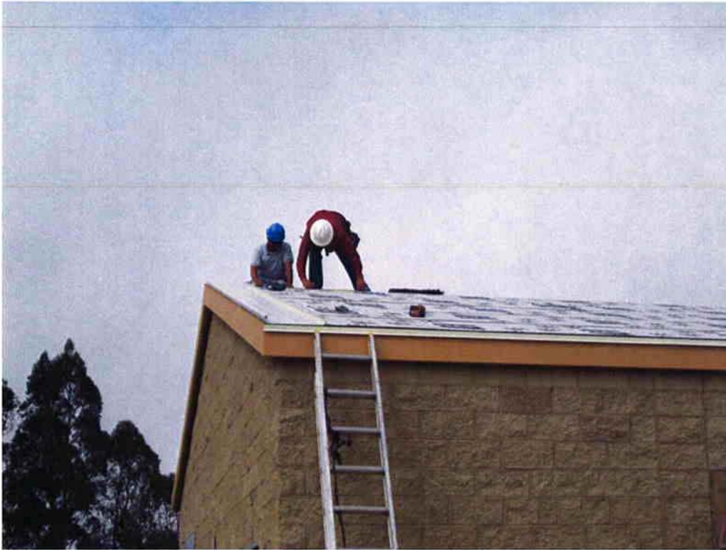
Dueck Roofing installing the standing metal roof on the Sodium Hypochlorite Building.
