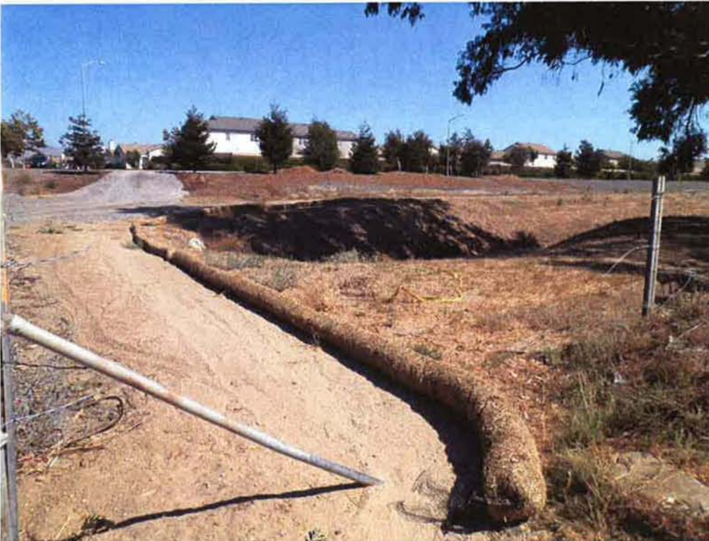
Straw waddles installed for SWPPP around the SBCFC drainage channel near the temporary access ARB constructed on the south side of the levee.
