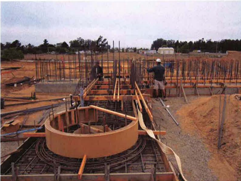
Cushman forming the slab and grit vortex of the Grit Removal System.
