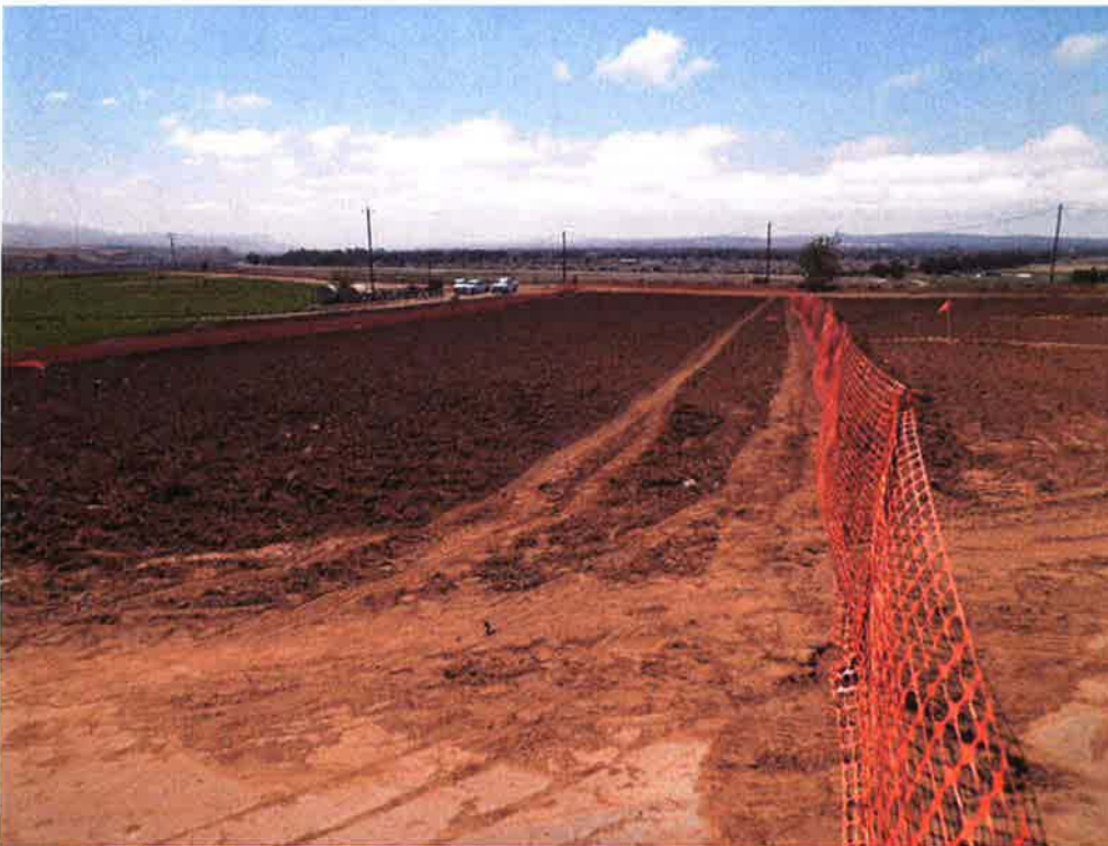
ARB installing temporary orange snow fence on boundaries of temporary construction easement to protect HDD tracing wires during drilling.
