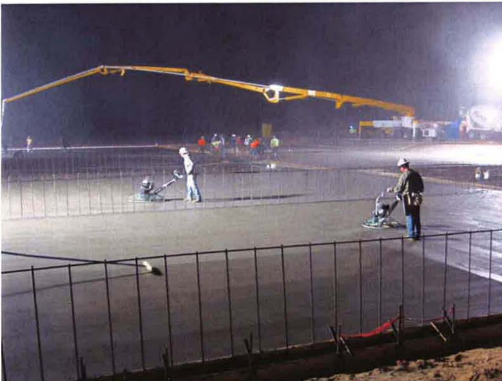
Cushman starting finish work on concrete slabs at Sludge Drying Beds during first night pour.
