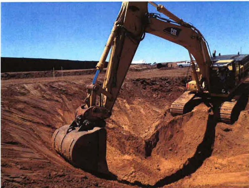
Excavation for the 54-inch diameter casing at the north side of the project.
