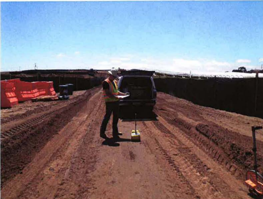
Fugro taking compaction tests for the base under the temporary access road.
