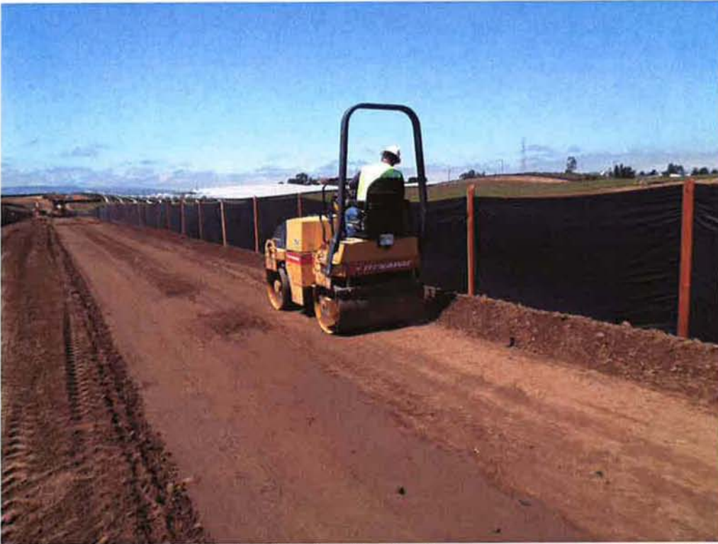
ARB's subcontractor Burke Construction building temporary access road to the pump station site on the north side of the project.
