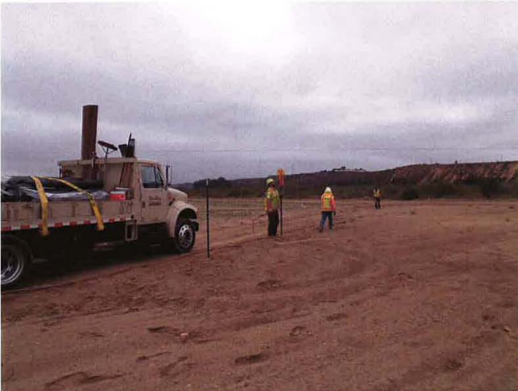
Marborg installing fence posts for 6' silt fence on south side of project.
