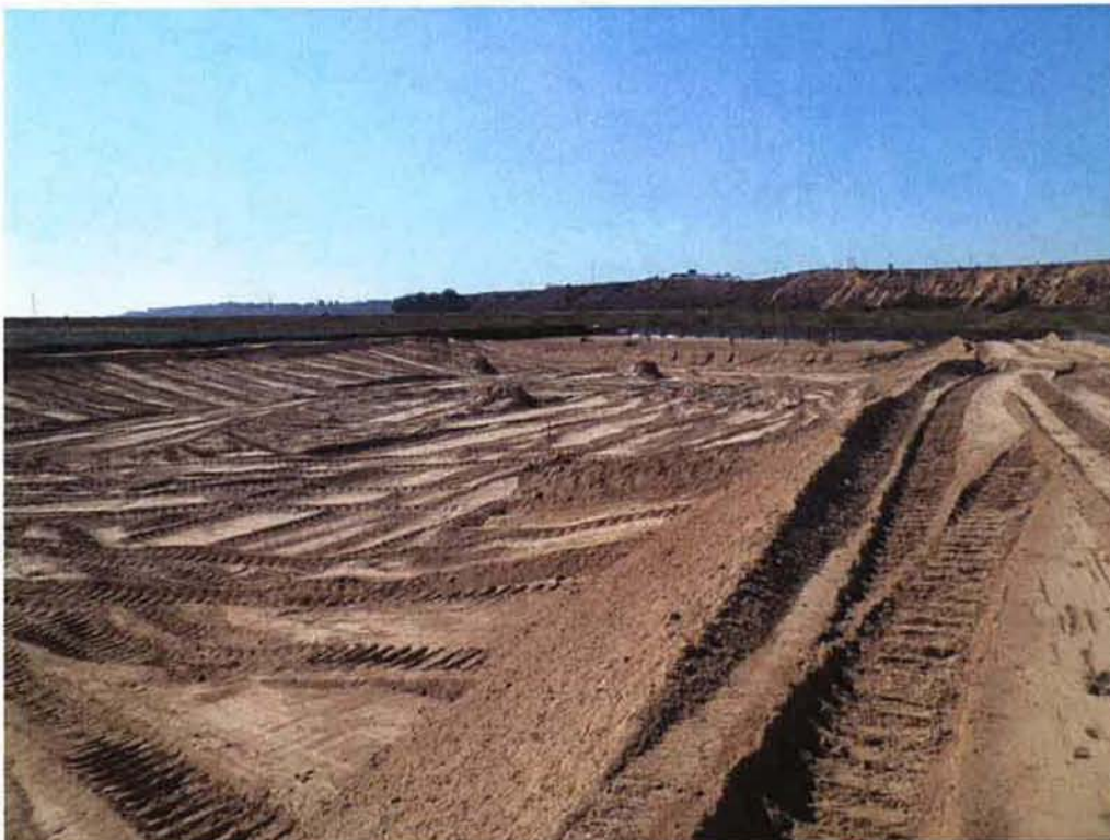
Excavation and preservation of top soil on the south side within the temporary construction easements.
