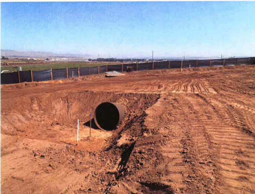
Completed installation of 54-inch diameter casing on north side of the project.
