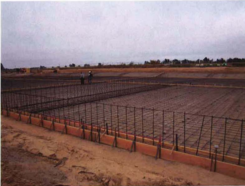
Cushman setting screed guide rails at Drying Bed #1 in preparation for first concrete pour.
