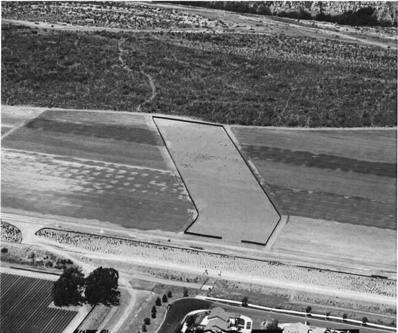
Aerial photo of the south side with silt fence installed at temporary construction easements.
