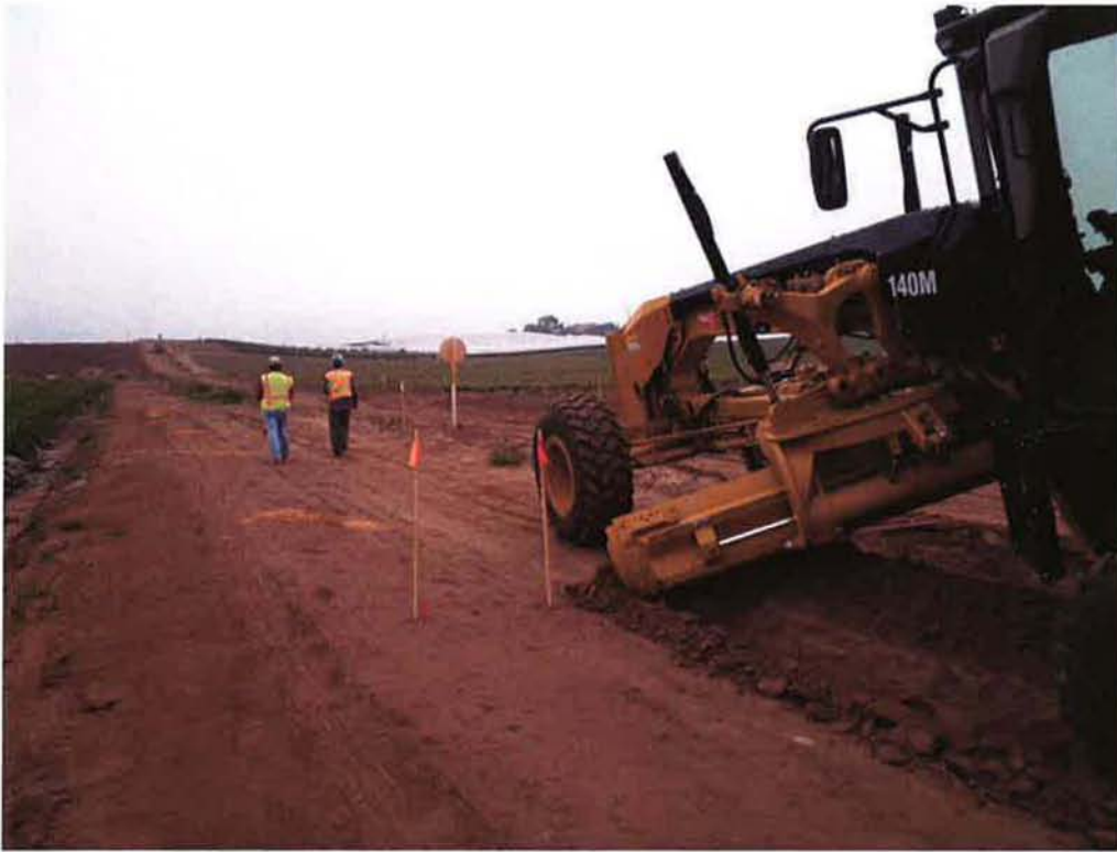
Burke and ARB creating a 12" deep ditch to key in the silt fence on the north side to prevent migration of California Red Legged Frogs onto the site.
