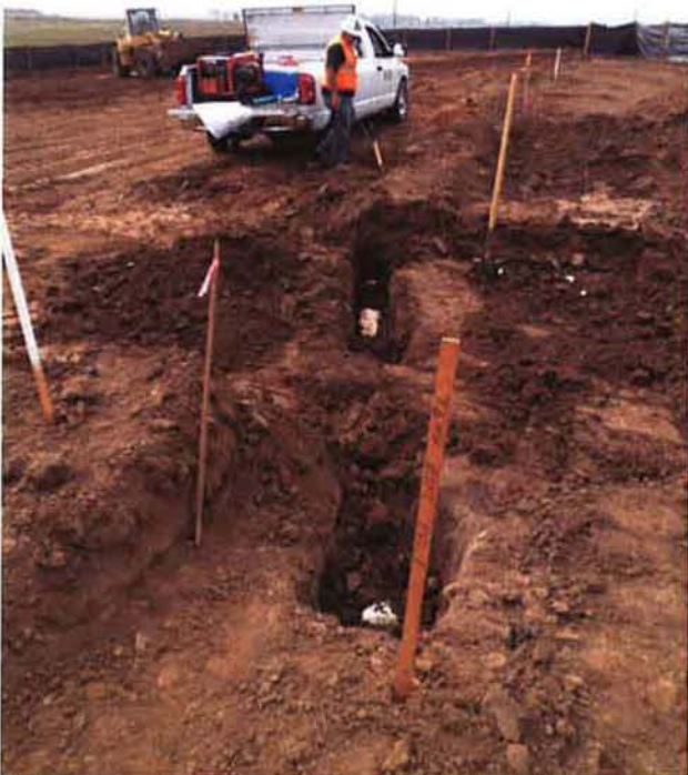
ARB potholing for existing irrigation lines crossing the future pump station site and HDD work area.
