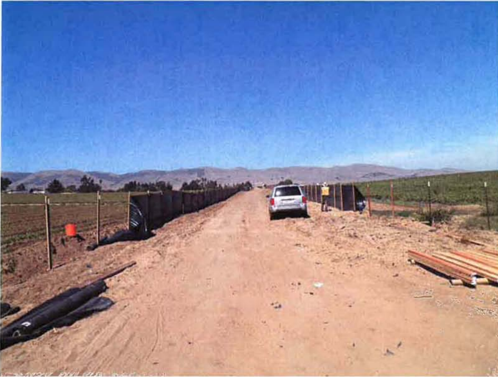
Silt fence installed along access road to the pump station site. Rincon on site to provide monitoring for CRLF's.
