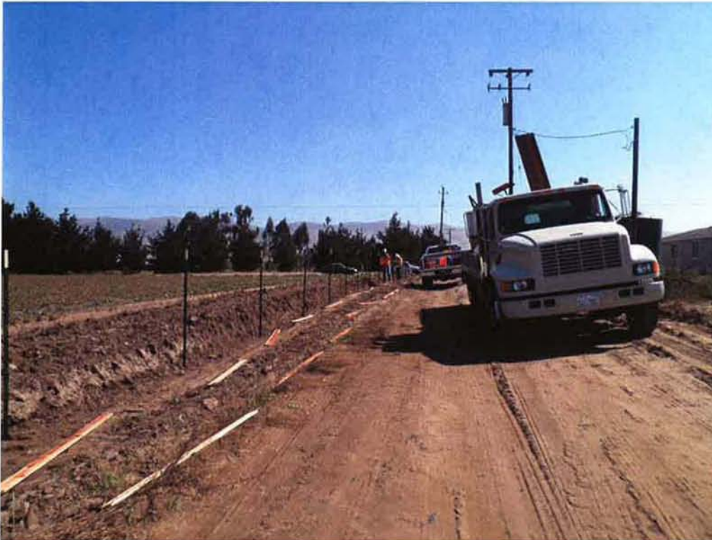
Marborg and ARB installing tee posts for the silt fence along the access road to the pump station site on the north side.
