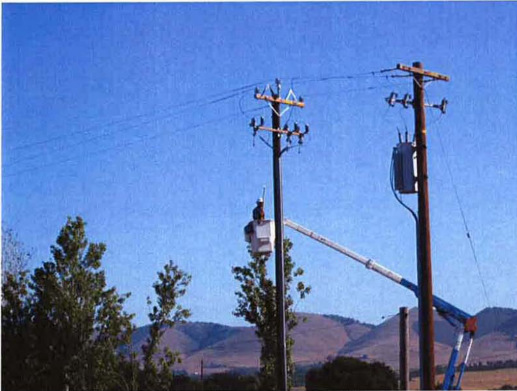
PG&E energizing the new service on August 15, 2013.
