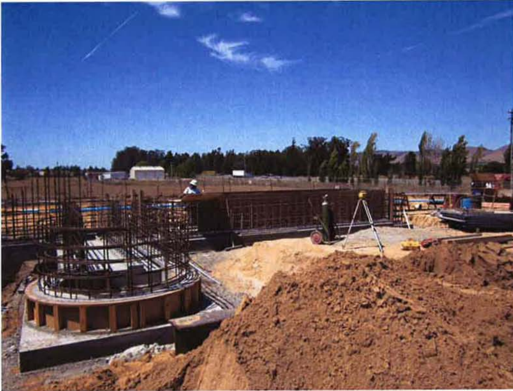
Forming walls of the grit vortex and the interior walls of the Headworks Screening System.
