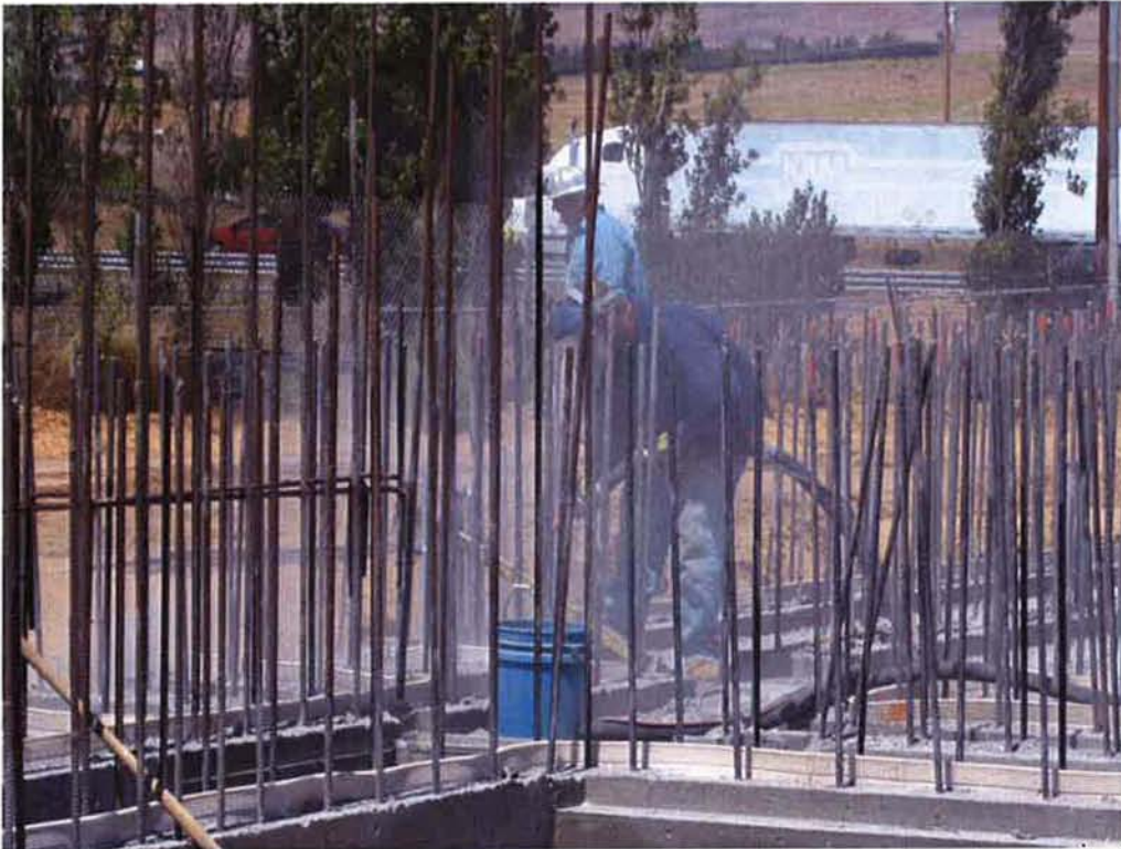
Cushman sand blasting base of starter walls in preparation for forming interior walls of the Headworks Screening System.
