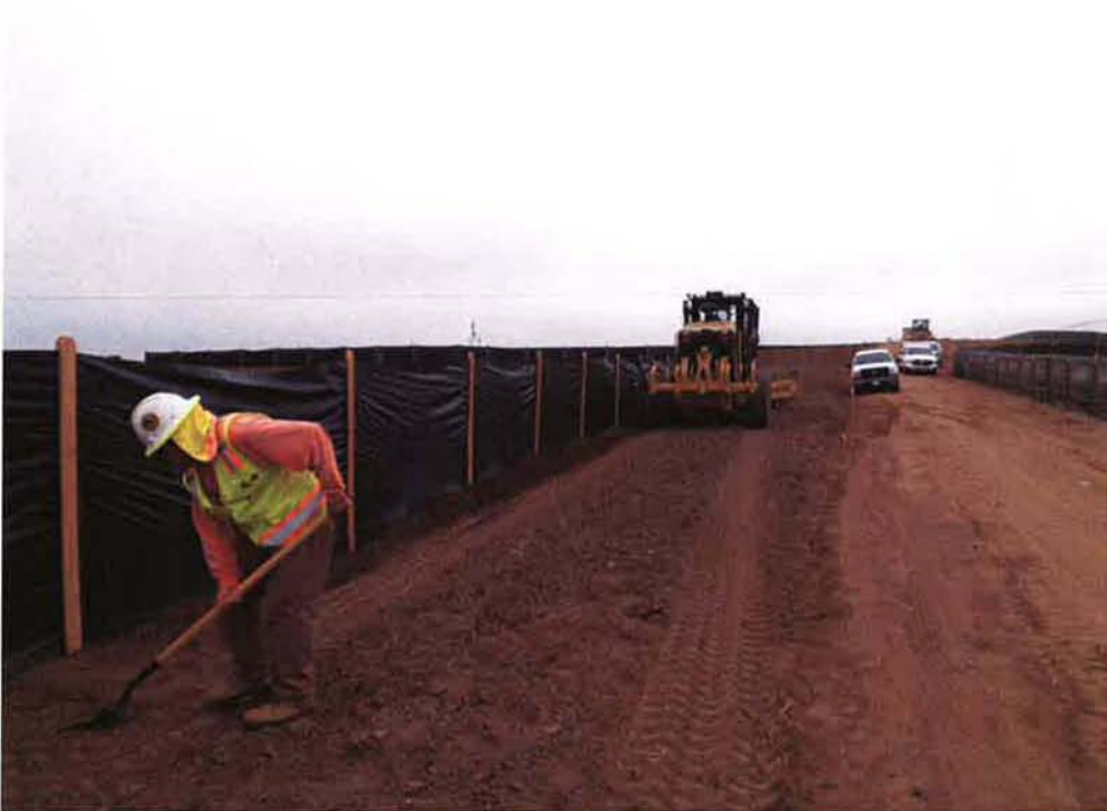
Burke using grader and ARB working by hand to key in the bottom of the silt fence along the access road to prevent CRLF's from migrating onto the site during construction.
