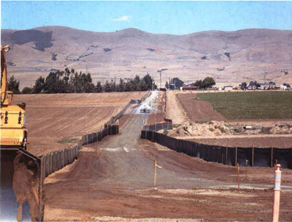
View from future pump station site of temporary access road and silt fence installed.
