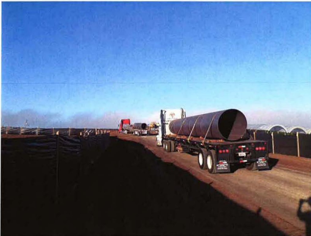
Casing (54-inch diameter) arriving on the north side at the future pump station site.
