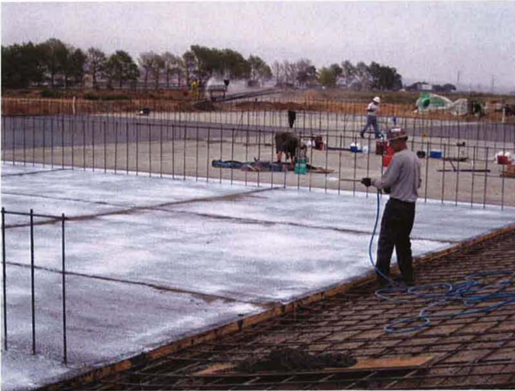
Cushman spraying curing compound on last slab section of Sludge Drying Bed #2 after last concrete pour.
