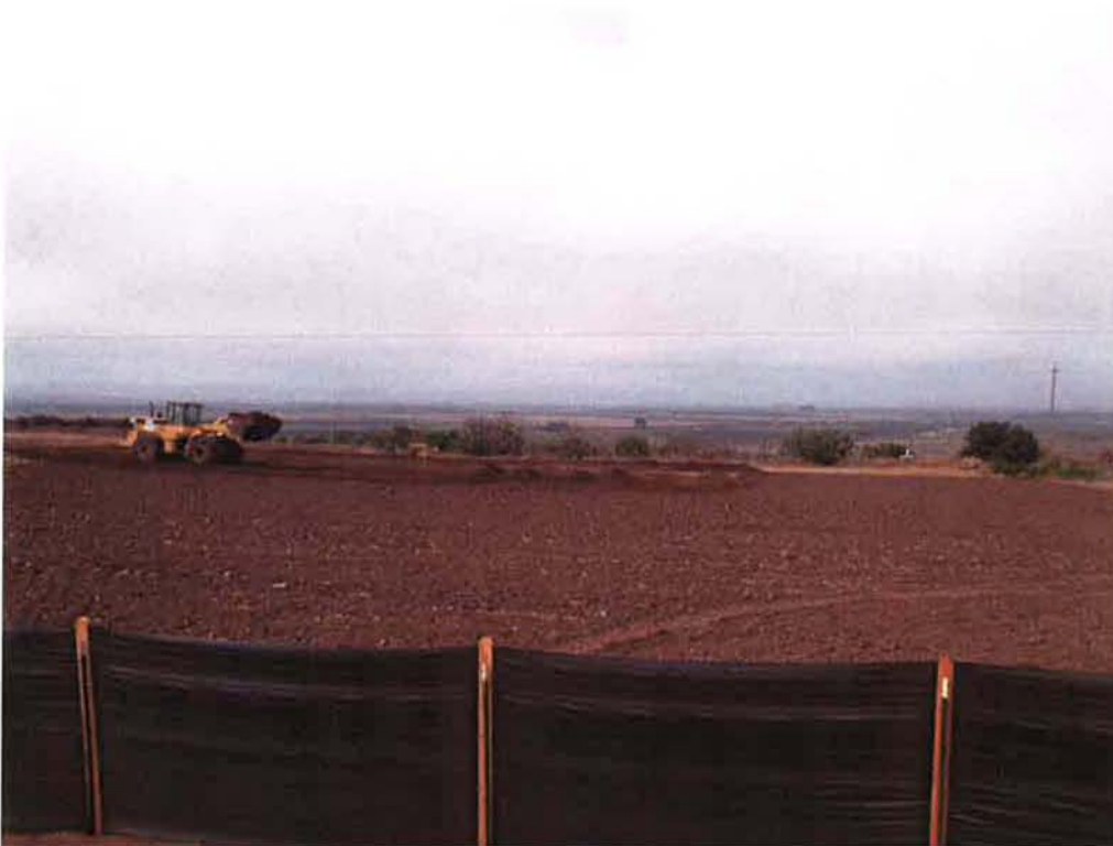
Burke spreading excavated and preserved top soil to the west of the future pump station as directed by Linda Vista Farms.
