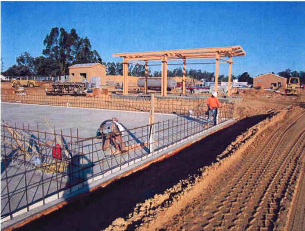
Cushman installing wall construction joints with water stop at Sludge Drying Bed #1.
