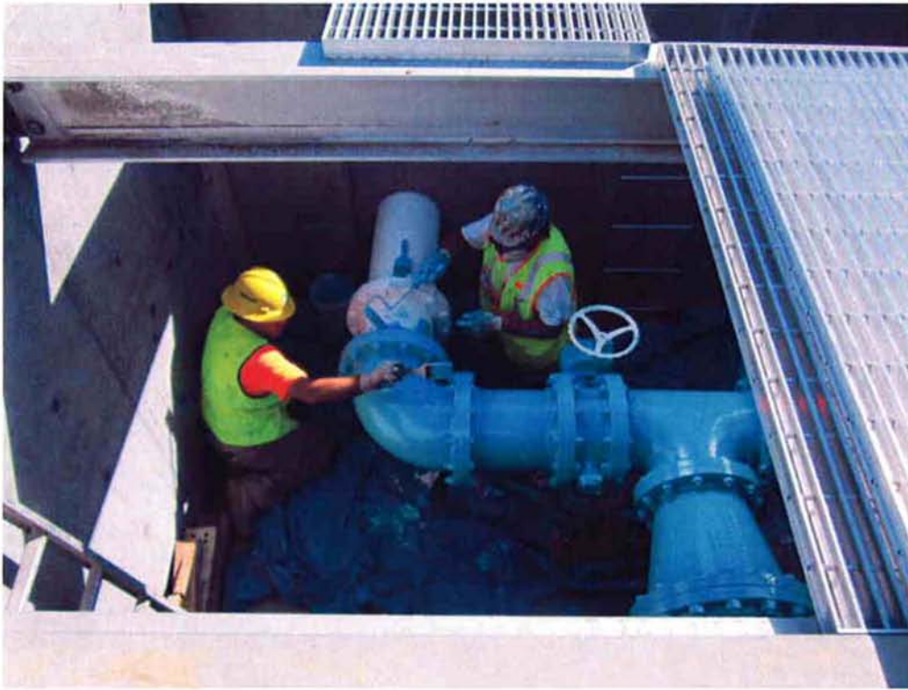
KNK Coating painting AR piping inside the Air Meter and Flow Control Valve Vault.
