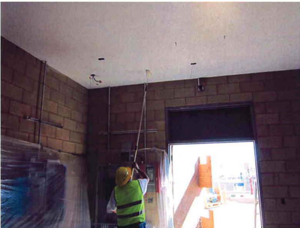
KNK Coating prime coating the ceiling inside the MCC Room of the Electrical/Blower Building.
