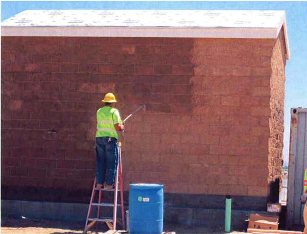
KNK Coating applying Bloc Seal to the outside of the Sodium Hypochlorite Storage Building for waterproofing.
