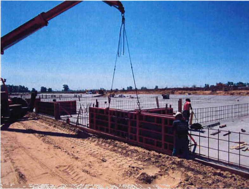
Cushman setting forms for intersections of divider walls at the Sludge Drying Beds.
