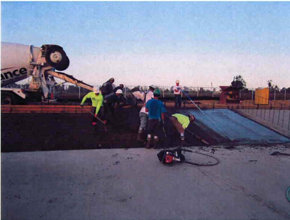
Cushman making final pour of the ramps for the Sludge Drying Beds.
