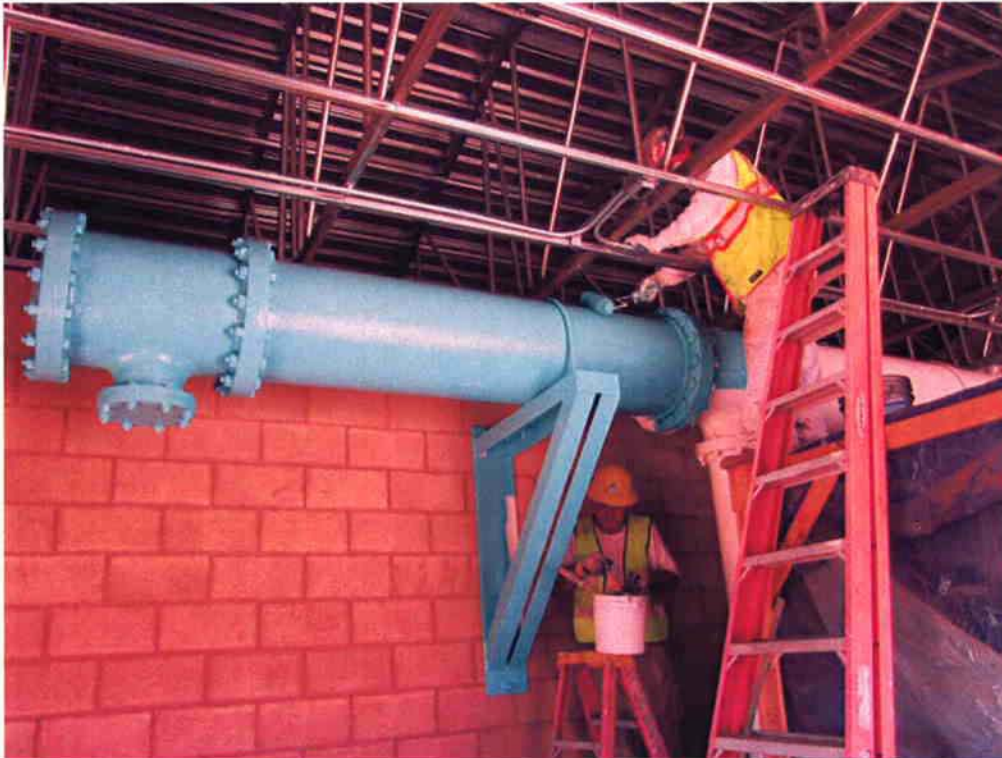
KNK Coating putting finish coat on AR piping in Blower Room of Electrical/Blower Building.
