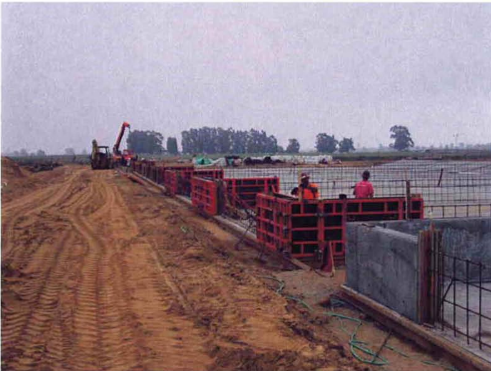
Cushman removing forms for divider wall intersections from the first pour and relocating and installing them for the next pour at the Sludge Drying Beds.
