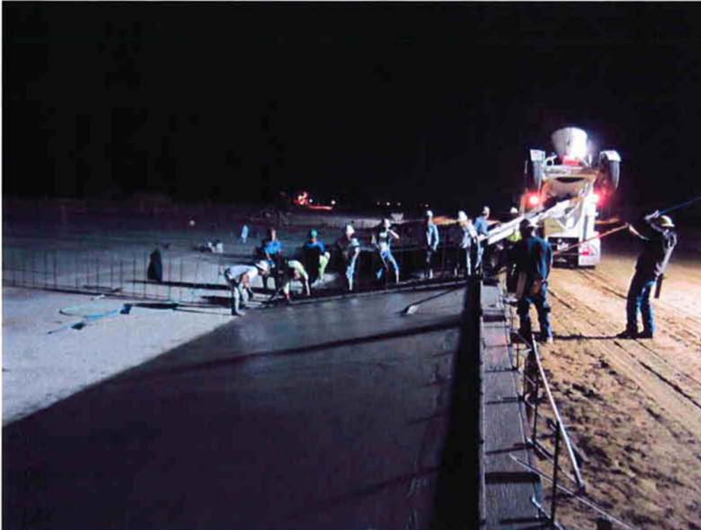
Cushman completing concrete pours of the ramps to the Sludge Drying Beds.
