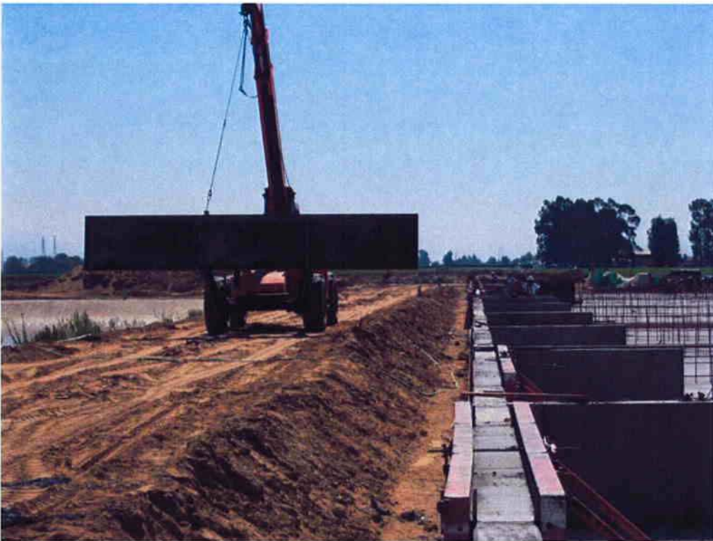
Cushman relocating reusable forms from the west wall concrete pours to the divider walls at the Sludge Drying Beds.
