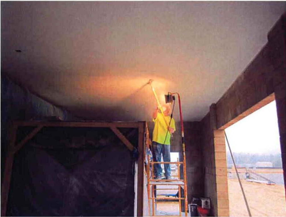
AIT sanding the smooth coating on the ceiling inside the Blower Room of the Electrical/Blower Building.
