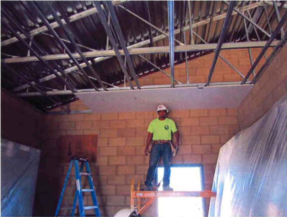
AIT installing sheet rock on the ceiling of the MCC Room in the Electrical/Blower Building.
