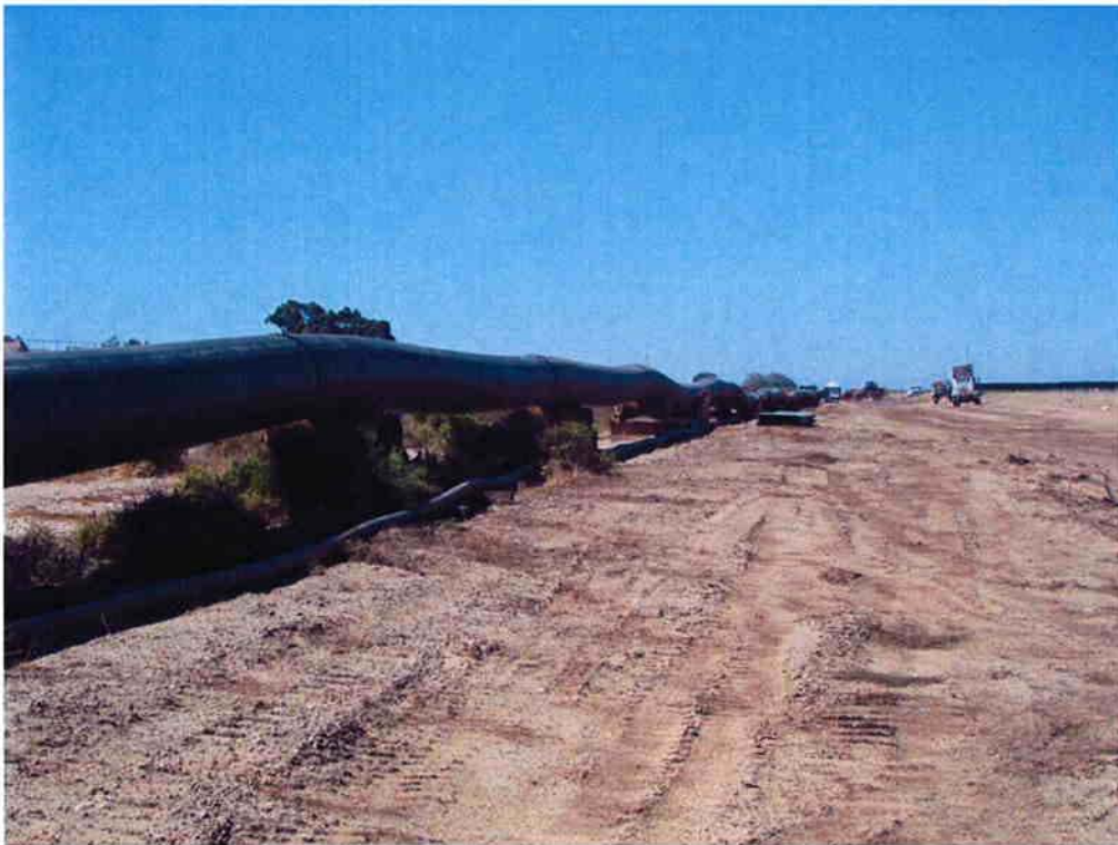
HDPE pipe with one of the 4-inch pipes next to it which will be inserted into the HDPE carrier pipe to provide a ballast and vent to prevent a vacuum when the pipe is pulled into place.
