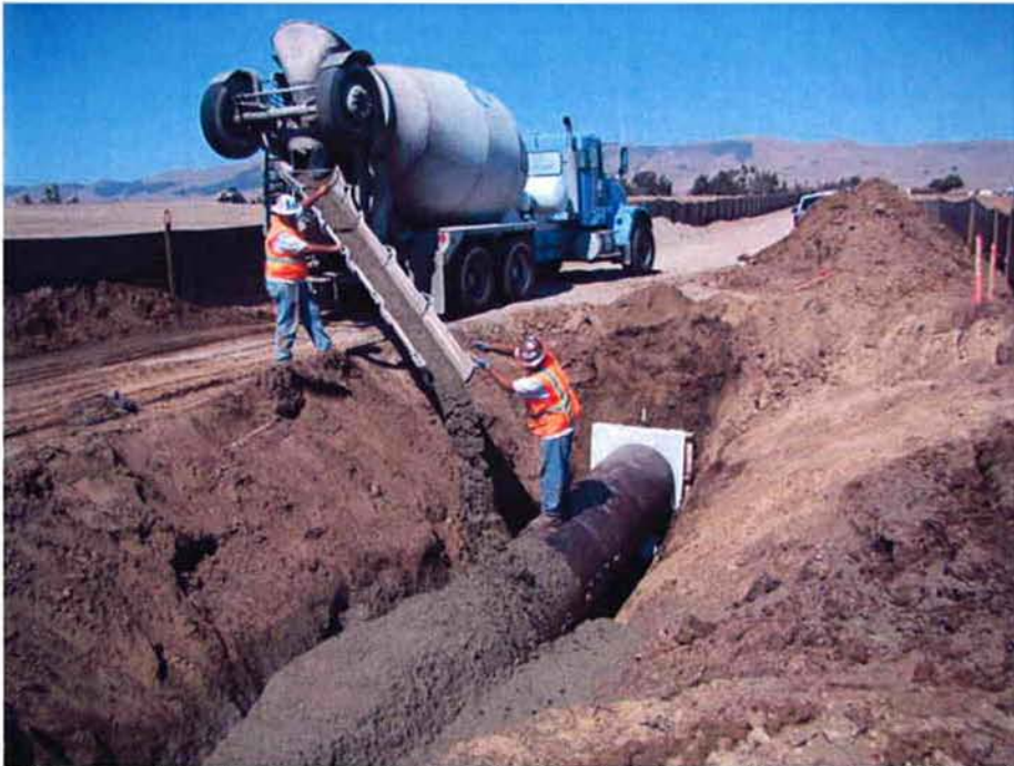
ARB pouring slurry over steel casing before backfilling to install the 18-inch RCP pipes.
