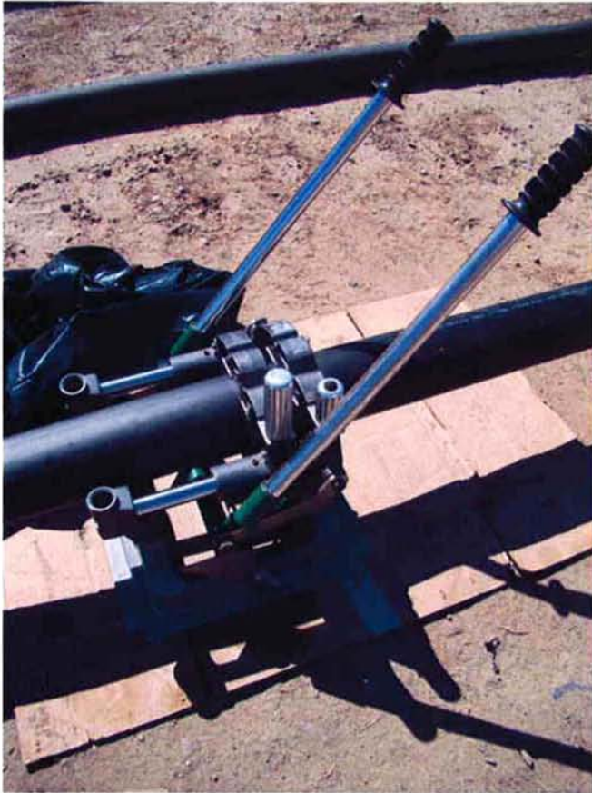
Small machine used to fuse weld the 4-inch ballast and vent pipes.
