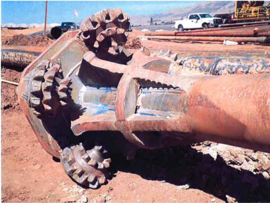
The 36-inch drill after reaching the north side with extensive wear.
