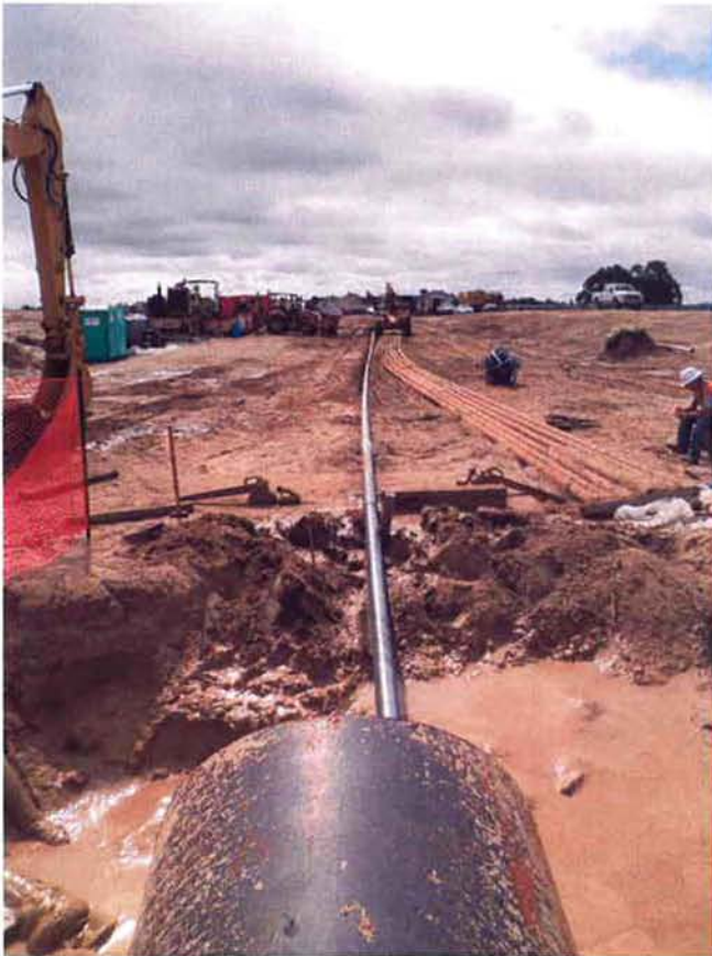
"Tail string" of pipe following the 36-inch drill being pulled from south to north.
