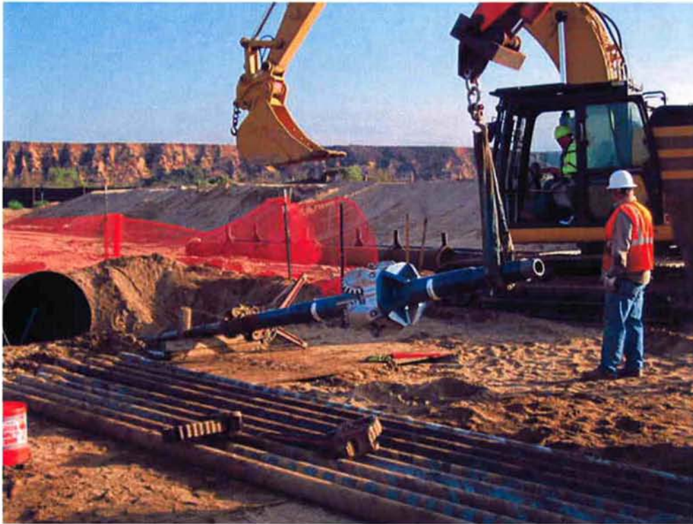
ARB preparing for the 26-inch reaming pass from the south site to the north site.
