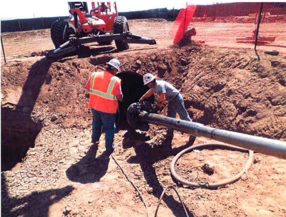
The 26-inch drill emerging from the 54-inch casing completing the 26-inch ream.
