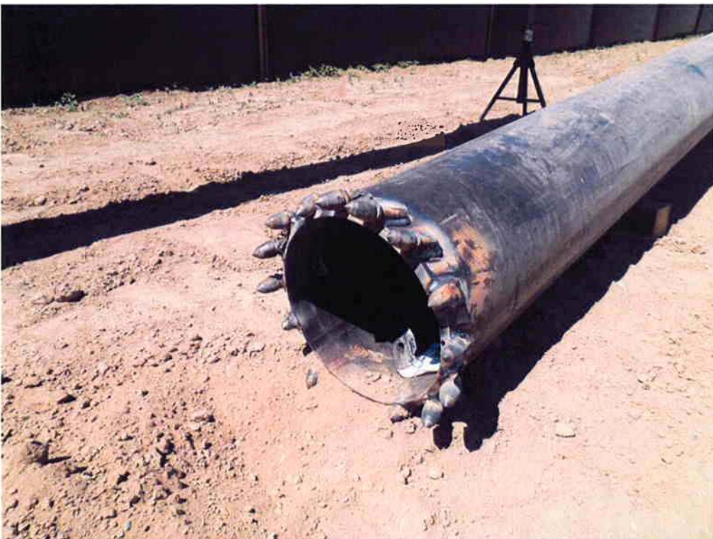
Steel "teeth" welded onto the end of the 12-inch casing to assist with installing it.
