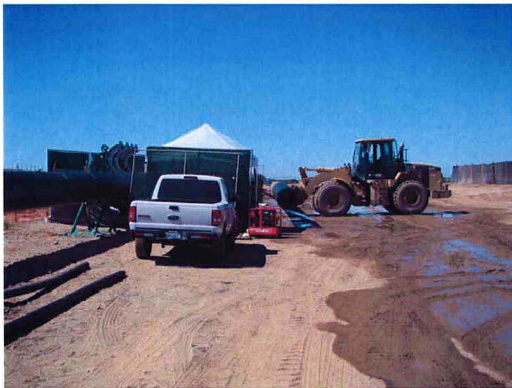
ARB moving another 50 foot section of HDPE pipe into place for fusion welding.
