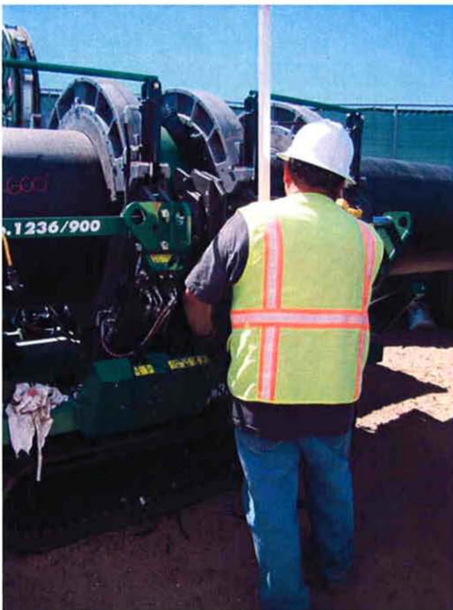
ARB welding operator cutting the pipe ends to achieve a smooth surface for fusion welding.
