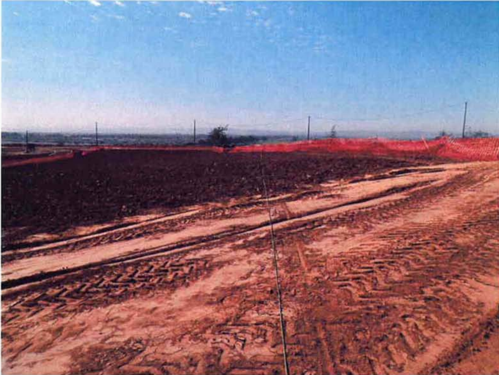
Tracer wire laid out across temporary construction easement from the north site to the bluff edge.
