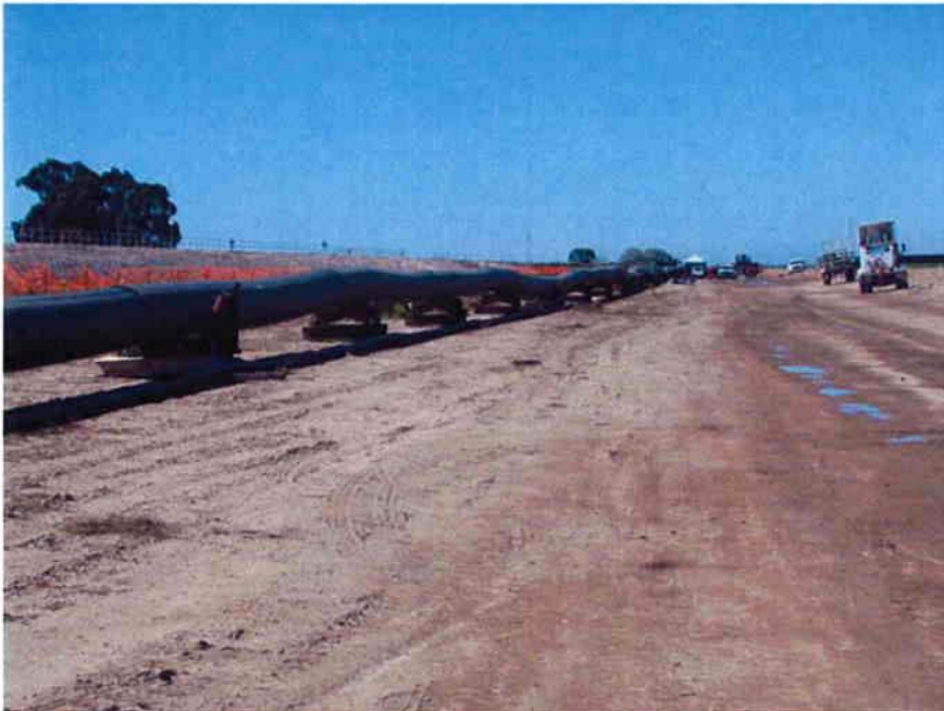
HDPE pipe laid out to the east of the site on rollers along the north side of the levee after being fusion welded.
