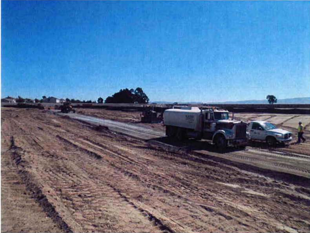
ARB building access road into south site due to soft, uncompacting native soils.
