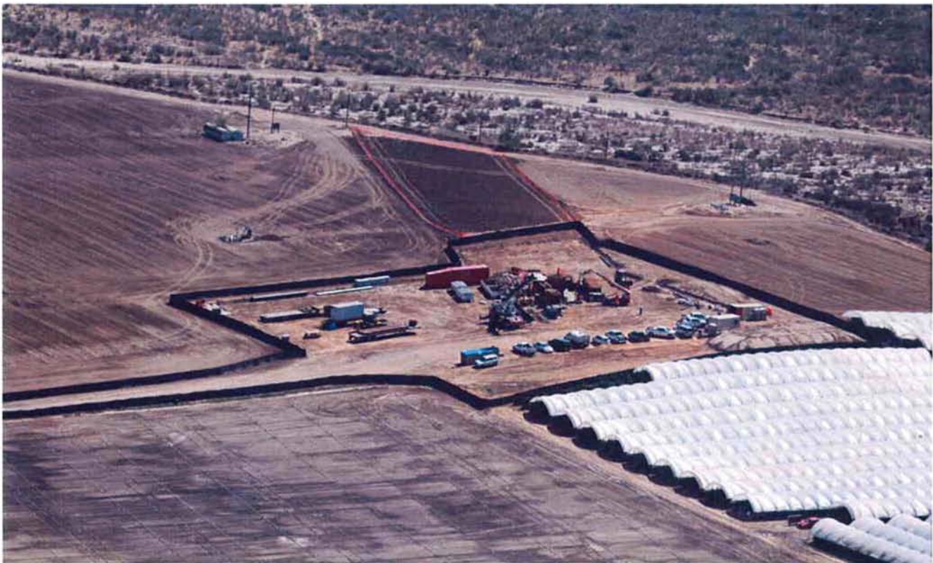
Aerial view of the north side of the project with ARB drill rig and equipment mobilized.
