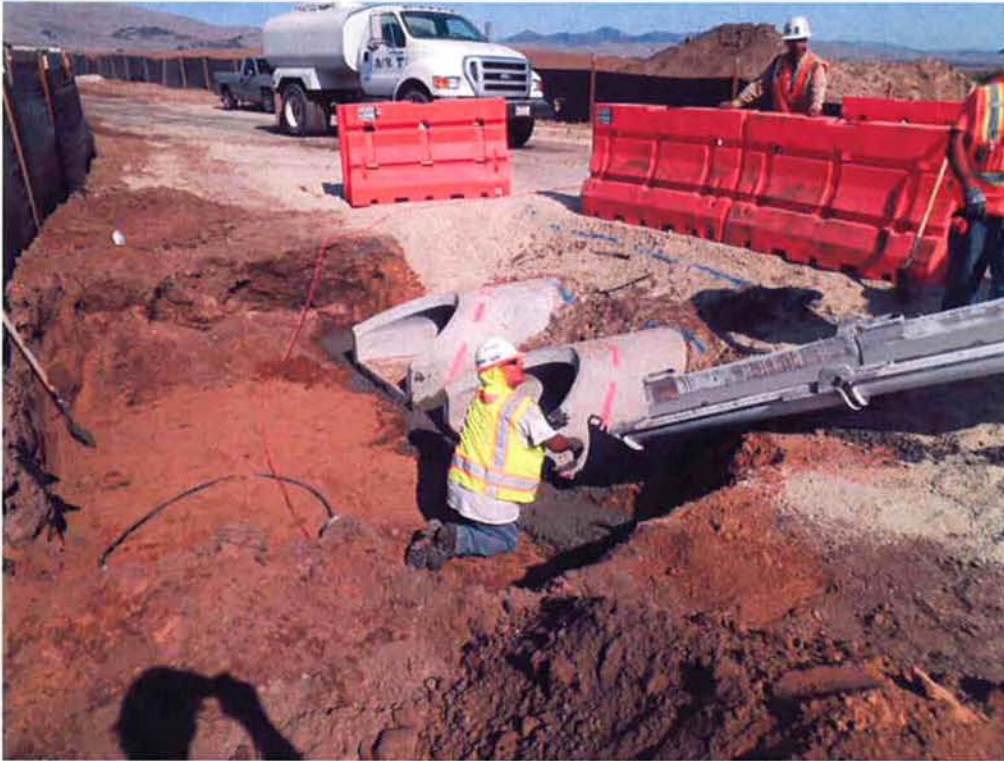
ARB pouring concrete cut-off wall at the end of the 18-inch RCPs.
