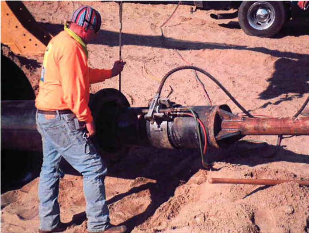
ARB's welder cutting the end of the 12-inch casing after it is in place.
