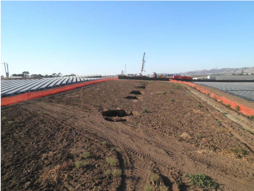
Sink holes when initially discovered on October 14.
