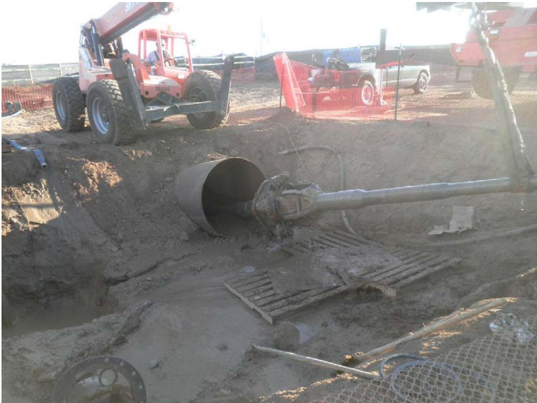
ARB removing 36-inch drill after it became stuck due to material settlement during the second reaming pass on October 16.
