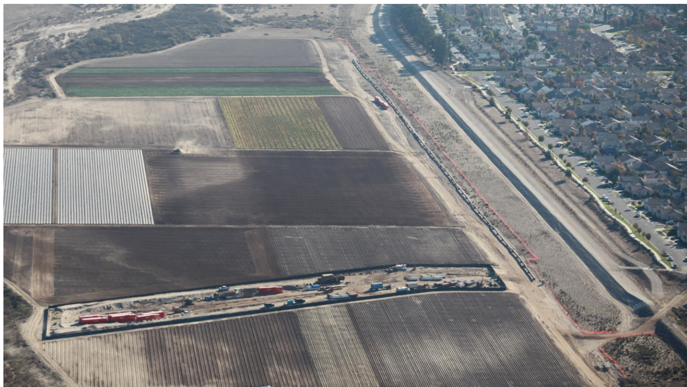
Aerial photo of the south side with ARB's equipment and the HDPE pipe fused and laid out to the east.
