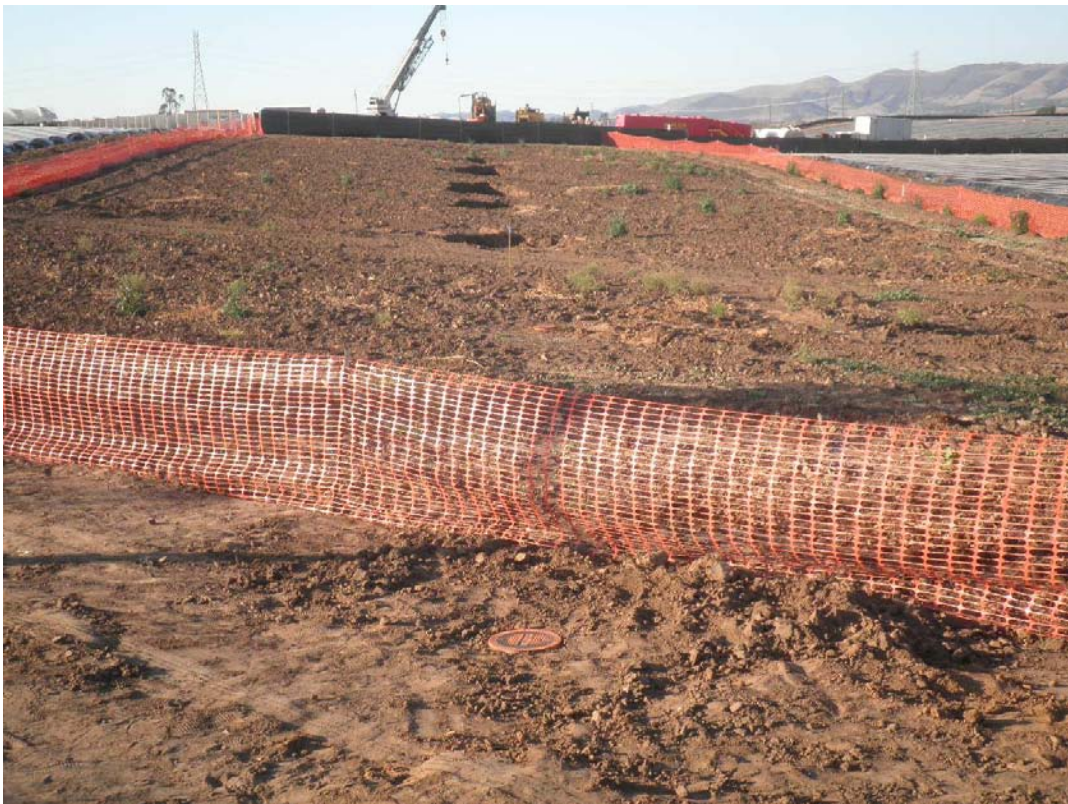
Settlement monitors installed by ARB to monitor further settlement closer to the edge of the bluff.
