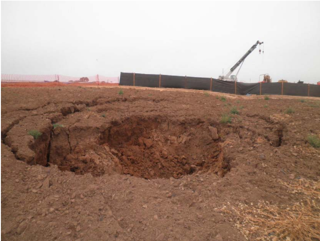
Sink holes increasing in size with continued reaming.
