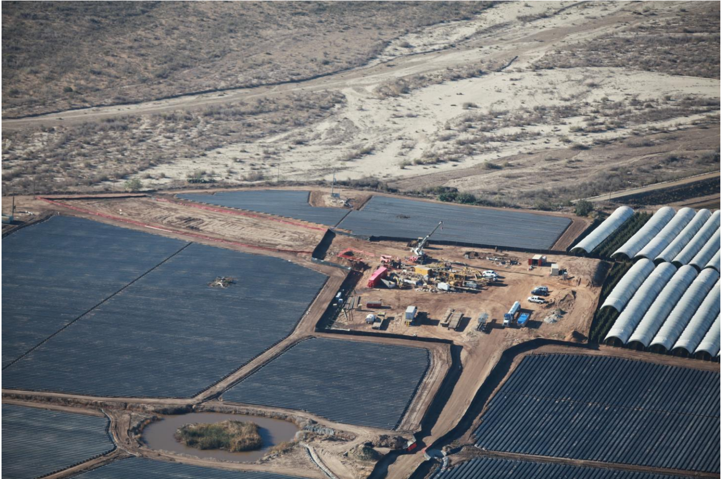
Aerial view of the north side of the project with orange fencing around area where permeation grouting occurred.
