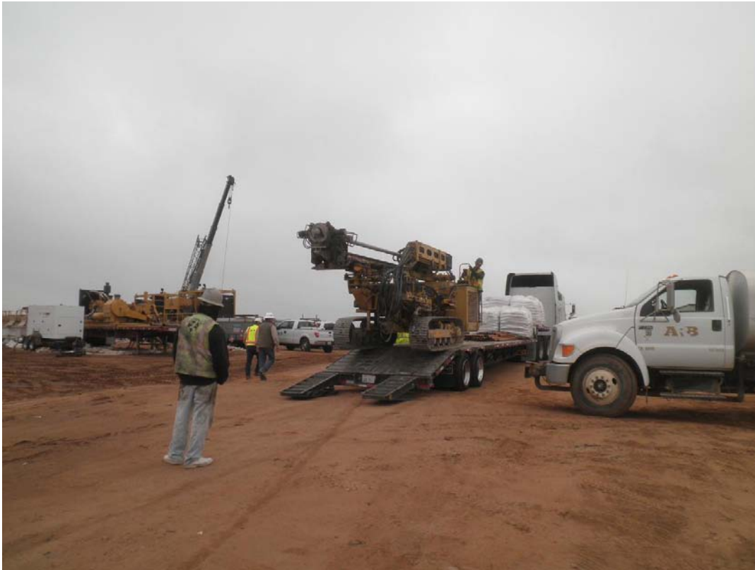
GeoGrout mobilizing one of their drill rigs to the north site on October 23.
