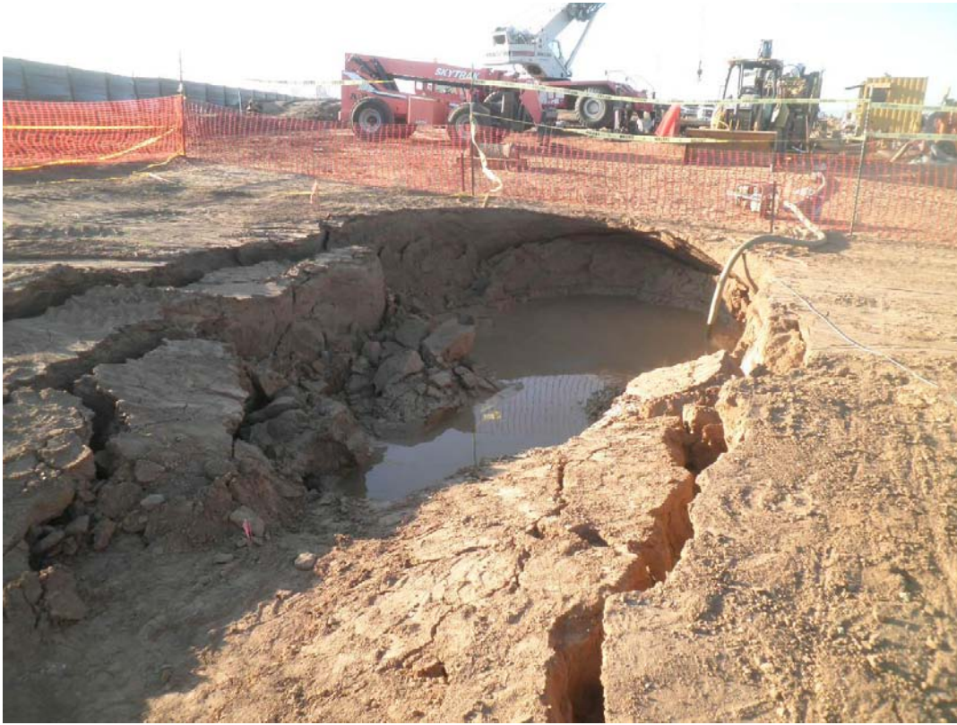
Mud rising in sink hole within the temporary construction easement area as ARB proceeds with the 42-inch ream on October 21.
