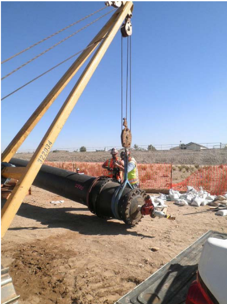
ARB installing welded flanged adapter and DIP reducer with pressure test fitting to the west end of the HDPE pipe.
