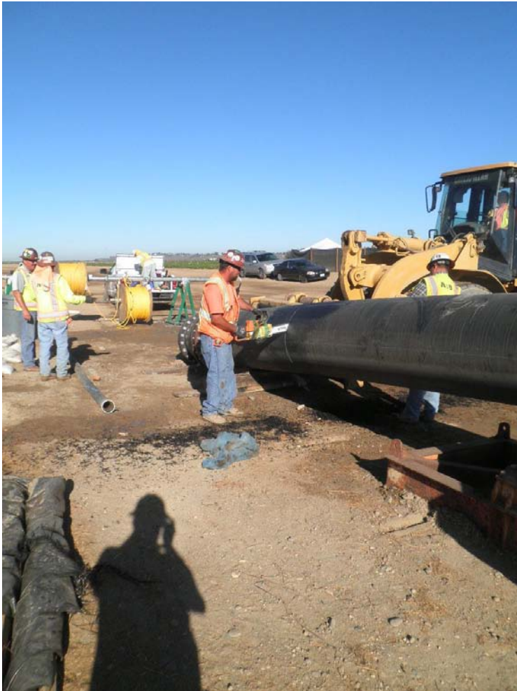
Removing flanged adapter and DIP reducer from west end of pipe after hydrostatic pressure test.
