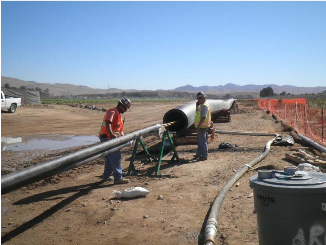
ARB positioning the two 4-inch pipes for pulling into the HDPE pipe.
