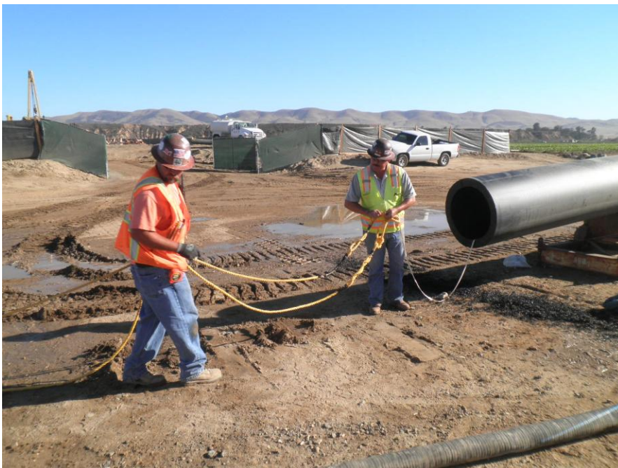
ARB using mule tape and rope to prepare for pulling of two 4-inch pipes (ballast and vent) into HDPE pipe.
