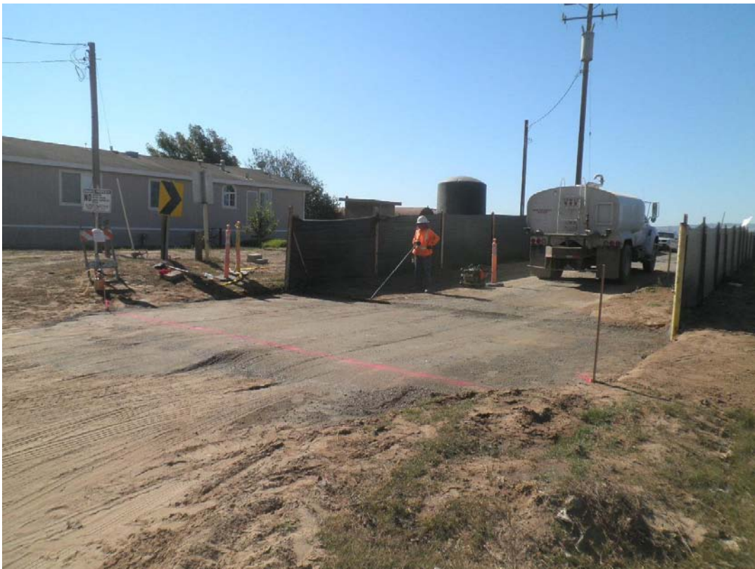
R. Burke Construction placing base for installation of a gate at the site entrance to prevent CRLFs from entering the site.
