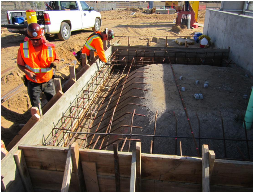
Reinforcing and forms being installed for the trash enclosure slab at the Headworks.
