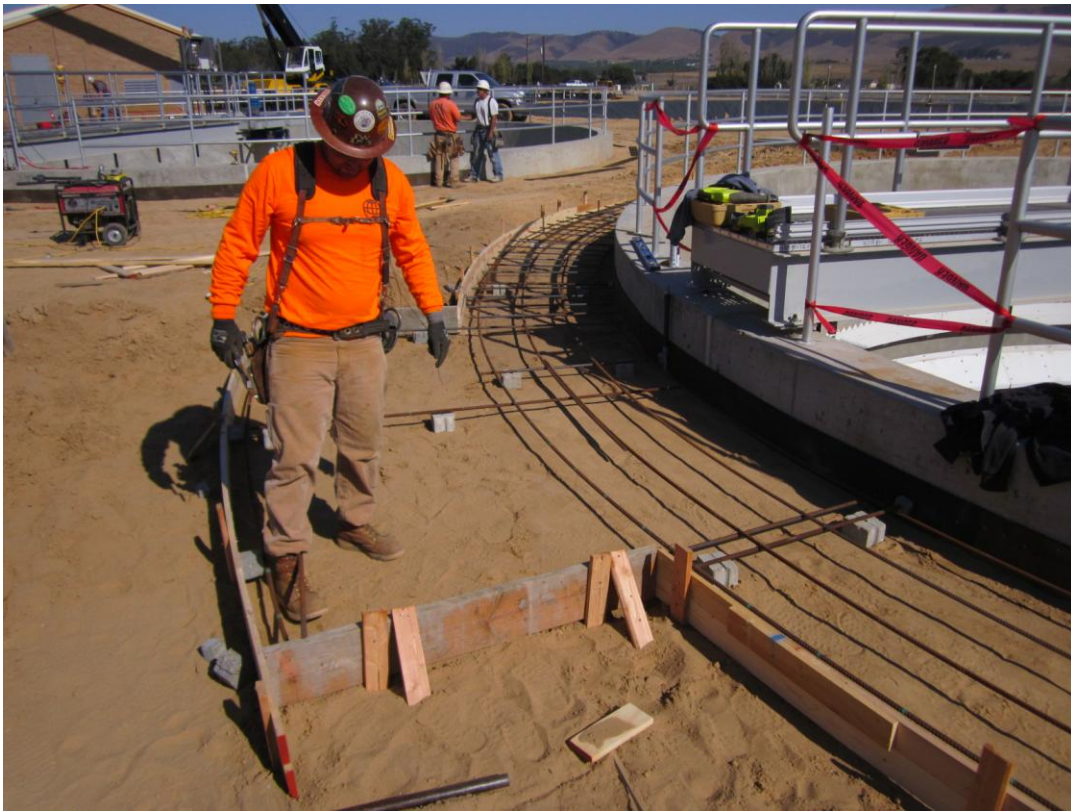
CMC Rebar and Cushman installing reinforcing and forms for sidewalk around Clarifier #1.
