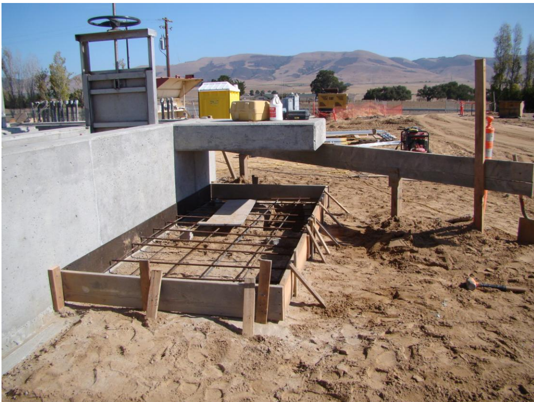
Forms and reinforcement for one of the stair landings at the Headworks.
