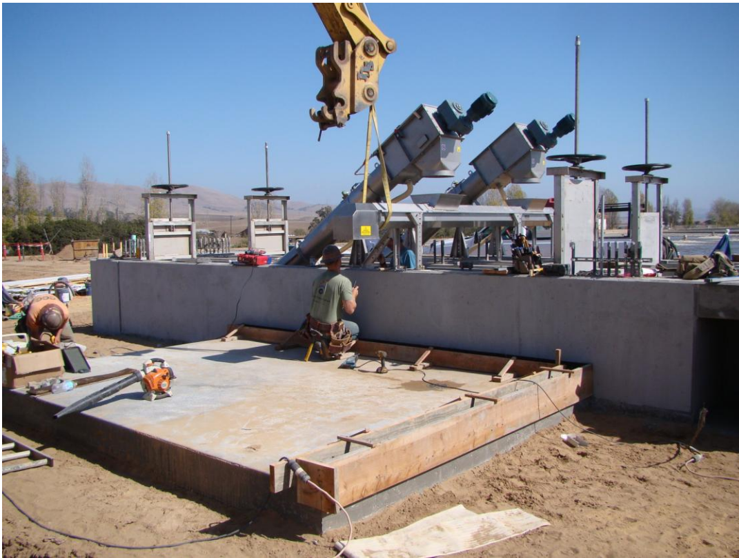
Cushman forming the curb at the trash enclosure slab and locating the screw screens at the Headworks before removing them to allow KNK Coatings to coat the channels with Carboline.
