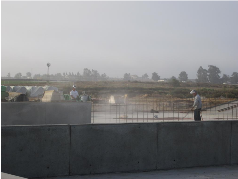
Cushman sandblasting concrete and reinforcing to prepare for next wall pour at Sludge Drying Beds.
