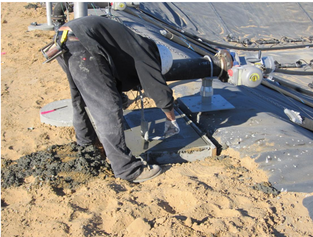
Cushman pouring pipe support pads for AR piping at the Aeration Basin.
