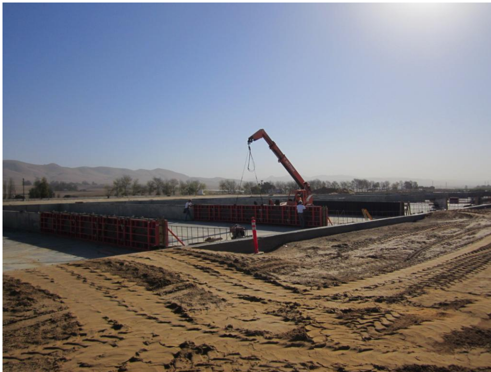
Cushman moving wall forms for next wall pour at Sludge Drying Beds.
