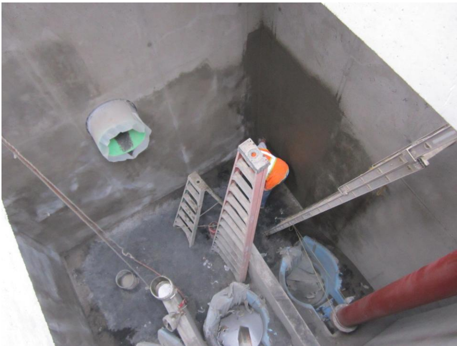
KNK Coating applying non-shrink grout to the inside of the Influent Pump Station in preparation for applying the Carboline coating.
