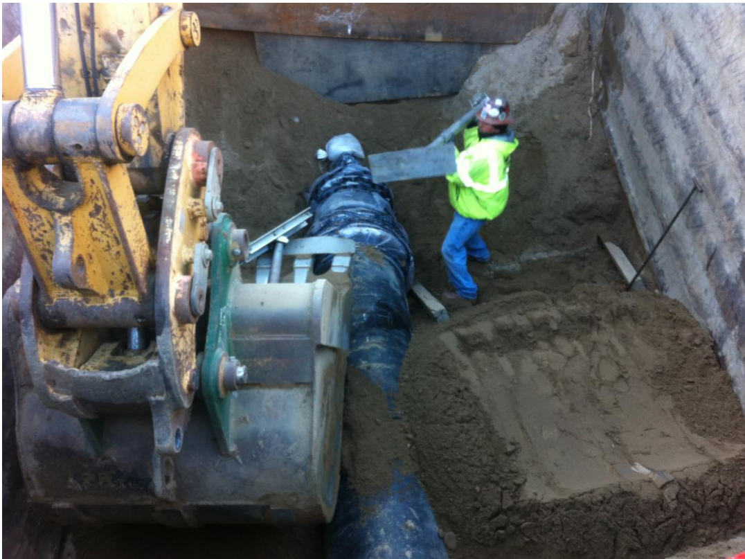
ARB removing hydraulic shoring jacks holding pipe in place after securing with compacted backfill.
