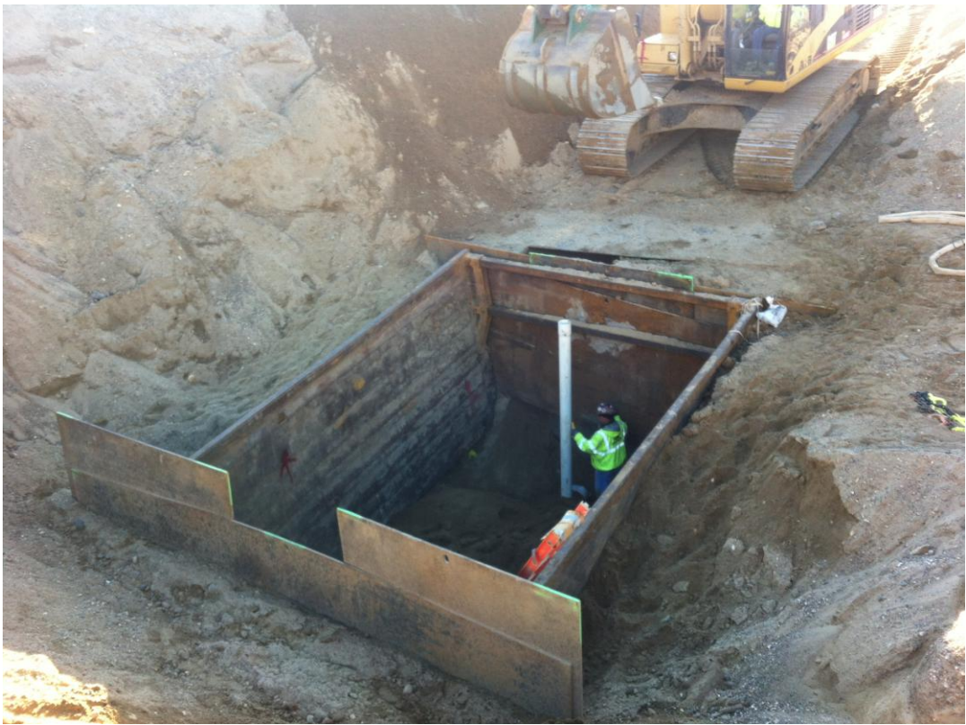
ARB installing 4-inch gate valve and riser at the end of the pipe.
