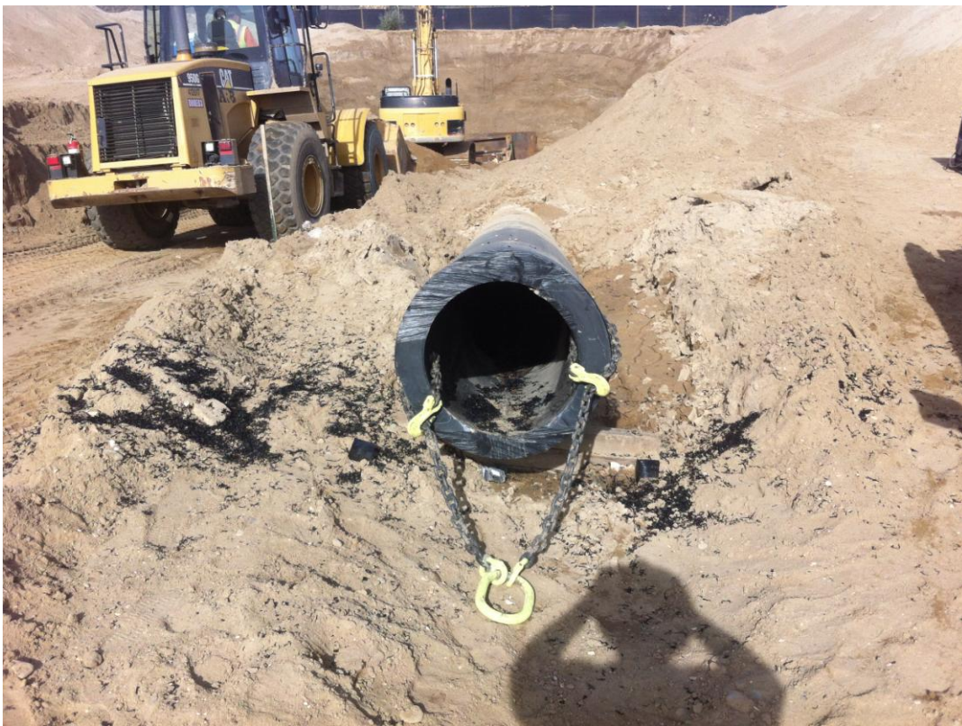
End of pipe at the surface, cut and ready for removal from remaining pipe which is at grade.
