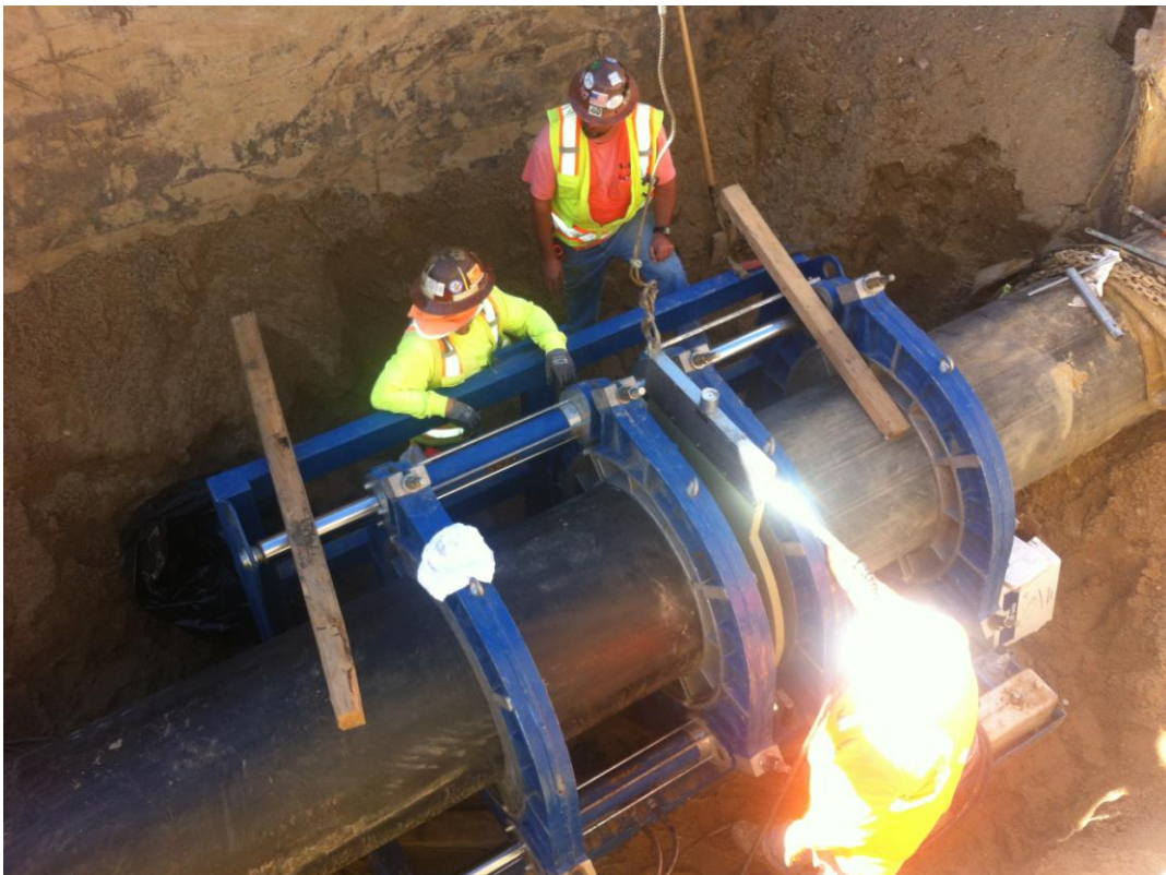
Pipe fusing machine in place with heater plate between HDPE pipe ends (reaches 472 degrees F).
