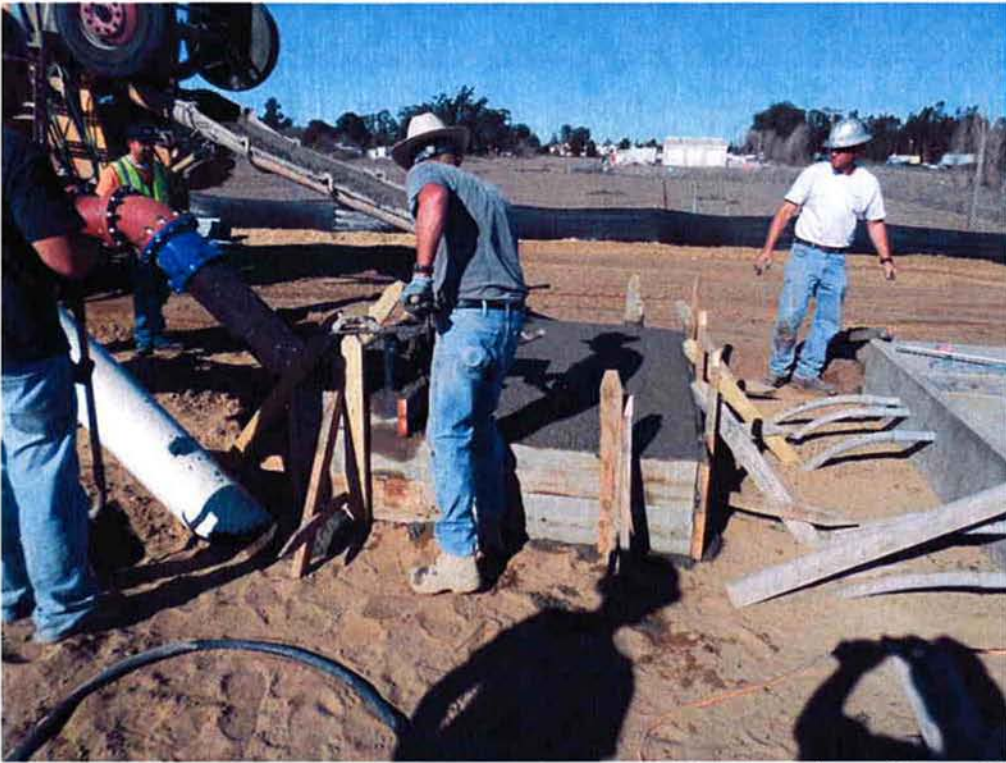
Cushman pouring concrete at the control panel pad for the Influent Pump Station.
