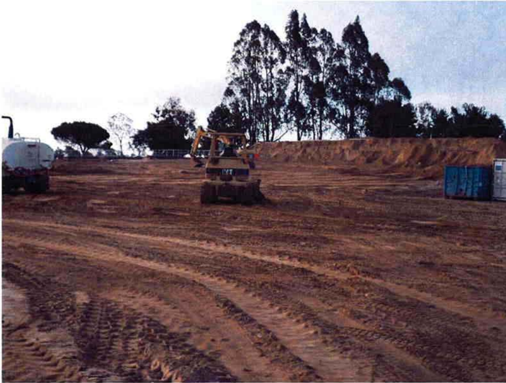
Cushman performing site grading to the north west of the Electrical/Blower Building.
