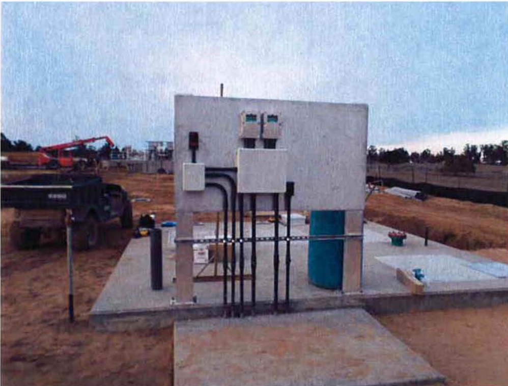
Pull boxes, level transmitters and disconnect switches installed at the control panel rack at the Influent Pump Station.
