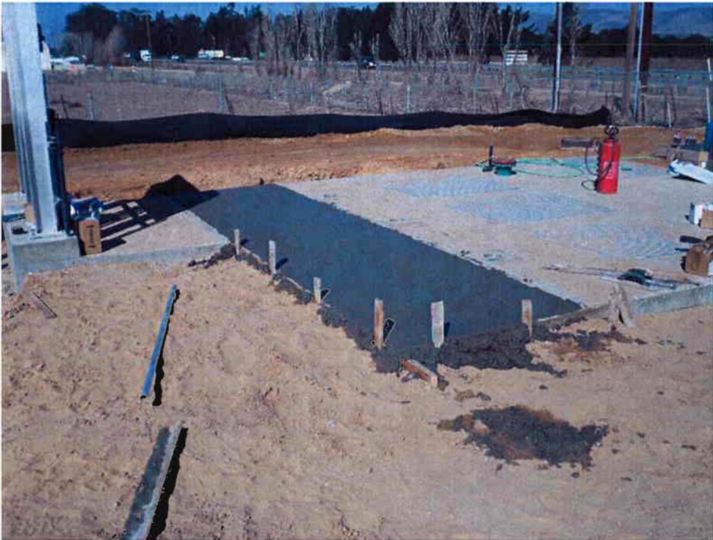
Cushman pouring sidewalk section between Influent Pump Station and the control panel pad.
