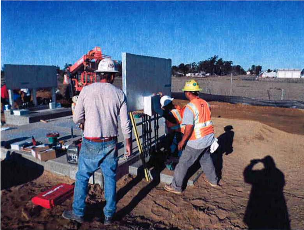
Bergelectric installing the aluminum stand and conduit for the control panel at the Influent Pump Station.
