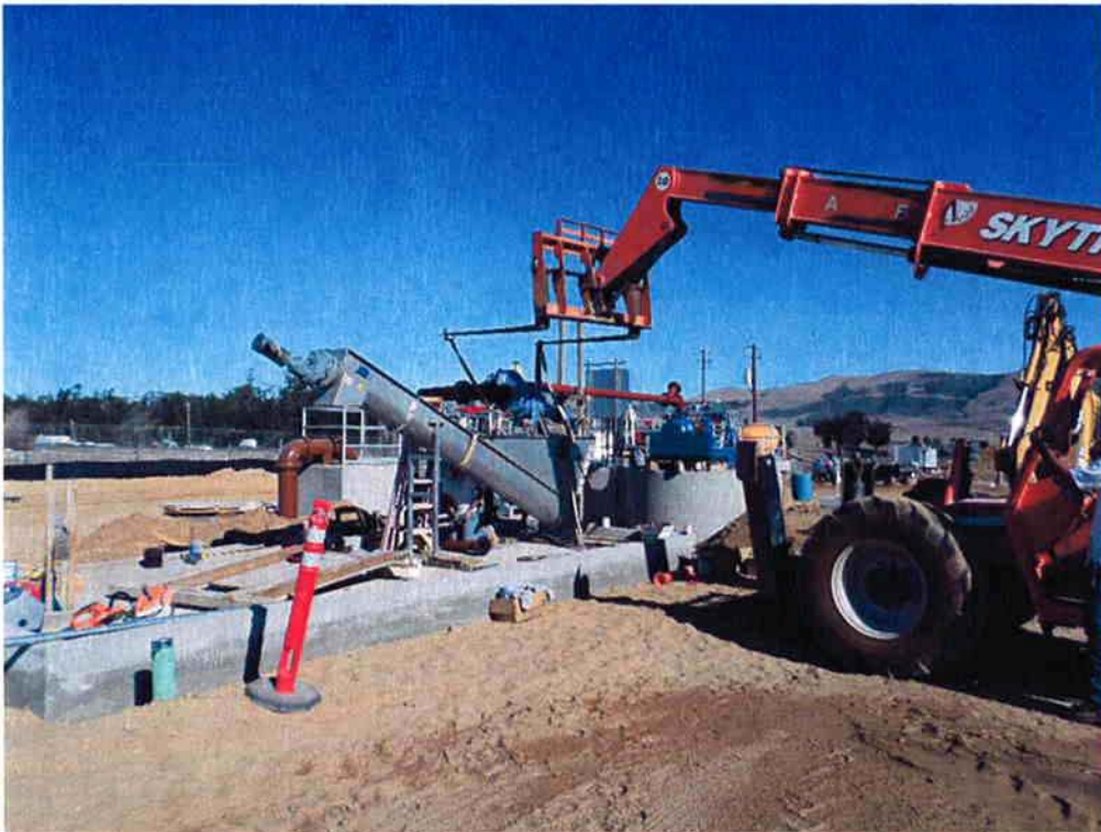
Cushman installing the piping from the Grit Pump to the Grit Classifier.
