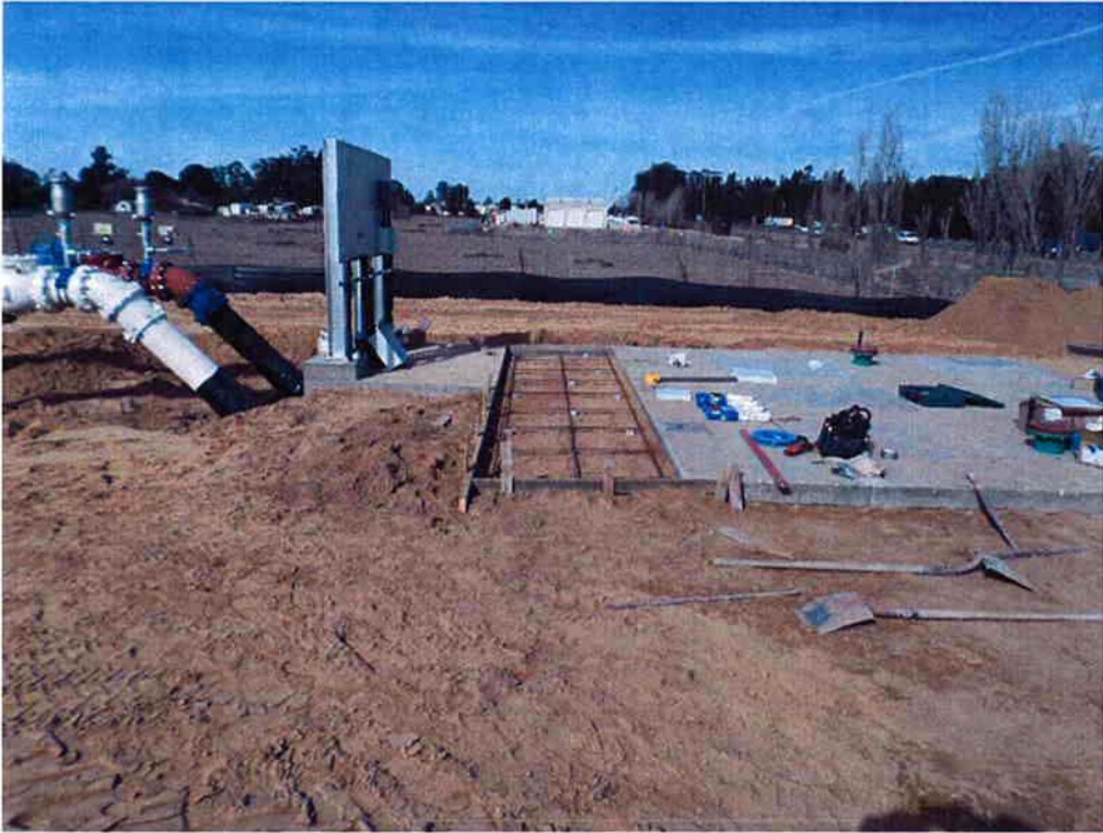
Forms and rebar for sidewalk between the control panel pad and the Influent Pump Station.
