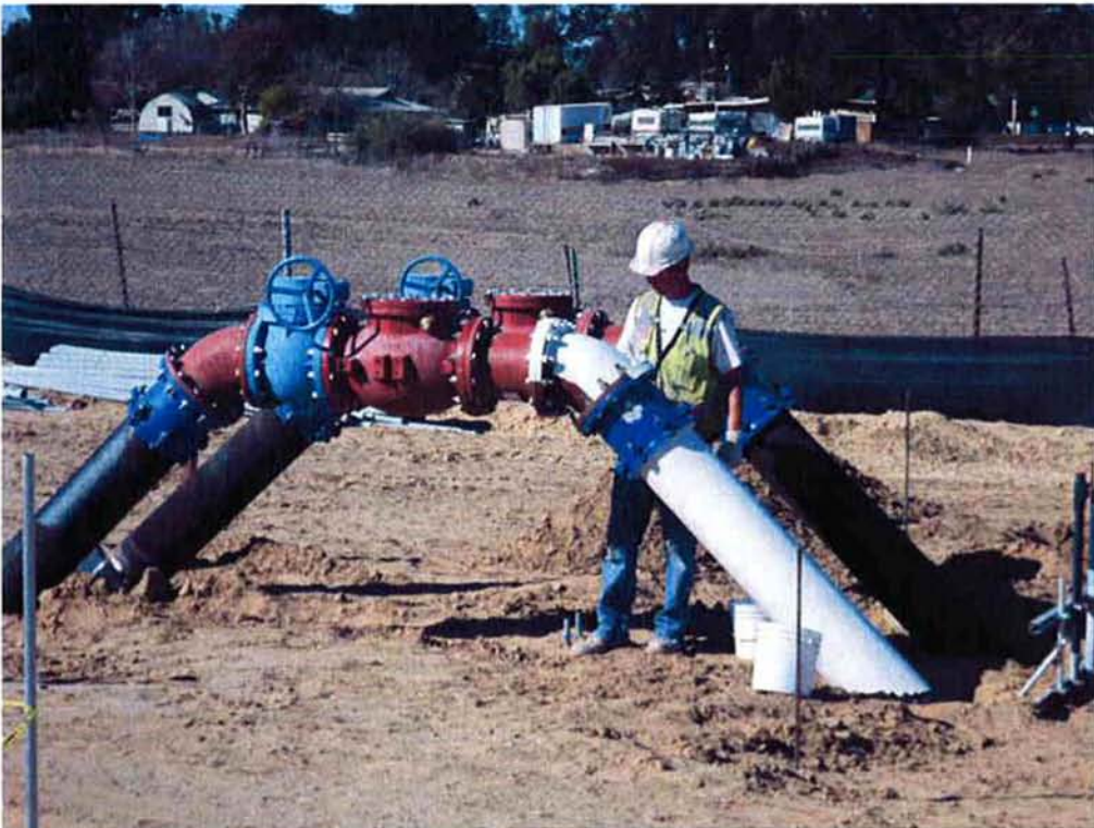
KNK Coating applying primer to the RW piping between the Influent Pump Station and the Headworks.
