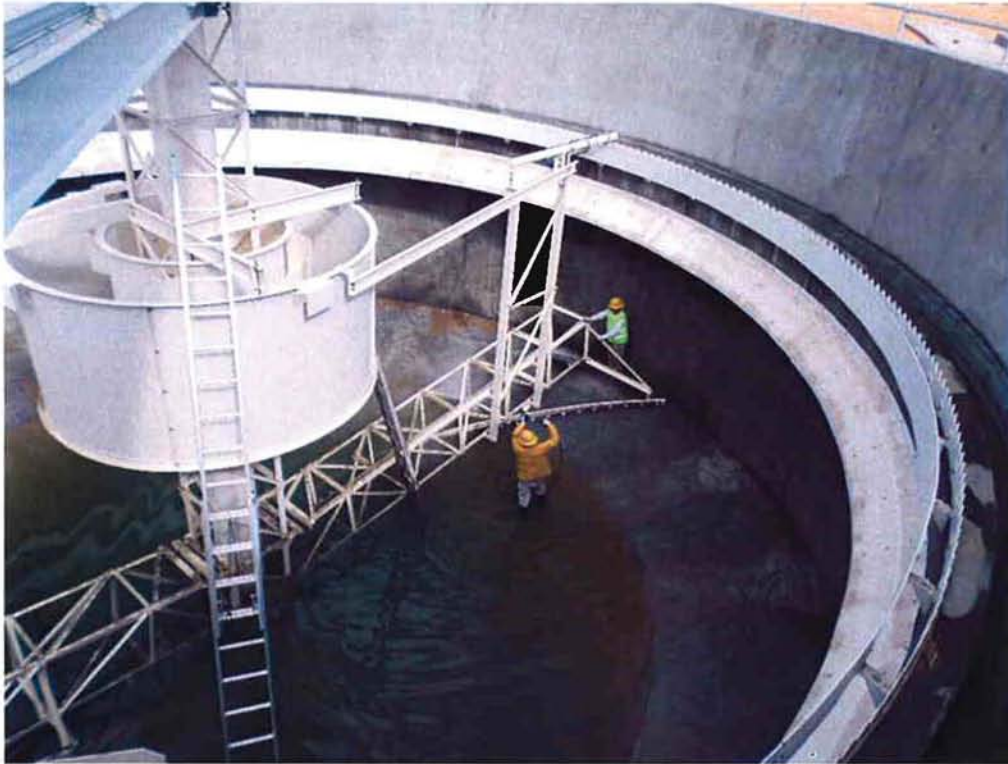
Draining and power washing inside Clarifier #2 in preparation for repair of corroded areas.
