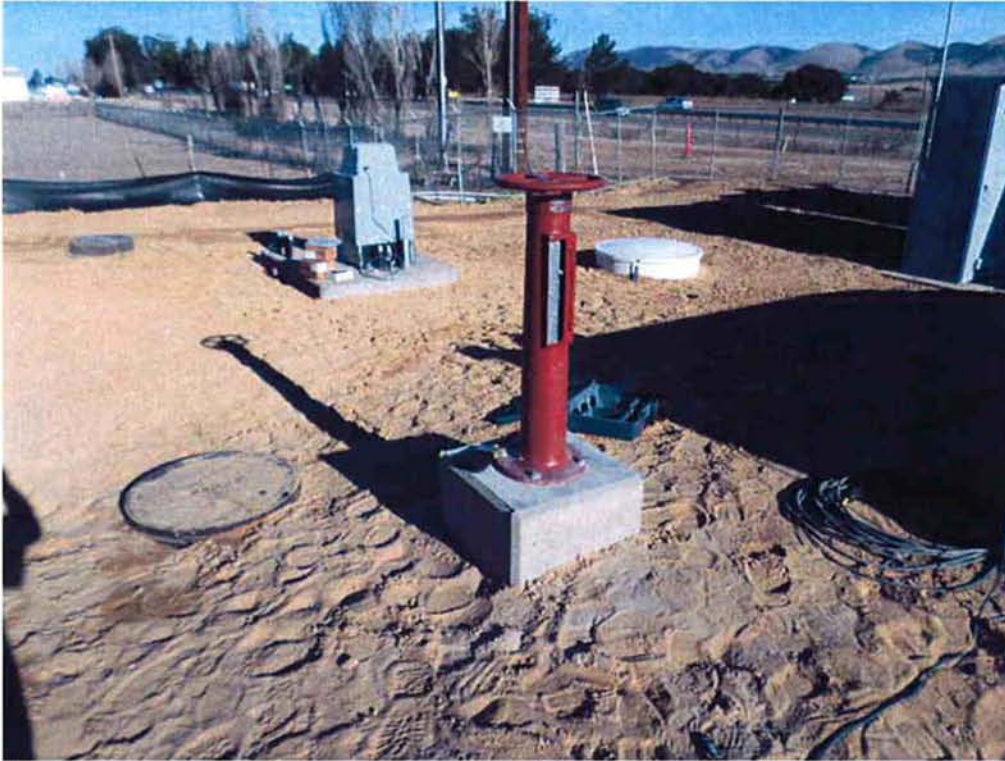
Cushman mounted the valve operator at the truck wash down station.
