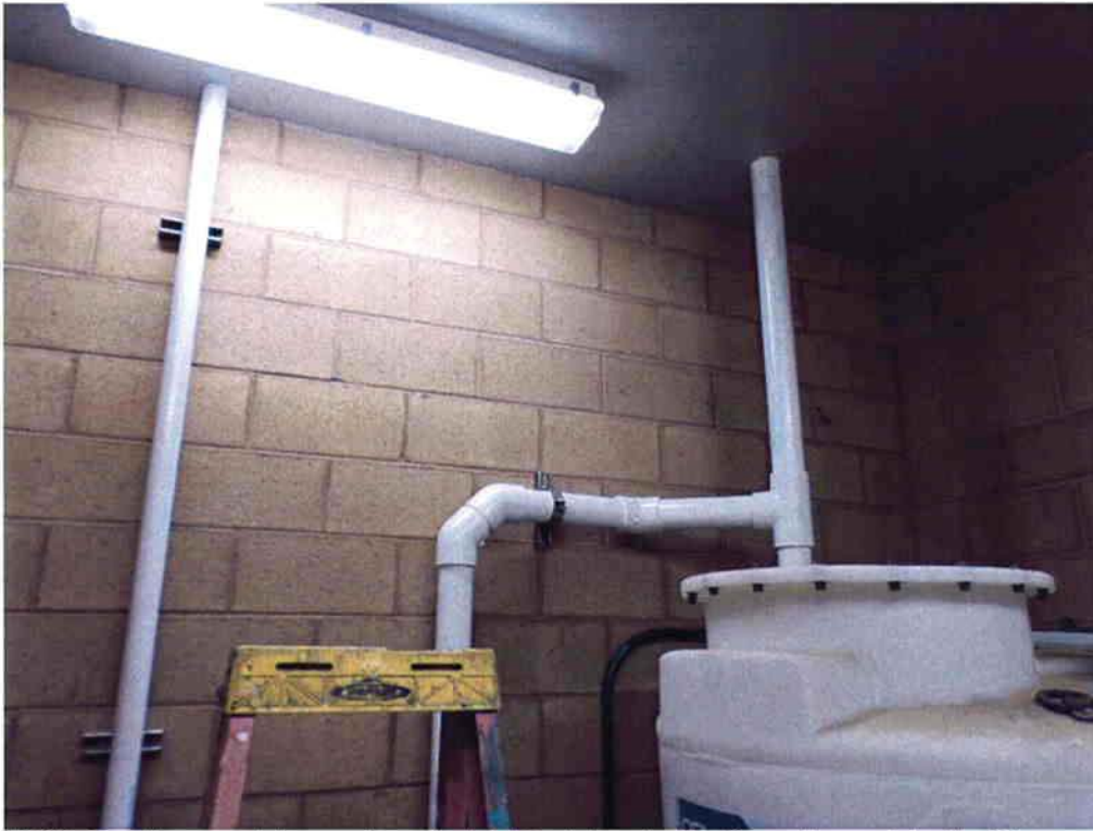
KNK Coating applying primer to PVC piping in Sodium Hypochlorite Storage Building.
