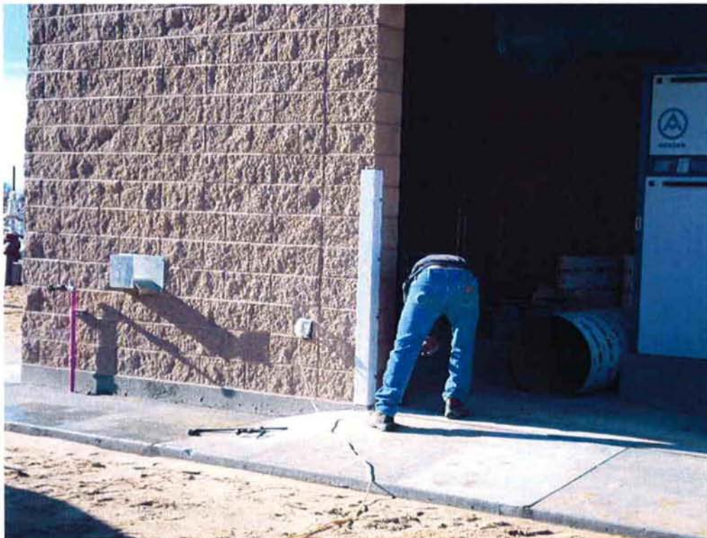
Cushman installing corner guards at the roll-up door in the Electrical/Blower Building.
