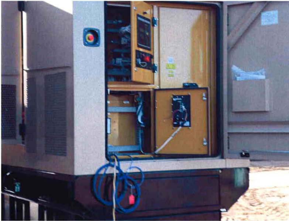
Start-up of new emergency generator.
