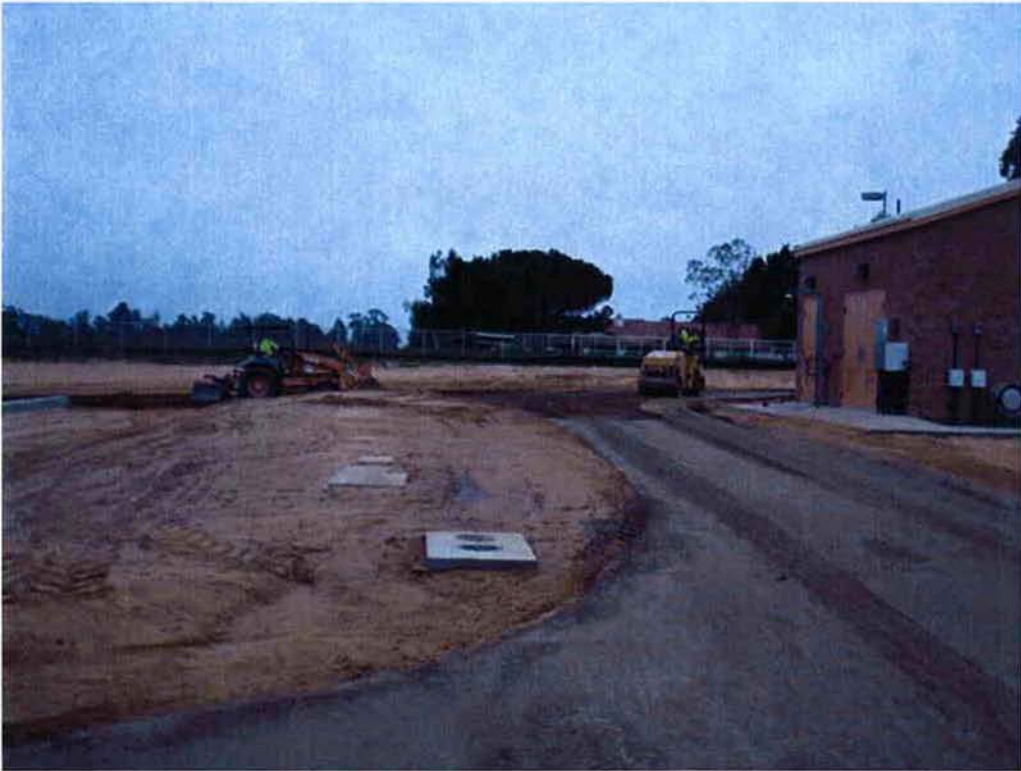
Mark Switzer Excavating compacting aggregate base material for roadways around the site.
