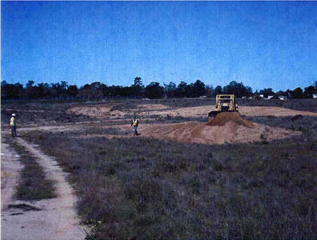
Rincon staff on site during clear and grub by Mark Switzer Excavating for Alternative Y work to build new Infiltration Ponds 9 & 10.
