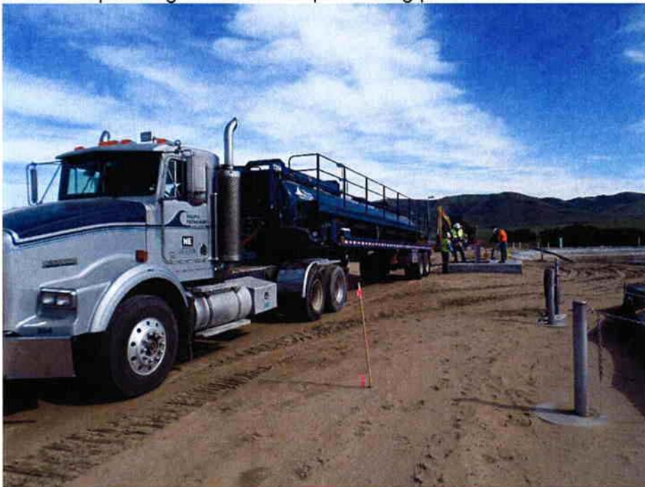
Cushman and District taking delivery of activated sludge from San Luis Obispo to seed the new treatment plant.
