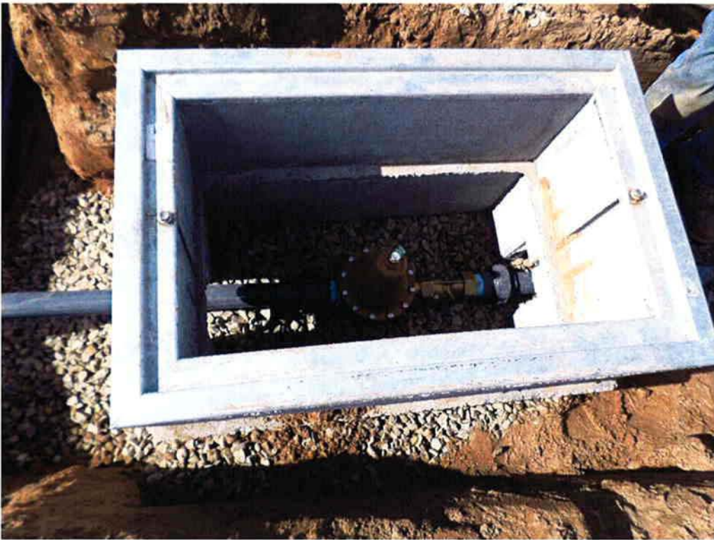
Pressure reducing installed on the 2-inch potable waterline.
