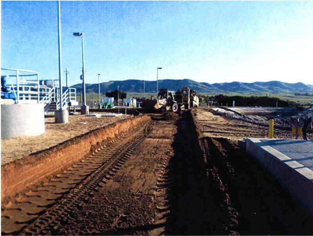
Mark Switzer Excavating cutting the new road to subgrade near the Headworks.
