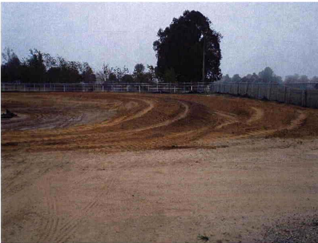
Start of new berm for landscape and screening from neighboring properties using material excavated from Alternative Y work.
