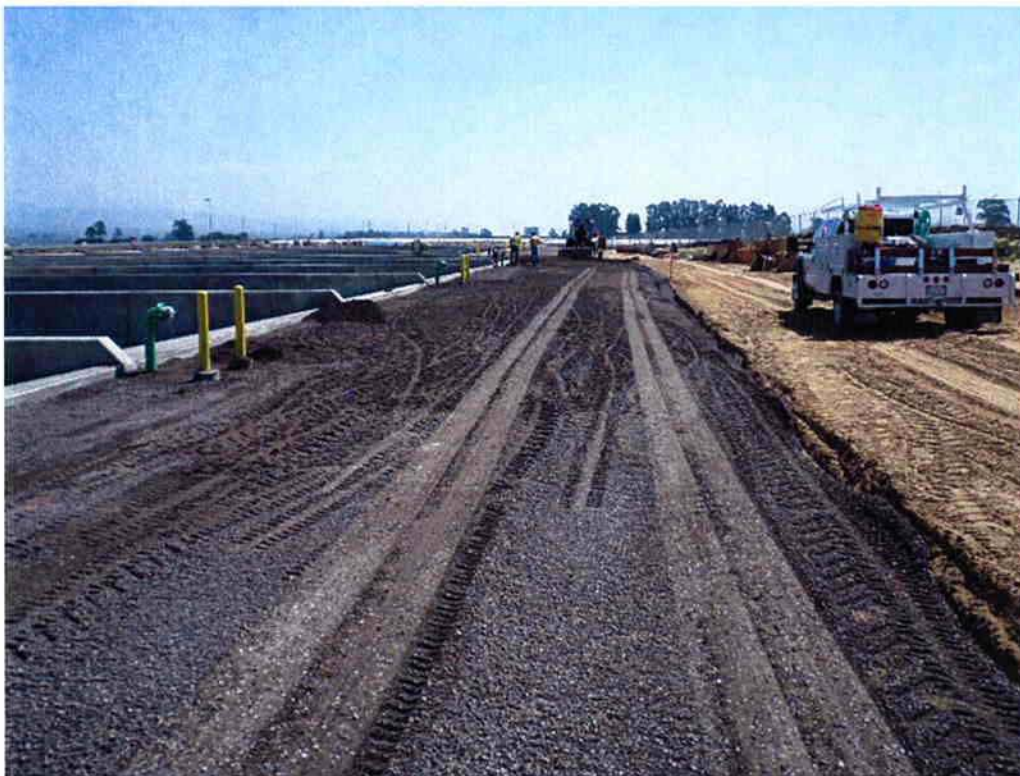
Mark Switzer Excavating placing aggregate base for roadway at the Sludge Drying Beds.
