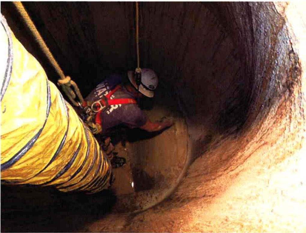
Cushman plugging the existing influent pipe penetration in the influent manhole after the plug for the new influent pipe was removed.
