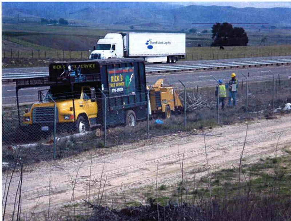
Rick's Tree Service removing trees from the east side of the WWTF, along Highway 101, as part of the new landscaping plan.
