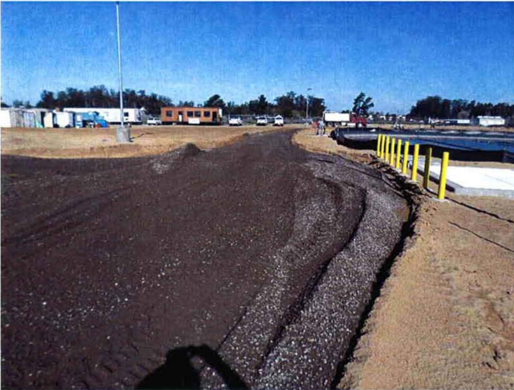
Mark Switzer Excavating placing aggregate base material for roadways around the site.
