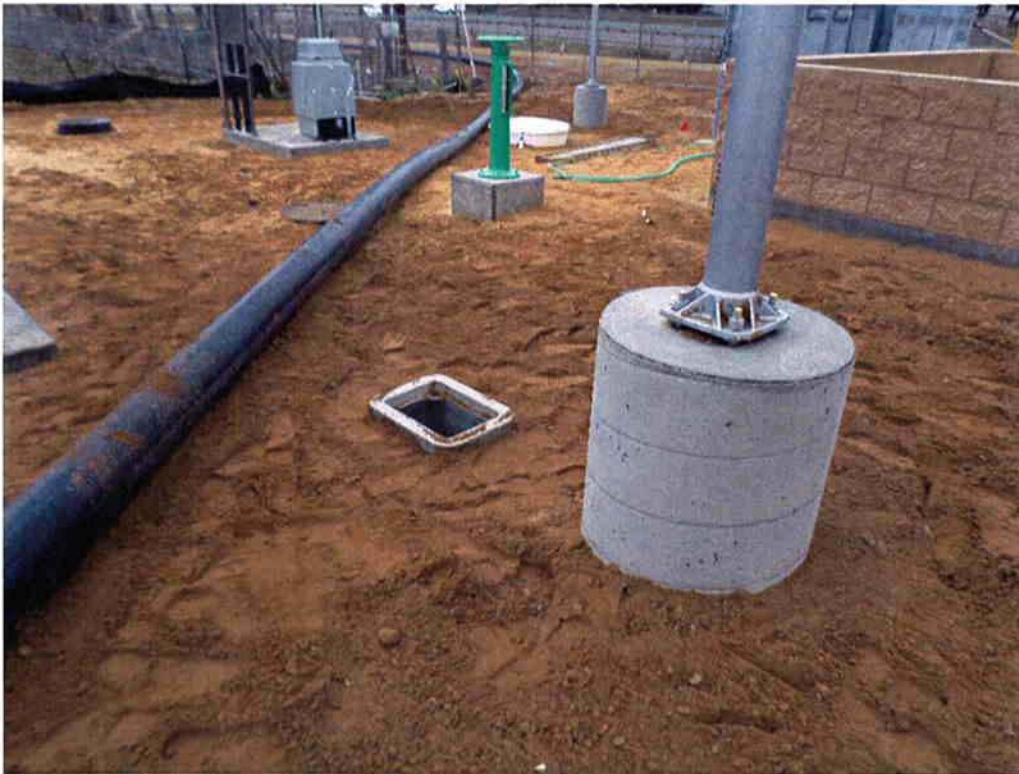
Bergelectric installing street light pull boxes and the temporary bypass pipe for the tie-in to the new treatment plant.
