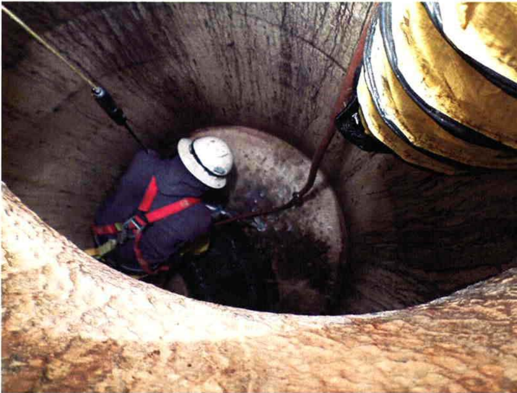
Cushman working at night on March 5, 2014 to break out grout plug in influent manhole, which was installed previously by R. Baker as part of the South Frontage Road Sewer Project in anticipation of this connection to the new WWTF.
