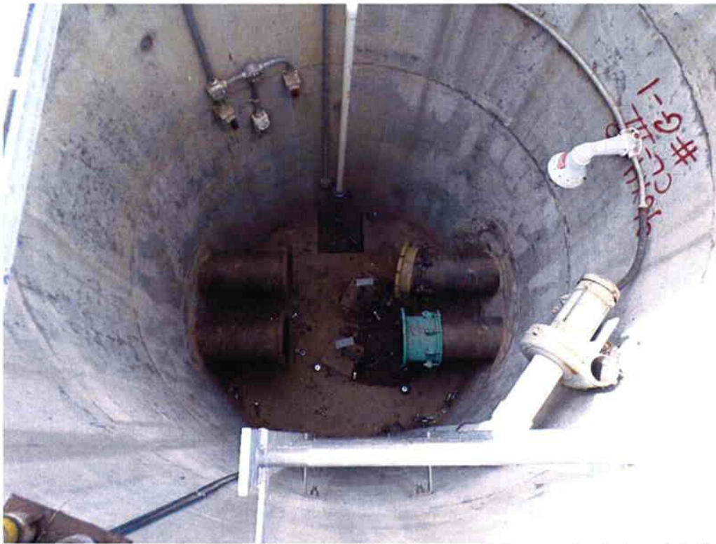
Cushman performing demolition of existing pump station and grinder at influent to old treatment facility.
