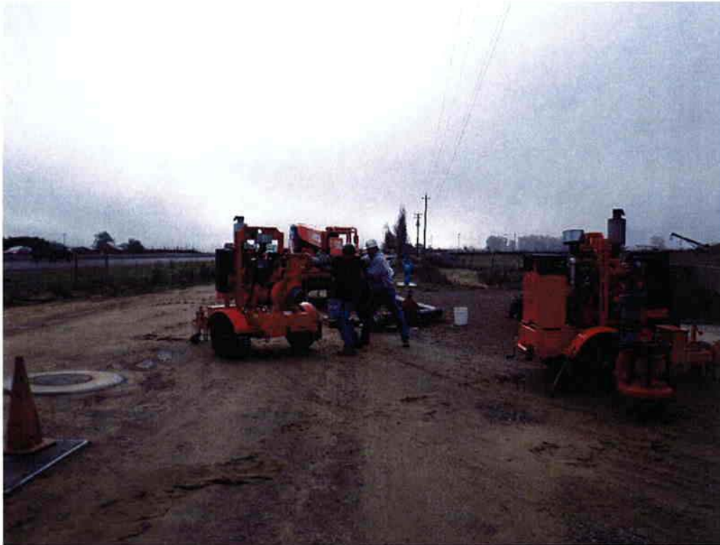
Cushman setting up temporary pumps for the tie-in to the new treatment plant.
