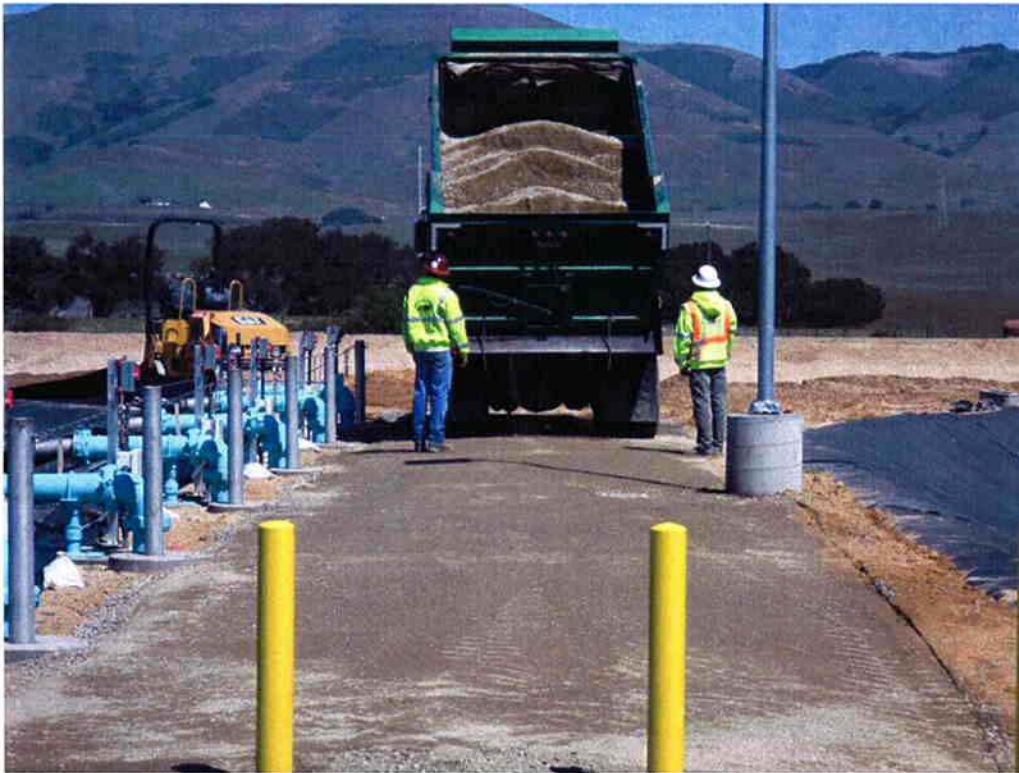
Mark Switzer Excavating placing aggregate base access road between the Aeration Basin and the Emergency Holding Basin.
