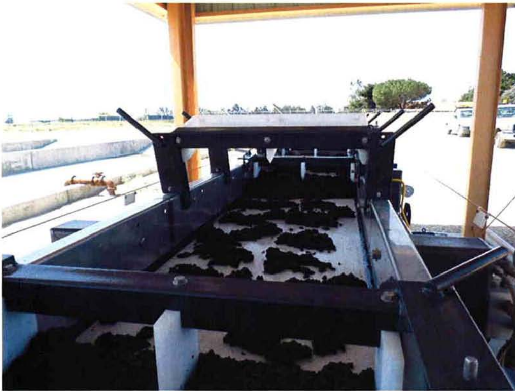
Commissioning and testing the Sludge Thickening System.
