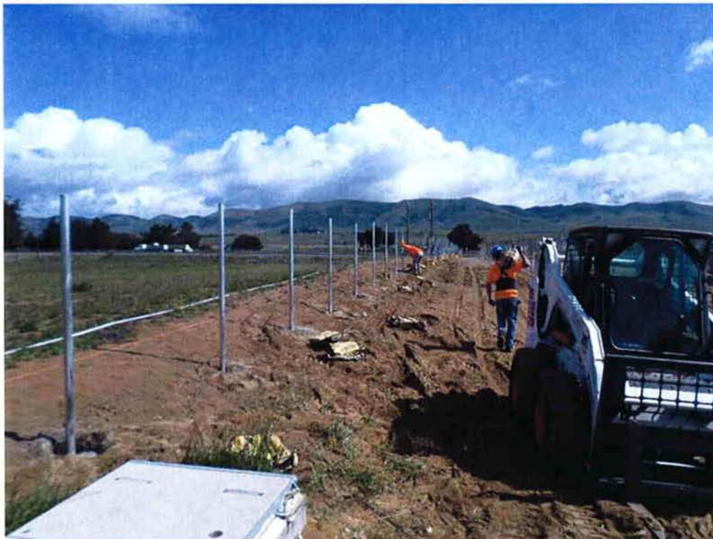
Valley Fence installing new fence on the north border of the site.
