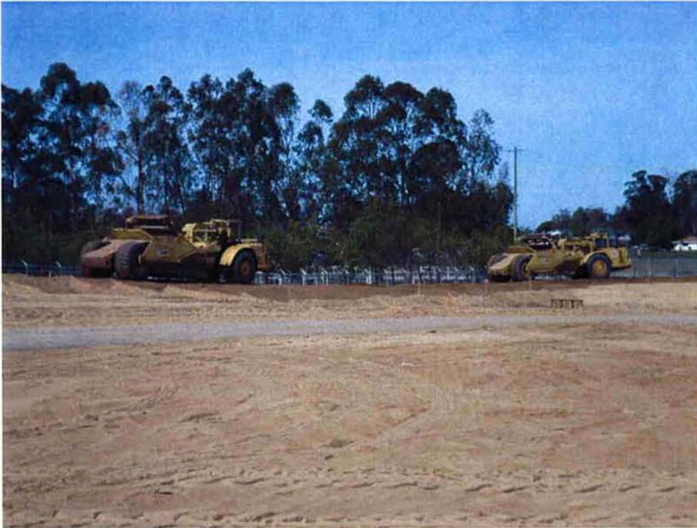
Switzer scrapers using native material from Area F, construction of Ponds 9 & 10, to build up the berm on the west side of the site.
