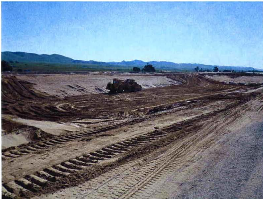
Switzer starting to backfill existing Pond 4 and build berm in the middle to create future Aeration Basin #2.
