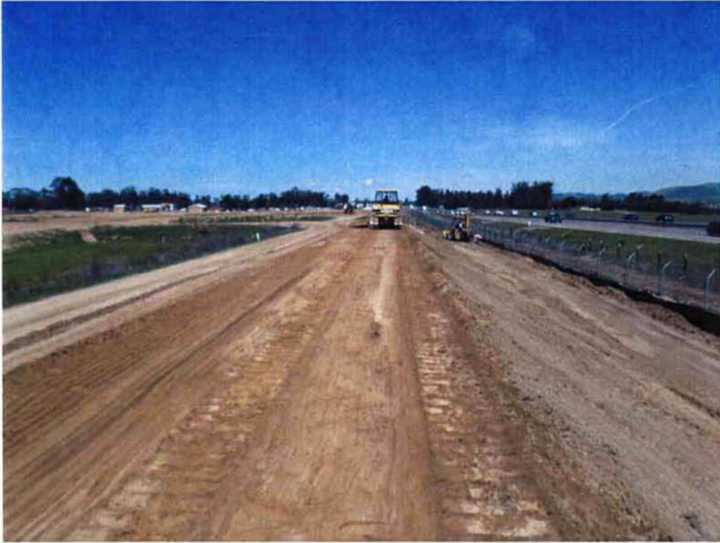
Switzer finish construction of berm on the east side of the site and Hwy 101.
