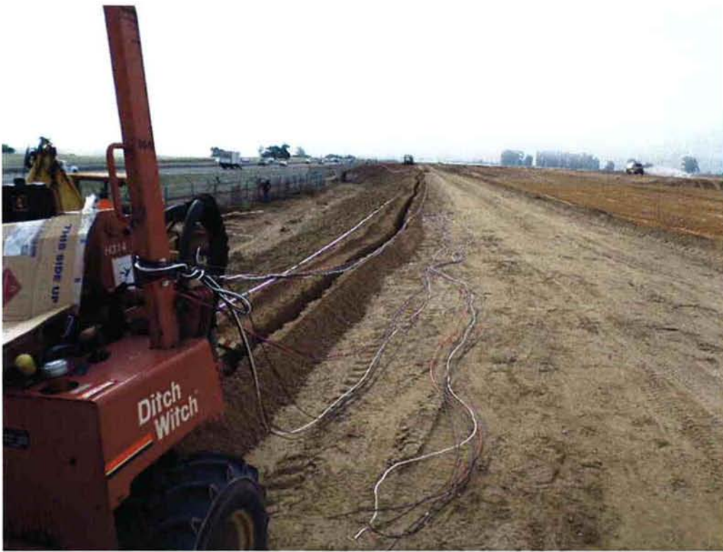
KCI Environmental laying out and installing reclaimed water irrigation lines and power to controllers.
