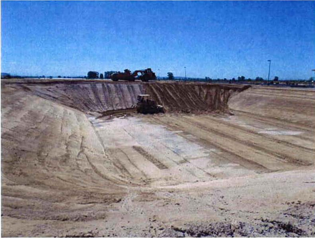
Switzer cleaning up slopes and finishing future Aeration Basin #2, which was constructed from half of existing Pond 4.
