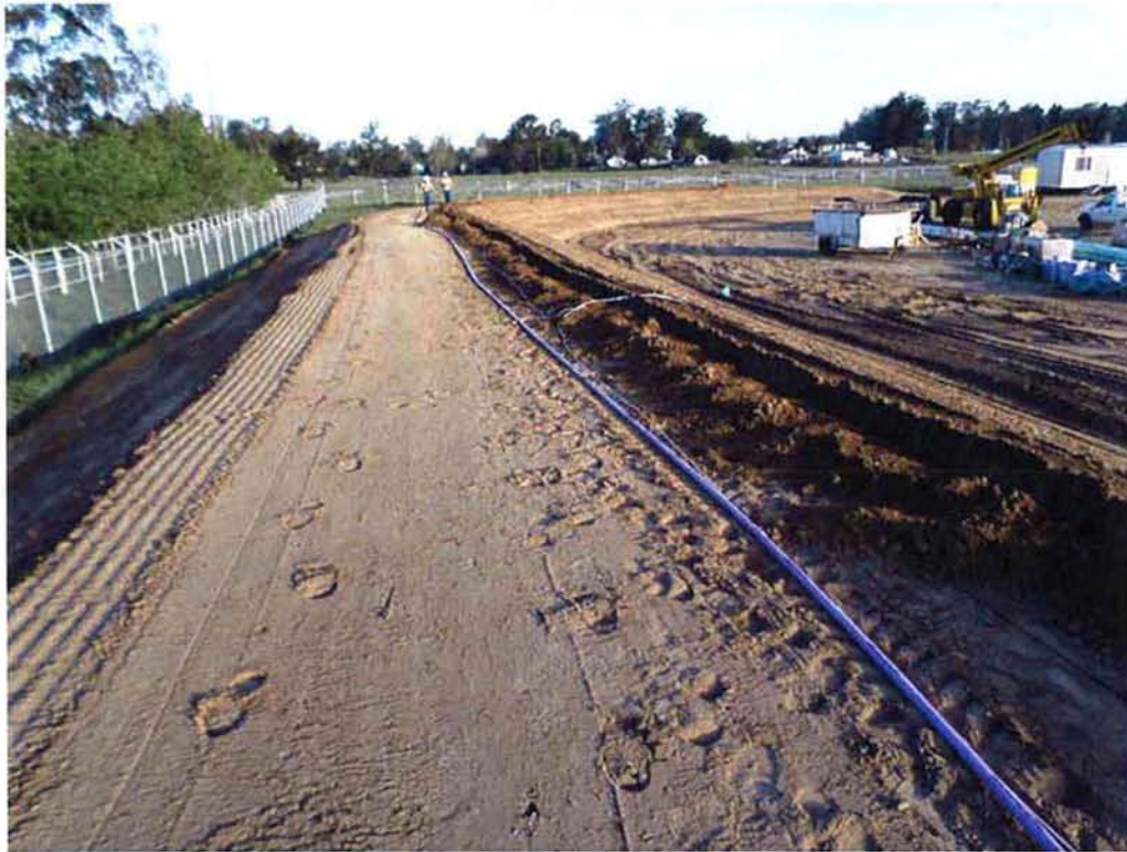
KCI Environmental installing reclaimed water irrigation system on berm to the east of the site.
