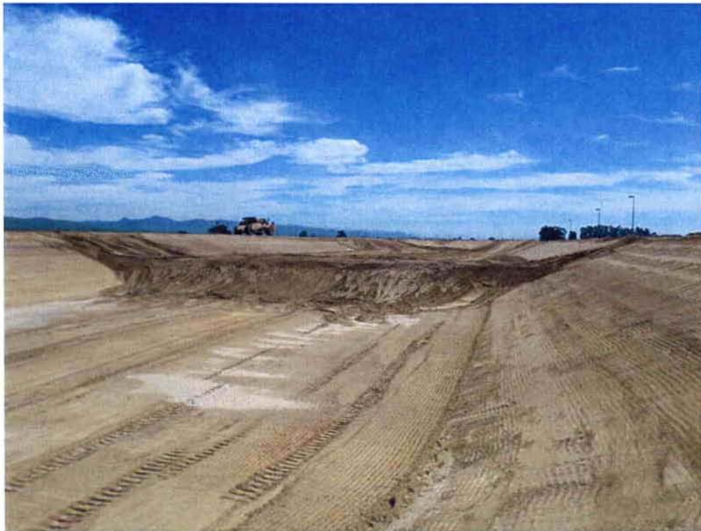
Switzer continuing to fill Pond 4 and build berm for future Aeration Basin #2.
