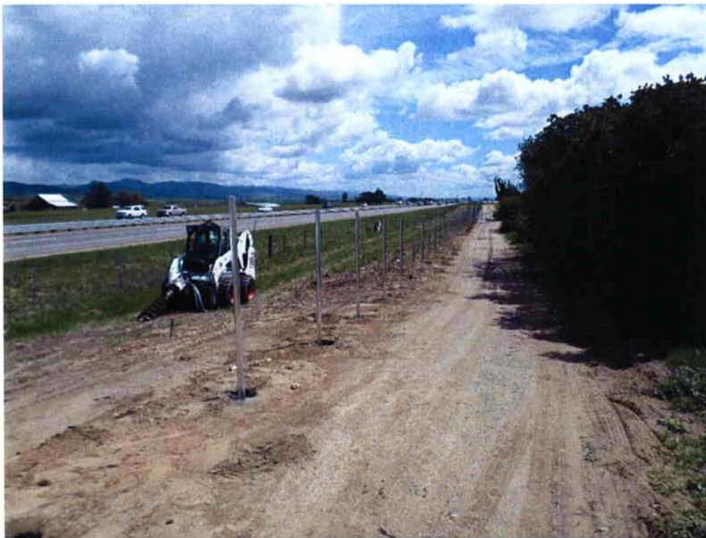
Valley Fence setting posts for the new fence along the east side of the site and Hwy 101.
