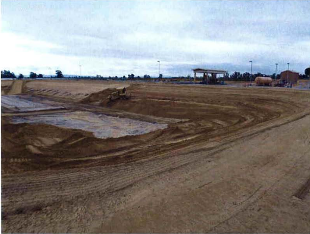
Switzer starting to cut existing banks of Pond 4 to shape it for future Aeration Basin #2.
