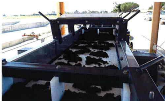
Gravity Belt Thickener in Operation
