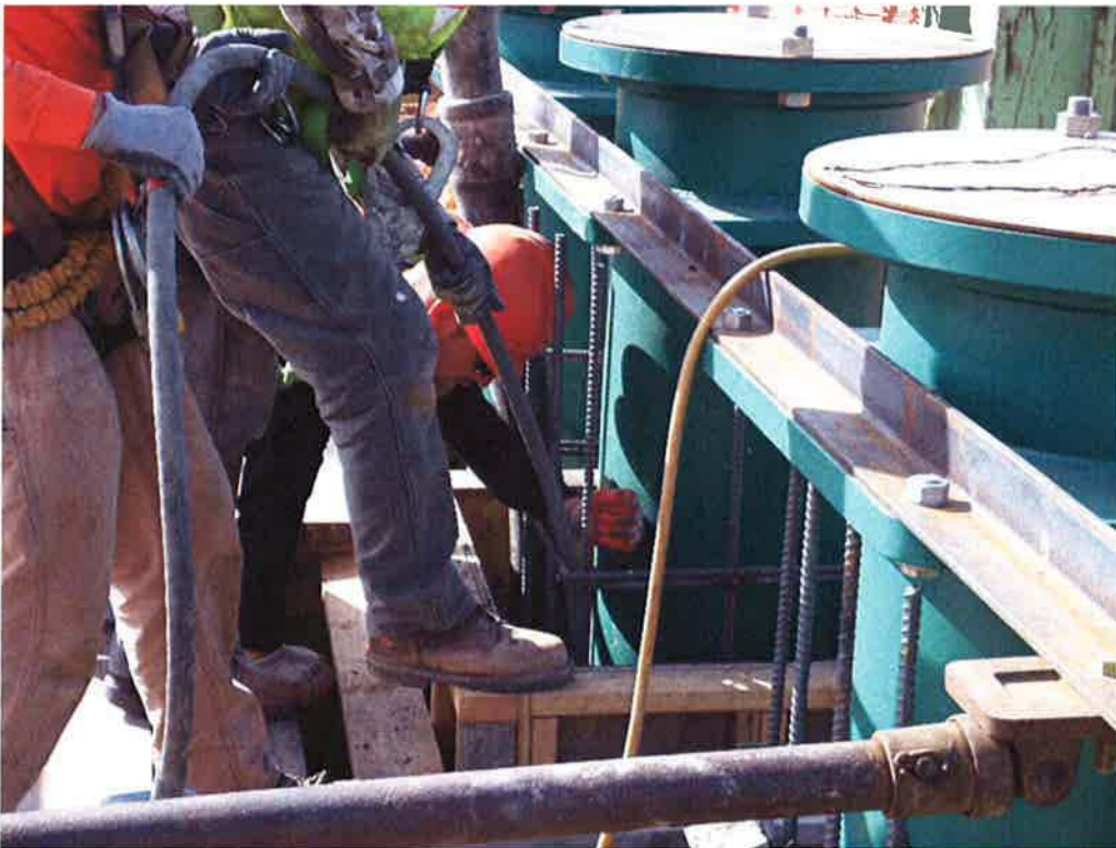
Spiess monitoring and vibrating concrete placement during pour of pump can encasements.
