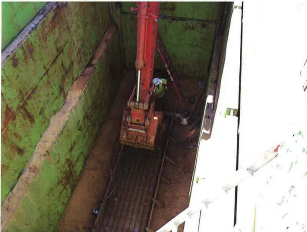
Spies using excavator to place concrete for slab to set pump cans on top of.
