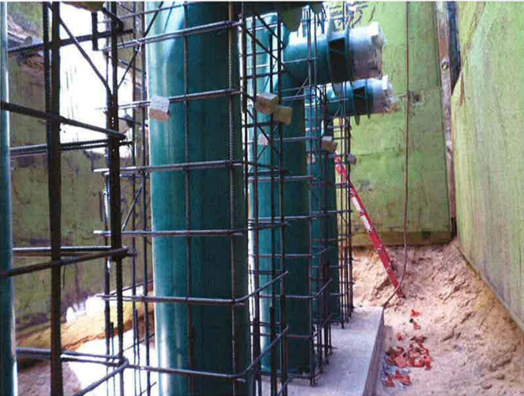
Reinforcing being installed for pump can encasements by Spiess subcontractor Valley Steel.
