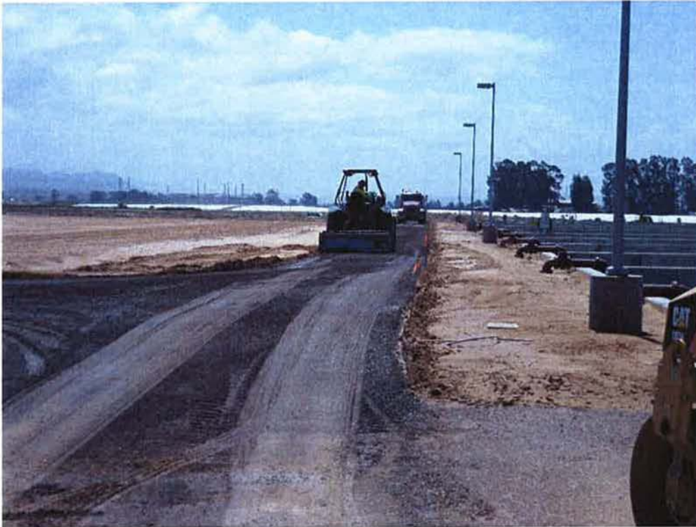
Mark Switzer Excavating completing new site roads with placement of aggregate base.
