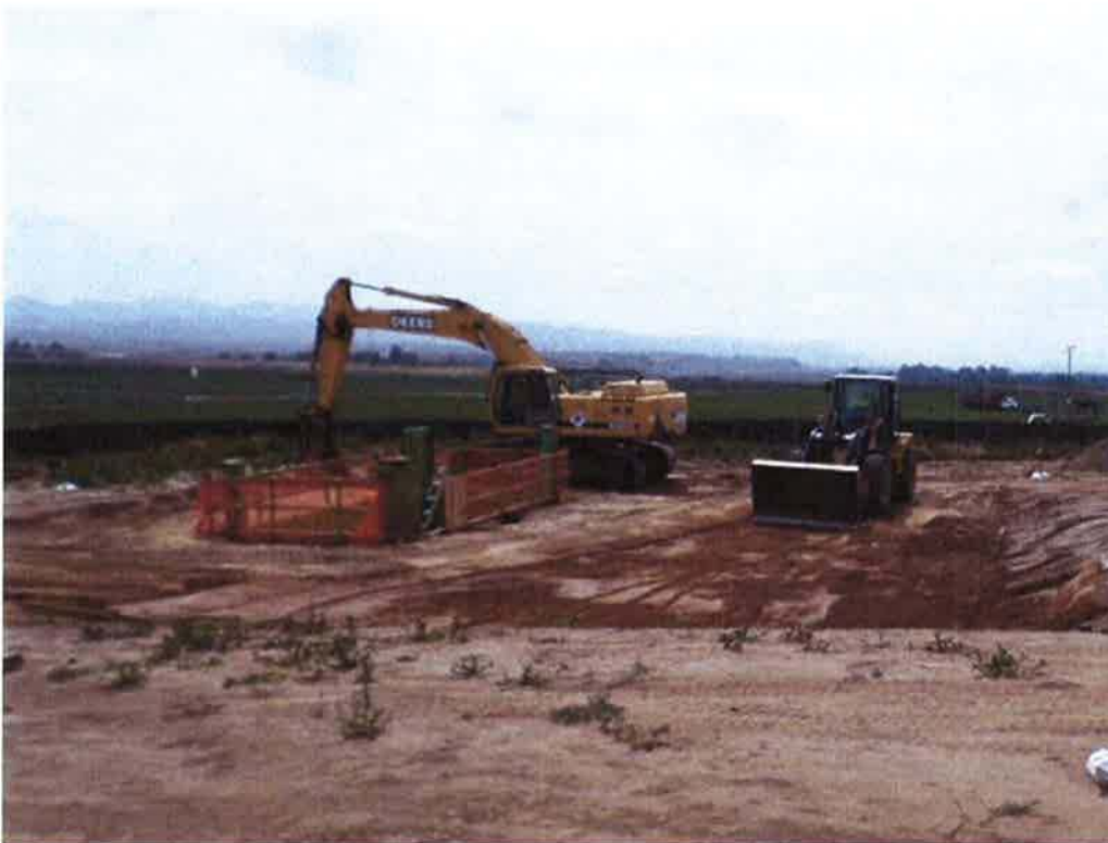
Spiess grading around excavation to prepare for installing supports to stabilize the pump cans when they are set.
