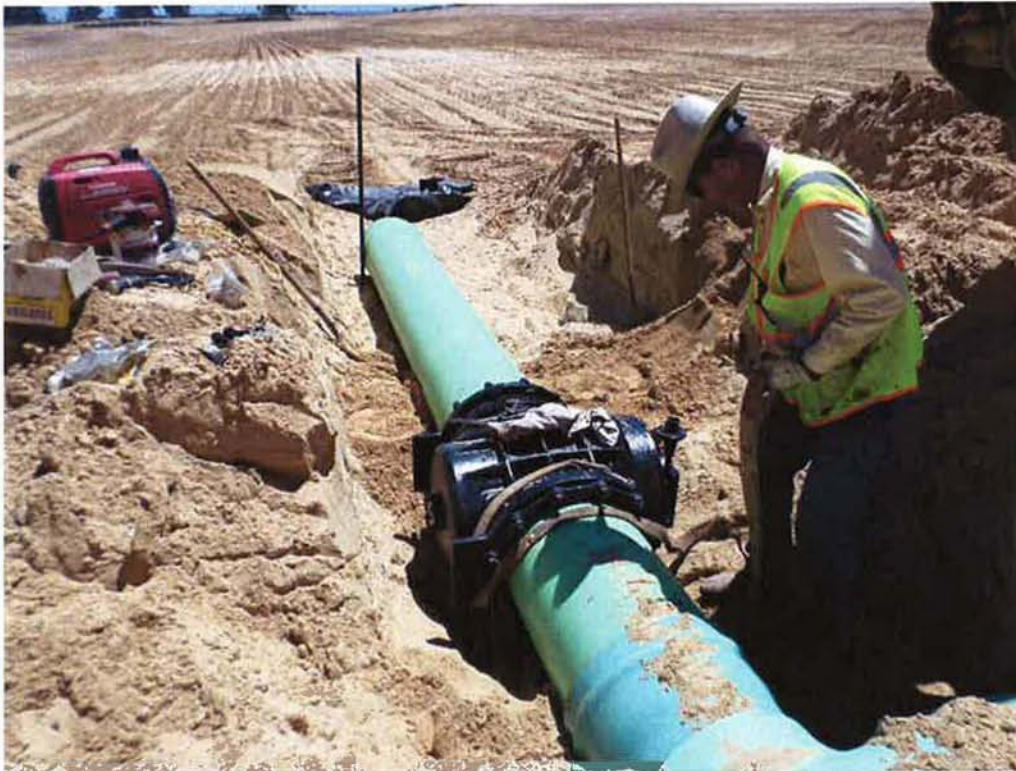
Cushman applying wax tape to bolts on valve of new 18-inch line.
