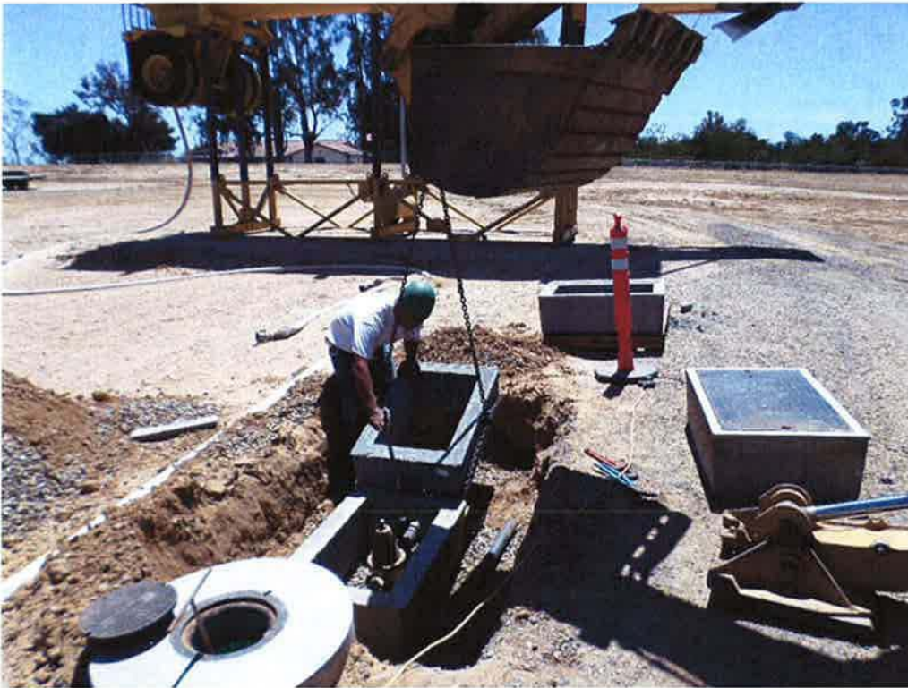
Cushman installing 2-inch meter on the treated water line for the site.
