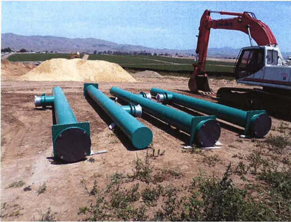
Pump cans delivered to site and coating inspected for thickness and any damage.
