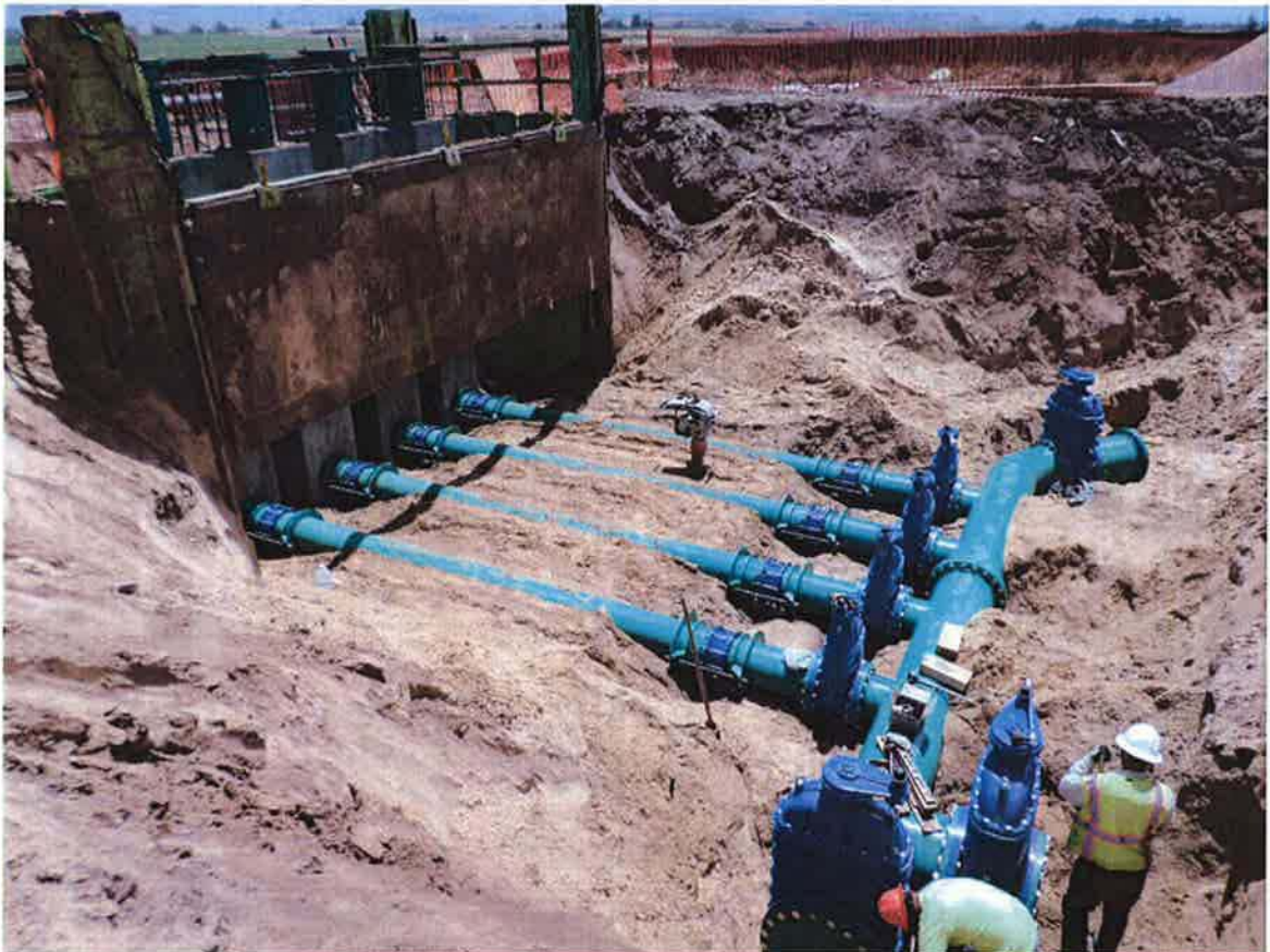
Joshua Road Pump Station Suction Piping June 16, 2014
