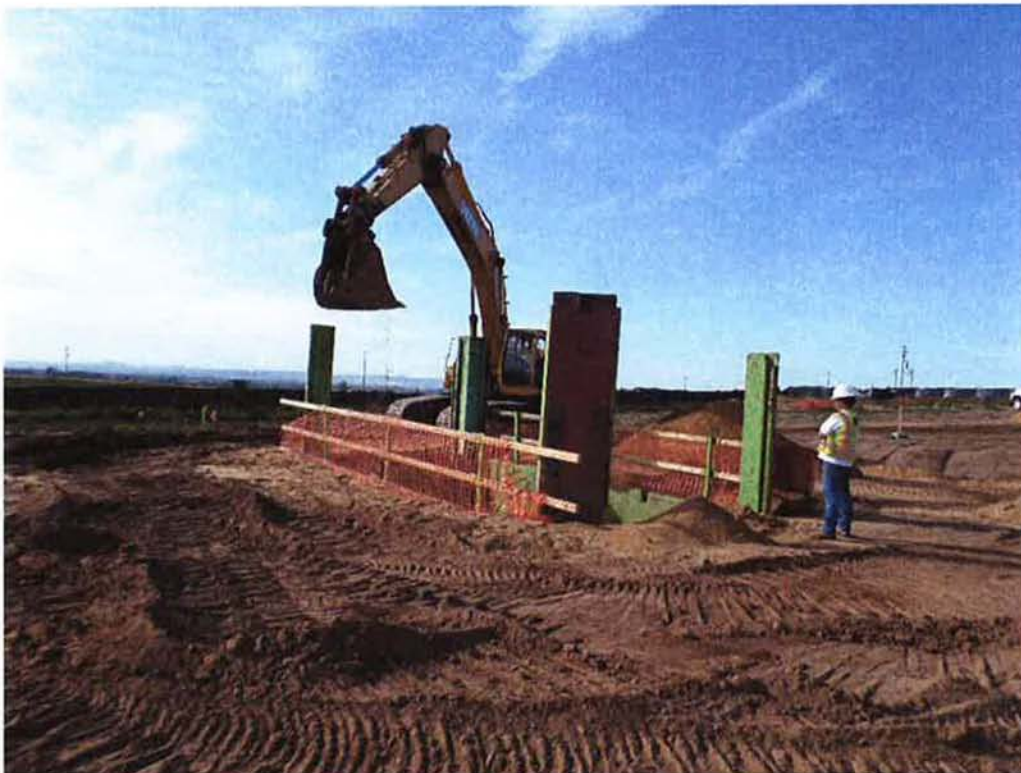
Spiess continuing excavation for pump cans and installing vertical shoring with shoring representative on site from Shoring Tech.
