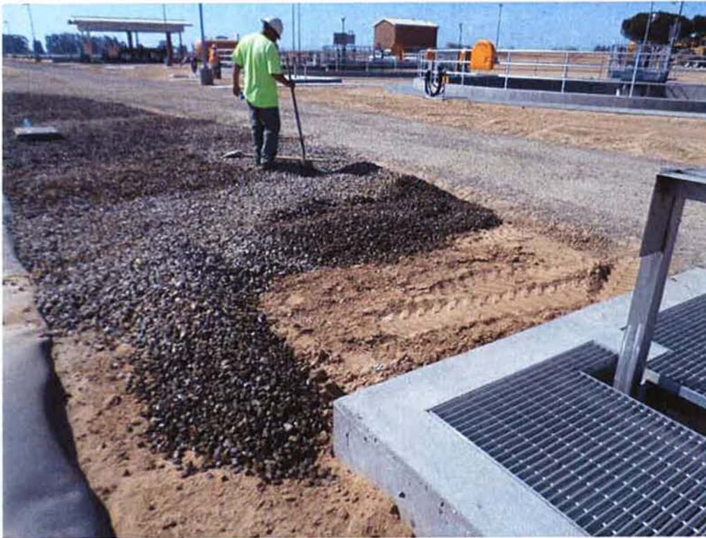
Placing \frac{3}{4} -inch rock around Aeration Basin #1 and the Emergency Holding Basin.
