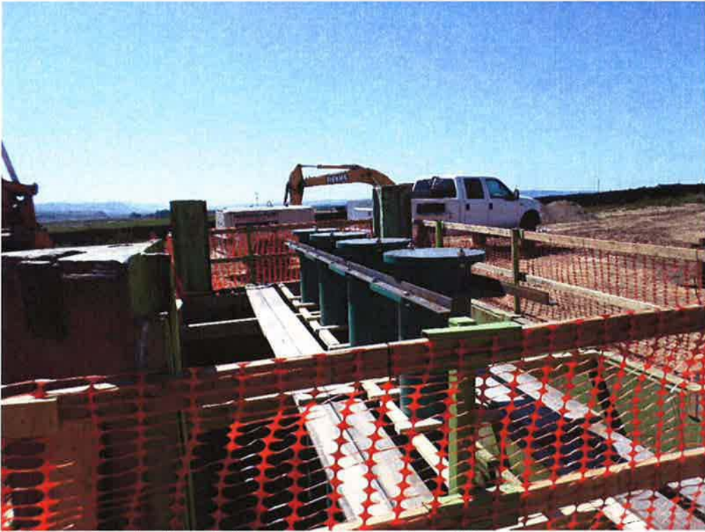
Spiess using steel angle iron to secure spacing of the pump can tops.
