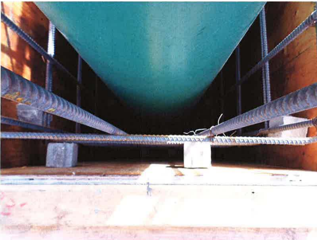
MNS verifying rebar and form spacing prior to Spiess pouring pump can encasements.
