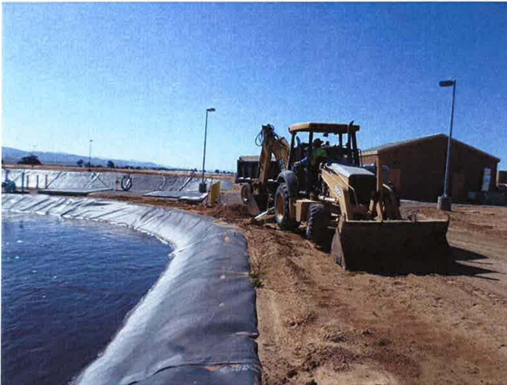
Cushman removing 4-inches of native material around Aeration Basin #1 to place ¾-inch rock.
