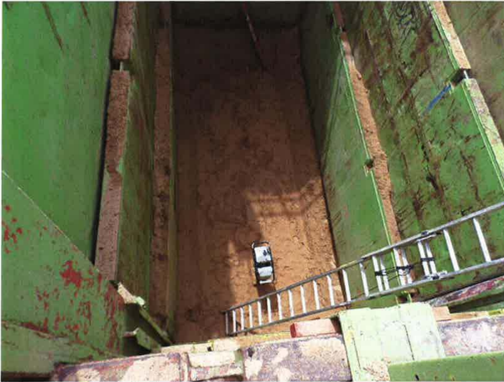
Spiess compacting the bottom of the excavation for the pump cans approximately 23 feet below grade.
