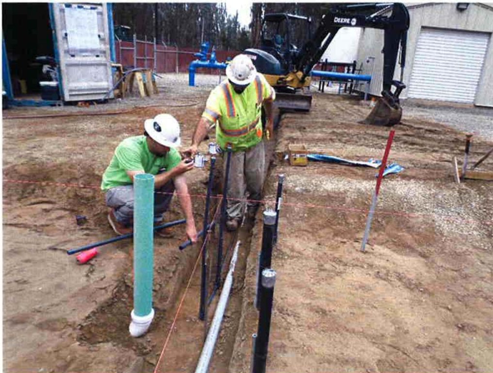
Spieß installing 1/2-inch PVC plant water line and 2-inch PVC chemical tubing line.
