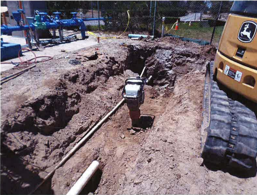
Spieß relocating existing 1-1/2-inch Irrigation line and 4-inch drain line which interfere with the future structures.
