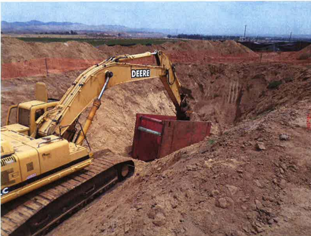
Spiess setting shoring for installing 24-inch DIP for future connection to the HDPE pipe installed as part of Bid Package #1.
