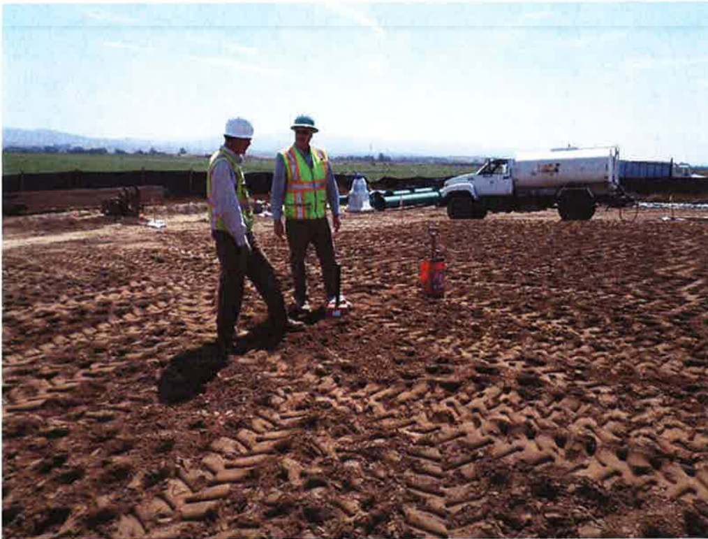
Fugro on site to test compaction of backfill at future pump station.
