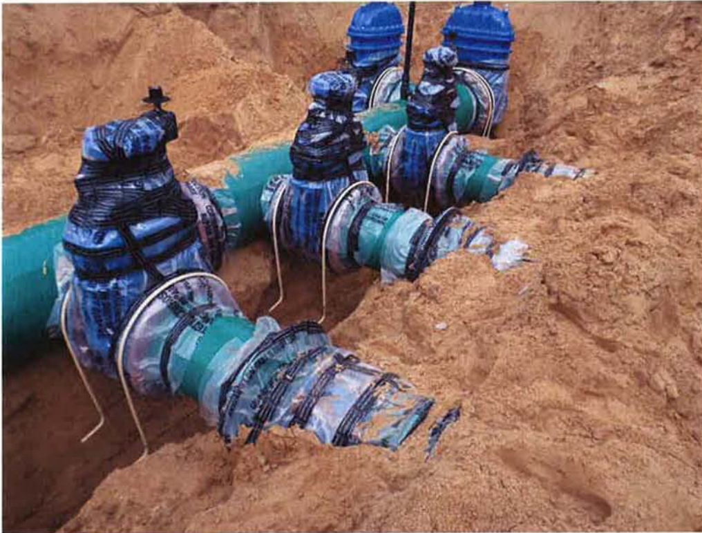
Spieess excavating for concrete blocks and placing epoxy rebar anchors over valves on inlet piping.
