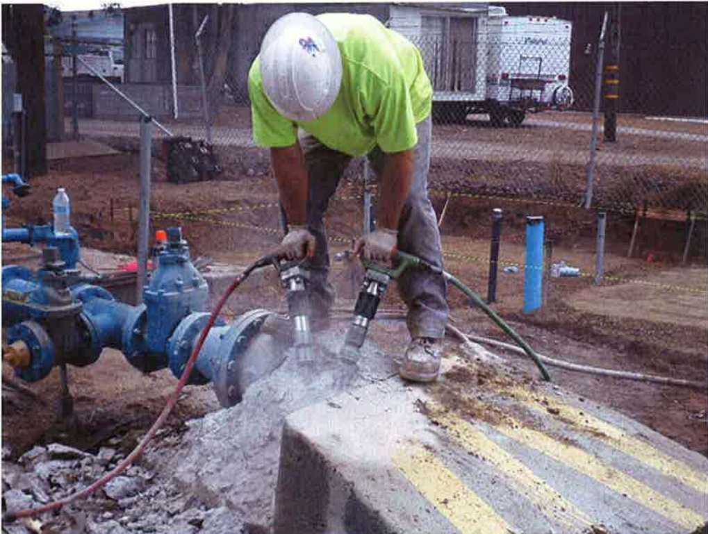
Spiess performing demolition of existing thrust block for installation of pipe riser.
