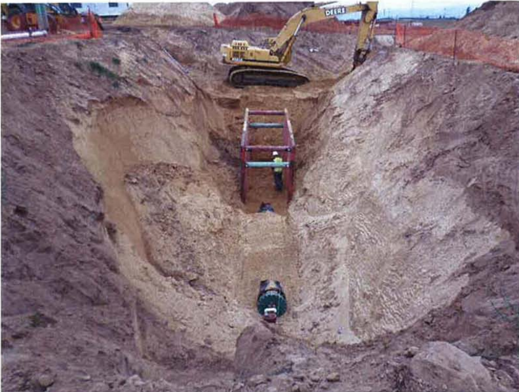
Spies continuing installation of 24-inch DIP from the future connection point at the HDPE pipe to the pump station inlet manifold.
