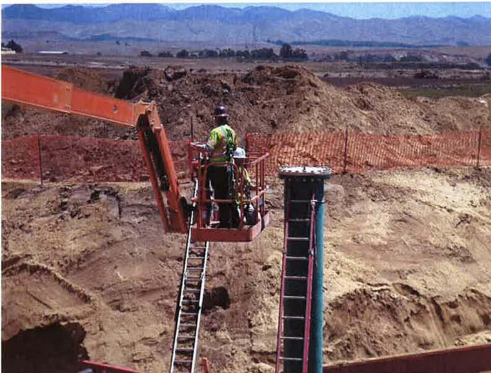
Spiess tightening bolts at the top of the pig launcher riser during pressure testing.
