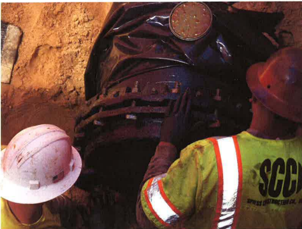
Spiess applying wax tape to bolted connection on the DIP pipe for the future tank outlet.
