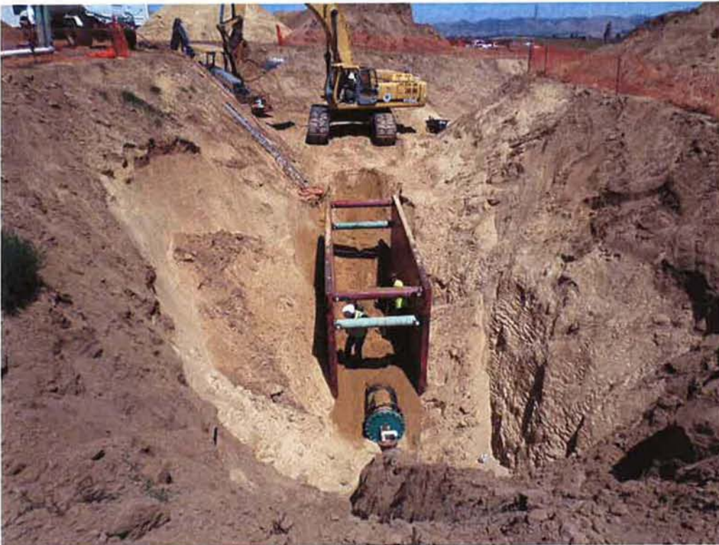
End of 24-inch DIP which will be connected to the HDPE in the future.
