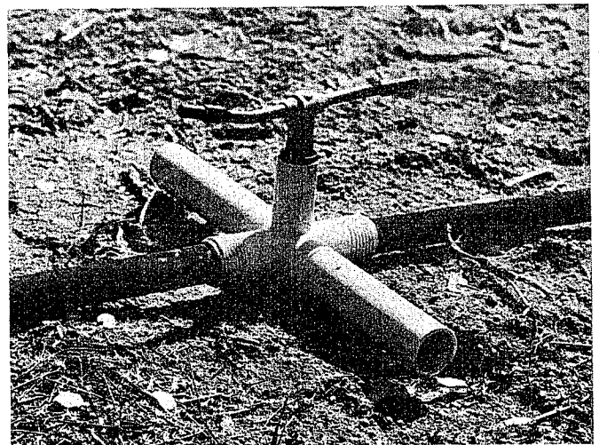
An under-tree sprinkler.
