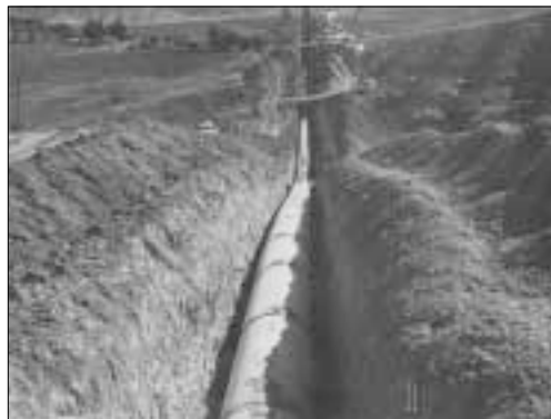
Construction of the South Coast Conduit Channel which runs from Tecolote Tunnel to Carpinteria
