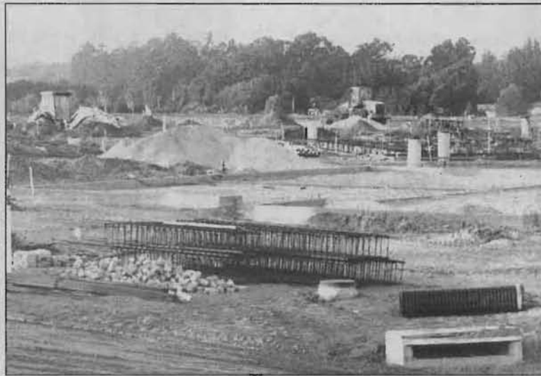
CONSTRUCTION WOES — New construction development is on its way to Nipomo, but the task force wades through five reports and a
