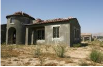
Empty houses under construction line Maria Vista Estates near Nipomo. Bankruptcy filings cloud the future of the development. / TPR/Bryan Walton
