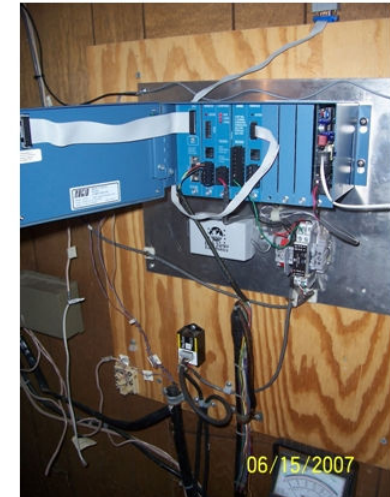
Water Level, Gates, & Evap. Pan Data Interface to SB City (RUG9/SCADA)
