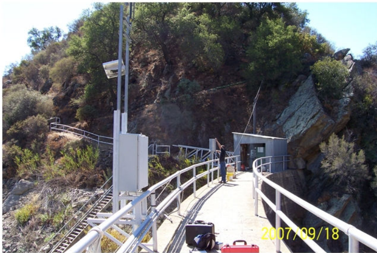
Water Level & Rain ALERT Instrumentation
