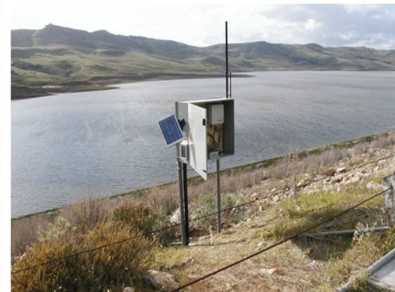
Reservoir & Level Instrumentation (Bubbler)
