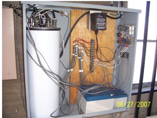
Reservoir Level & Gate Opening ALERT Instrumentation
