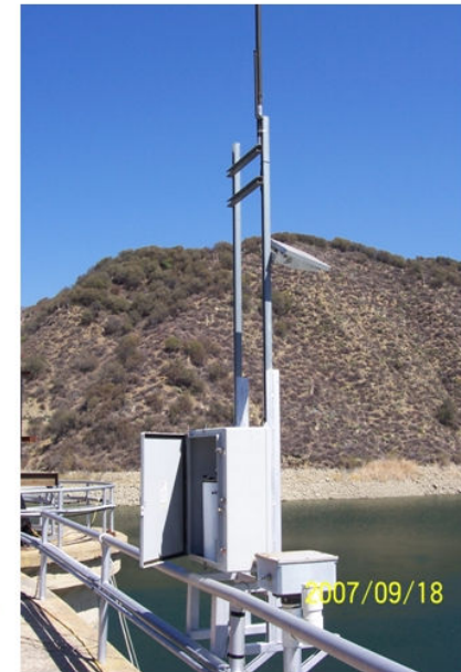
Water Level ALERT Instrumentation (Press. Trans.)
