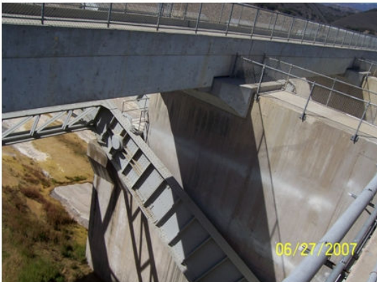
Dam Gates & Inclinometers
