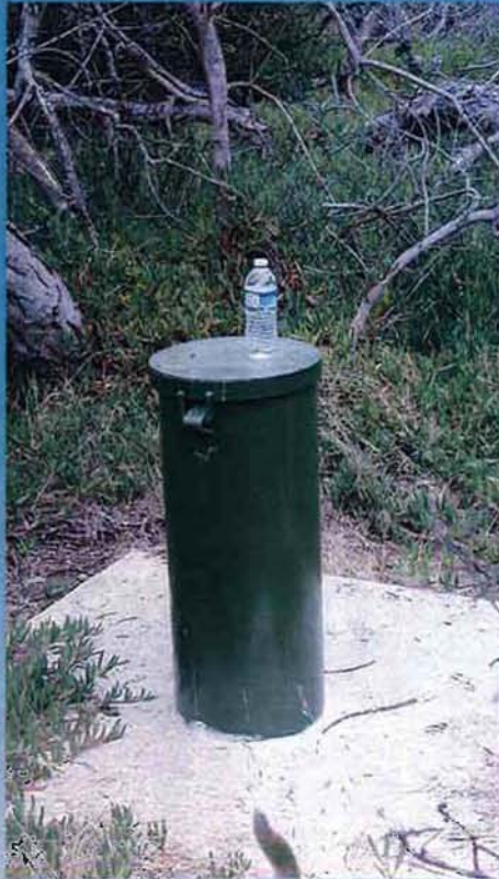
Pier Avenue Sentry Well 1/2 Mile Inland
