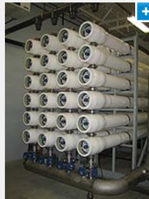
The plant has a single-rack RO skid design with four separate columns of pressure vessels.
