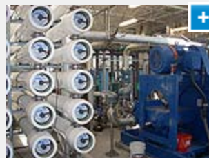
Internal RO equipment, pumps and piping within the
