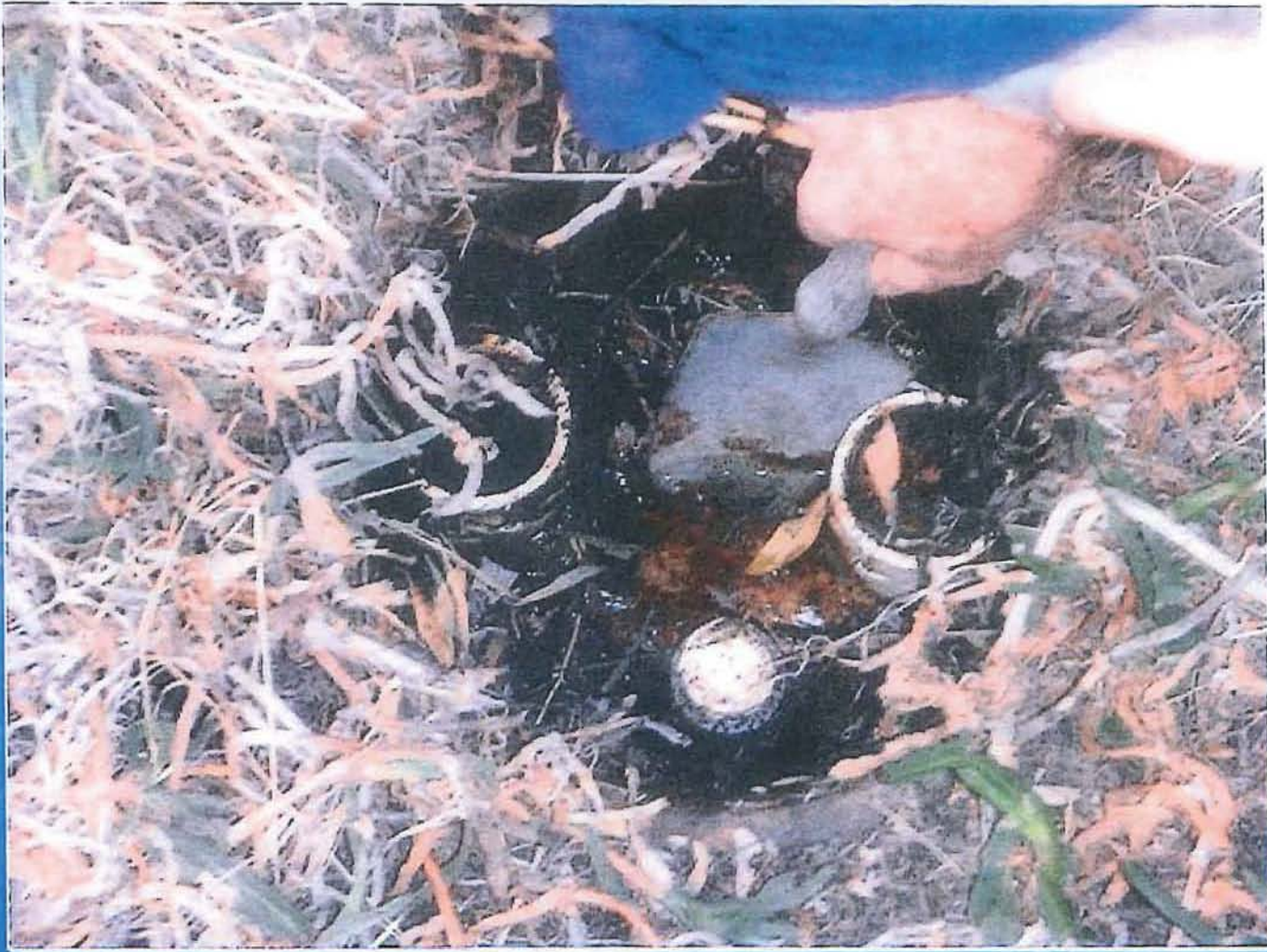
Well in Great Disrepair. Note High Level of Contamination.
